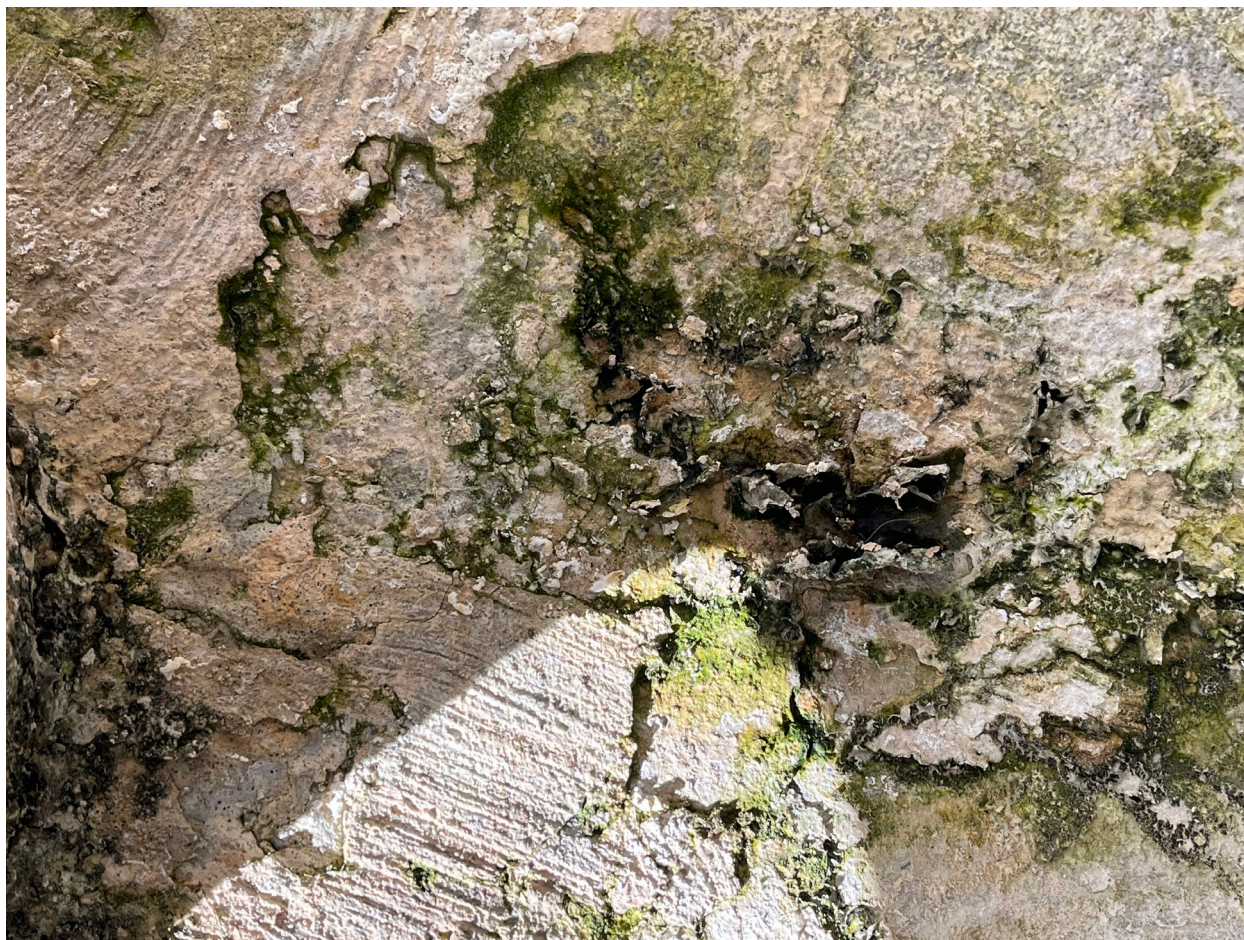
View of the concrete degradation and algae growth along the SBR sidewall. (IMG_0327). 03/27/2025 11:37 AM Photographed by D. Esparza
