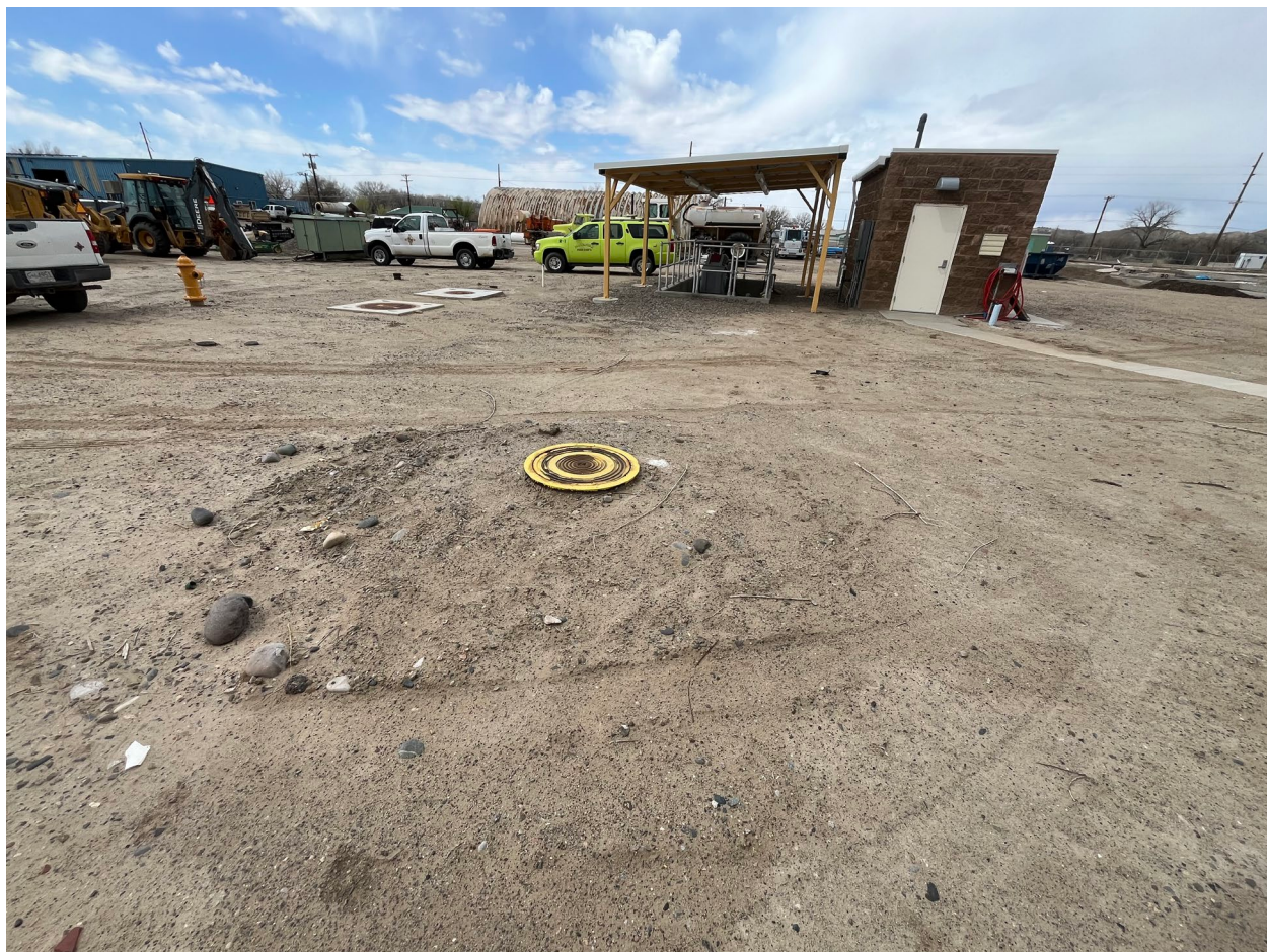
View of sodium bisulfite injection manway. Note: the visible vehicle tire marks around the manway and lack of structure protection, i.e., bollards. (IMG_0318) 03/27/2025 11:32 AM Photographed by D. Esparza
