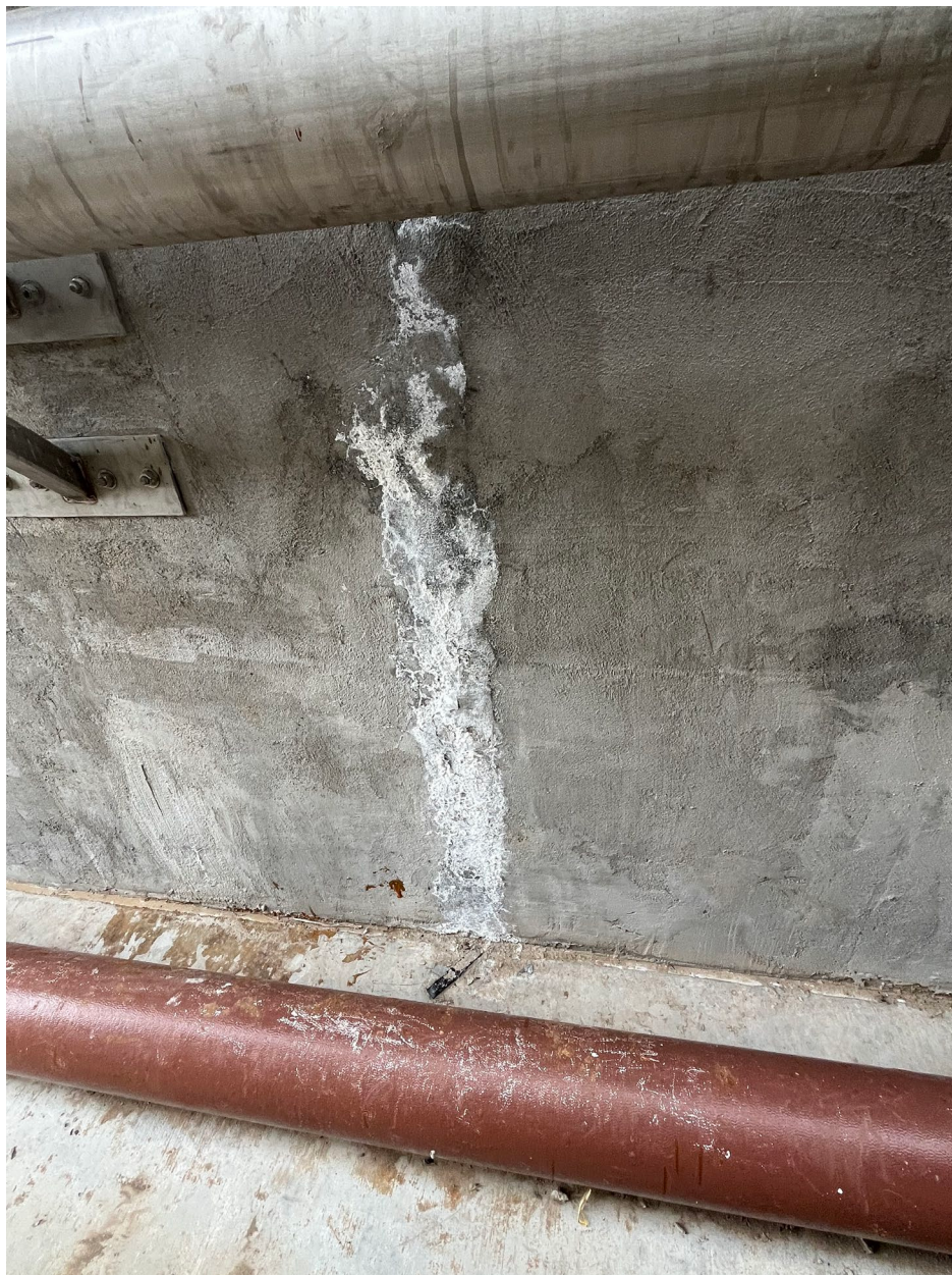
Another view of leaking along the new SBR basins approximately at land surface. (IMG_0312). 03/27/2025 11:23 AM Photographed by D. Esparza
