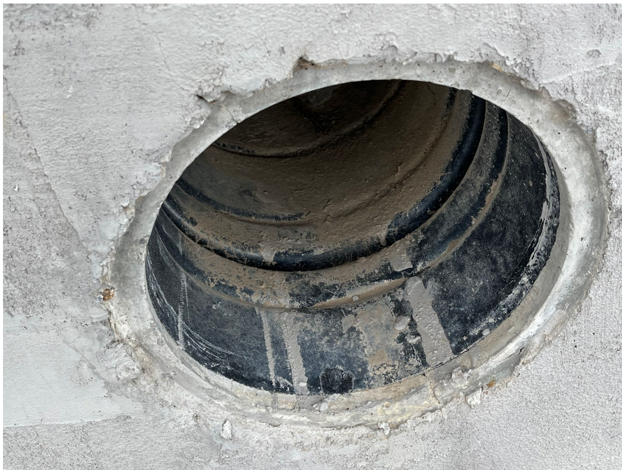
Close-up view of a sidewall penetration. Note: the cracking and spalling of the concrete around penetration. (IMG_0317). 03/27/2025 11:26 AM Photographed by D. Esparza
