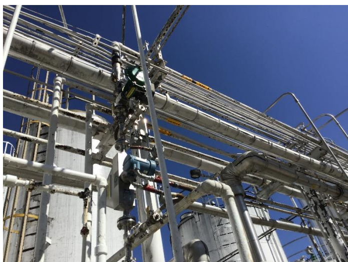
Photo 4: Overhead piping connected to tanks in tank farm, including hazardous waste tank T-81.
