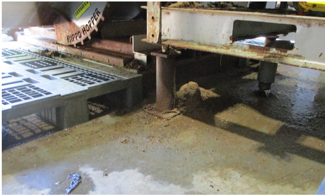
Photo 13: Sludge accumulating on floor outside of dumpster in Building 3.
