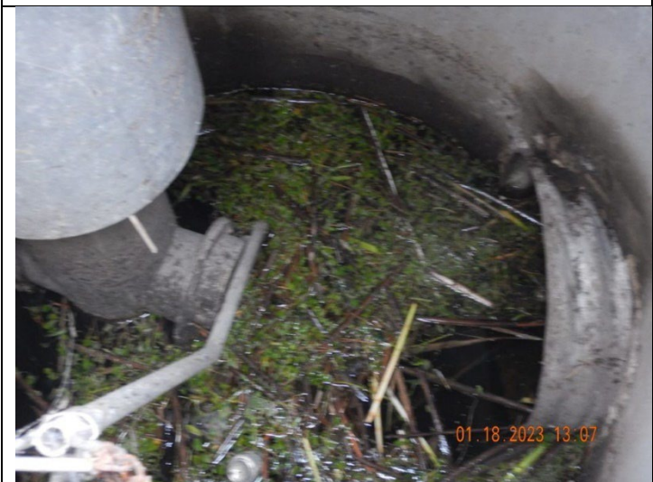
Photo: #41 (DSCN0498.JPG) Description: Interior view of a Type 2 catch basin situated between stormwater pond and drainage district lateral. Facility representatives referred to this as a stand pipe assembly; waters flow from pond through pipe (right) and would flow up through metal assembly (left) before discharging. Representatives stated they would sample here in the event the basin filled.
