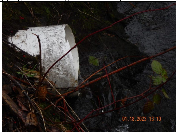
Photo: #42 (DSCN0499.JPG) Description: Image of pipe with water discharging into Drainage District 5 lateral. This outfall sat directly between Facility's stormwater pond and the lateral. Pipe appeared made from PVC or a similar material.
