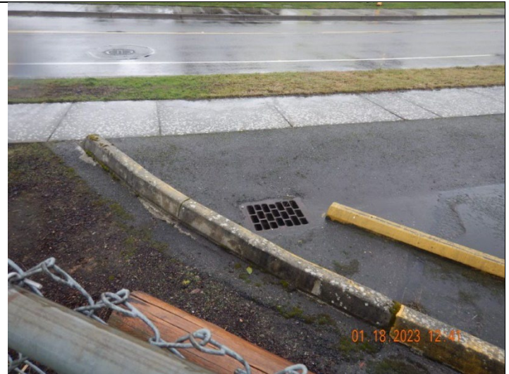
Photo: #20 (DSC0477.JPG) Description: Facing south, catch basin next to Battersby Avenue, located on neighboring property, did not appear to receive stormwater flow.
