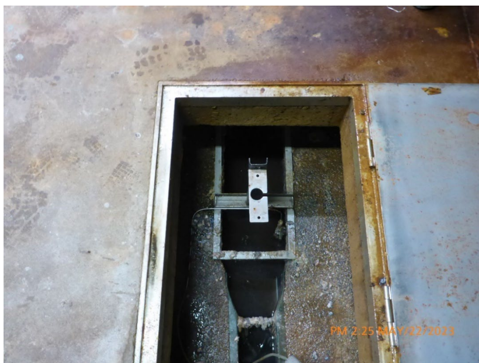
Photograph 4. The flow measurement pit identified in the permit as the designated sample point at Kunzler.
