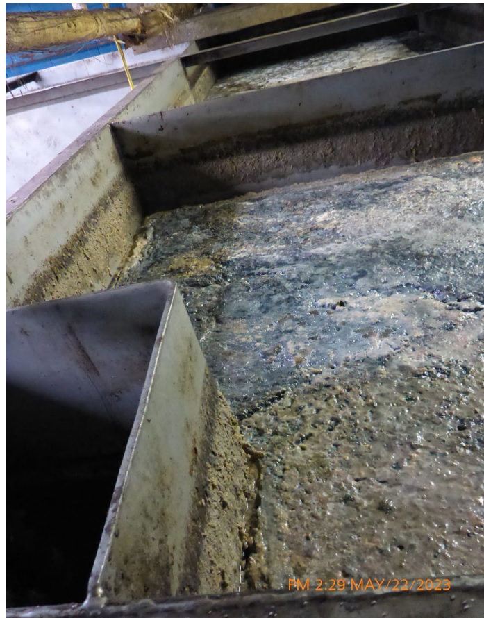
Photograph 2. View of floatable O&G on top of the holding tanks at Kunzler.
