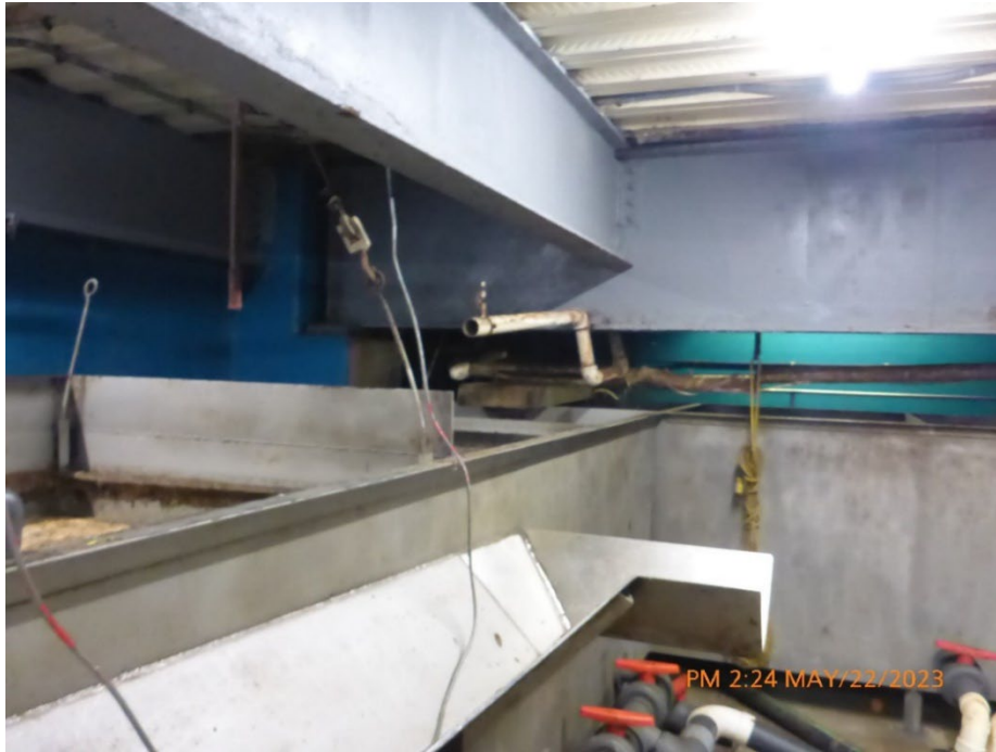
Photograph 1. View of the holding tanks in the treatment area at Kunzler.
