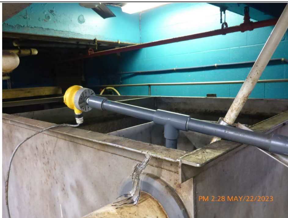
Photograph 3. View of the holding tank where the facility is measuring pH at Kunzler.
