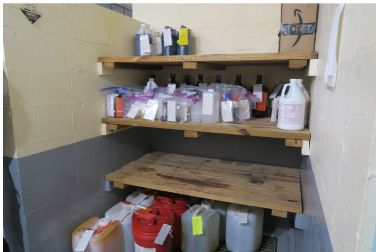
Photo 11: Waste containers on the wooden shelves in the TSD Building, shelf labeled with corrosive hazard indicator for acid waste storage.
