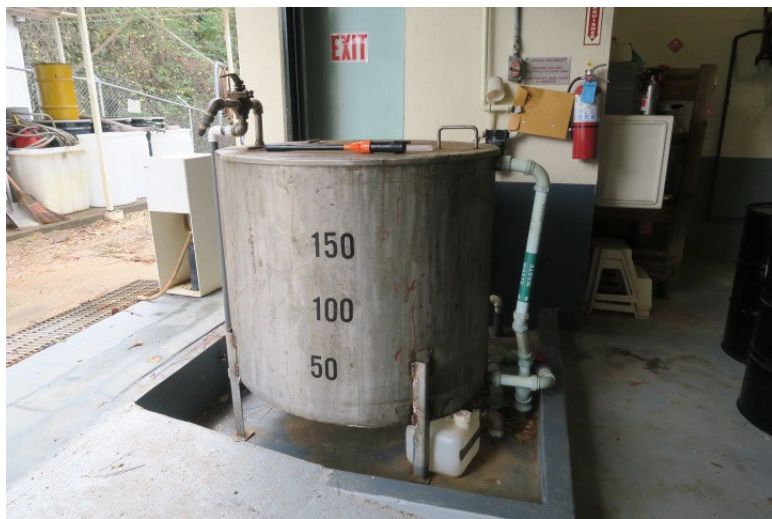
Photo 5: Neutralization tank in the TSD building.
