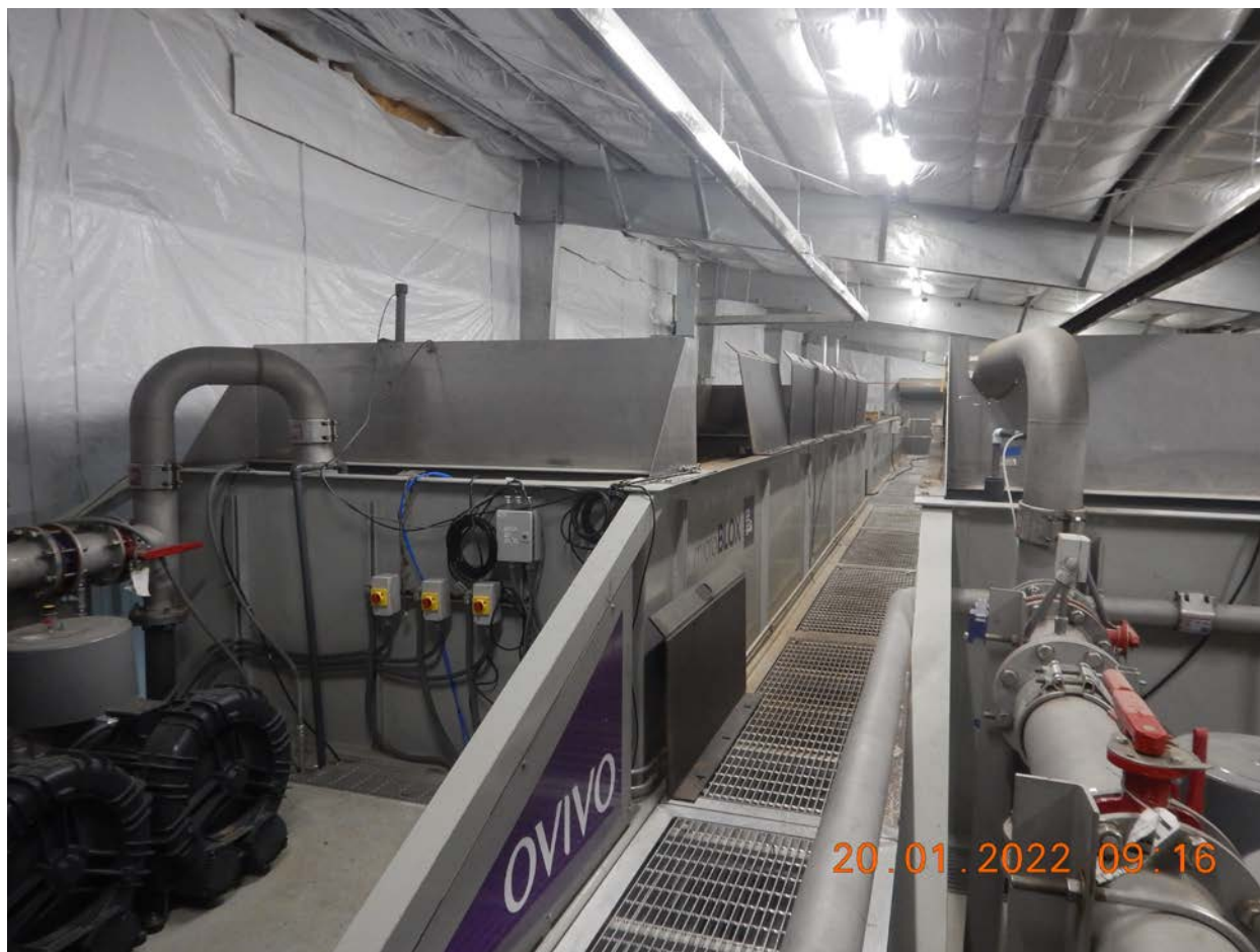
A view of a portion of the Ovivo Membrane Bioreactor (MBR) system. (DSCN2114). Photographed by D. Esparza
