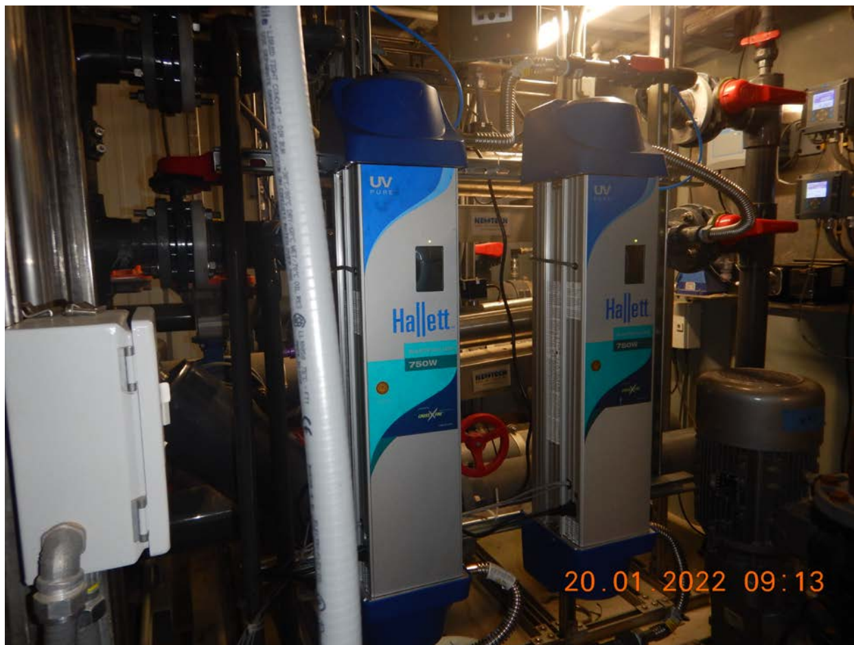
View of the upgraded UV disinfection system in conjunction with the Ovivo Membrane Bioreactor (MBR) system. (DSCN2113). Photographed by D. Esparza
