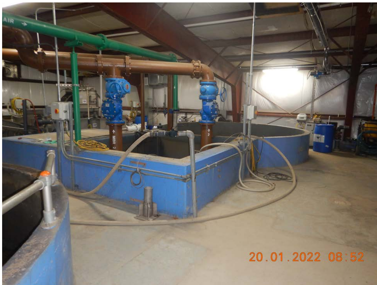
Another view of the in-ground equalization (EQ) basins. (DSCN2109). Photographed by D. Esparza
