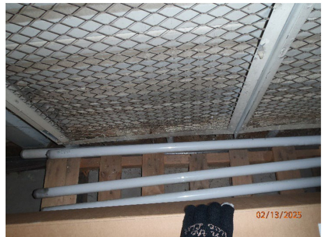
Picture 12 – Building 72 Universal Waste lamps uncontained, not dated, not labeled
