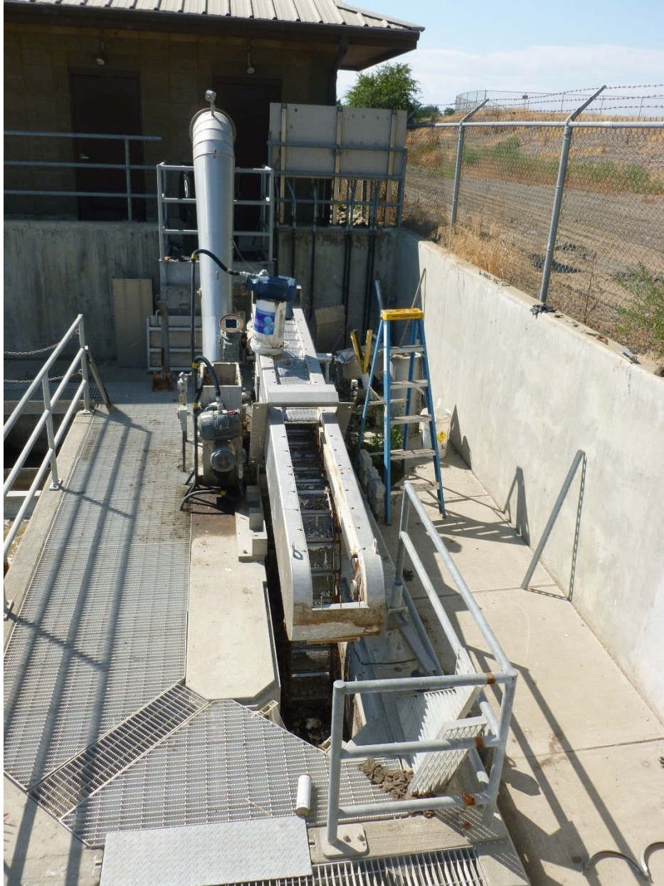
Photo 1 / P1010448 – Influent Screen, inoperable
