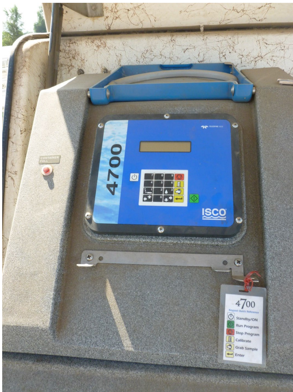
Photo 5 / P1010463 – Auto-Sampler, control panel
