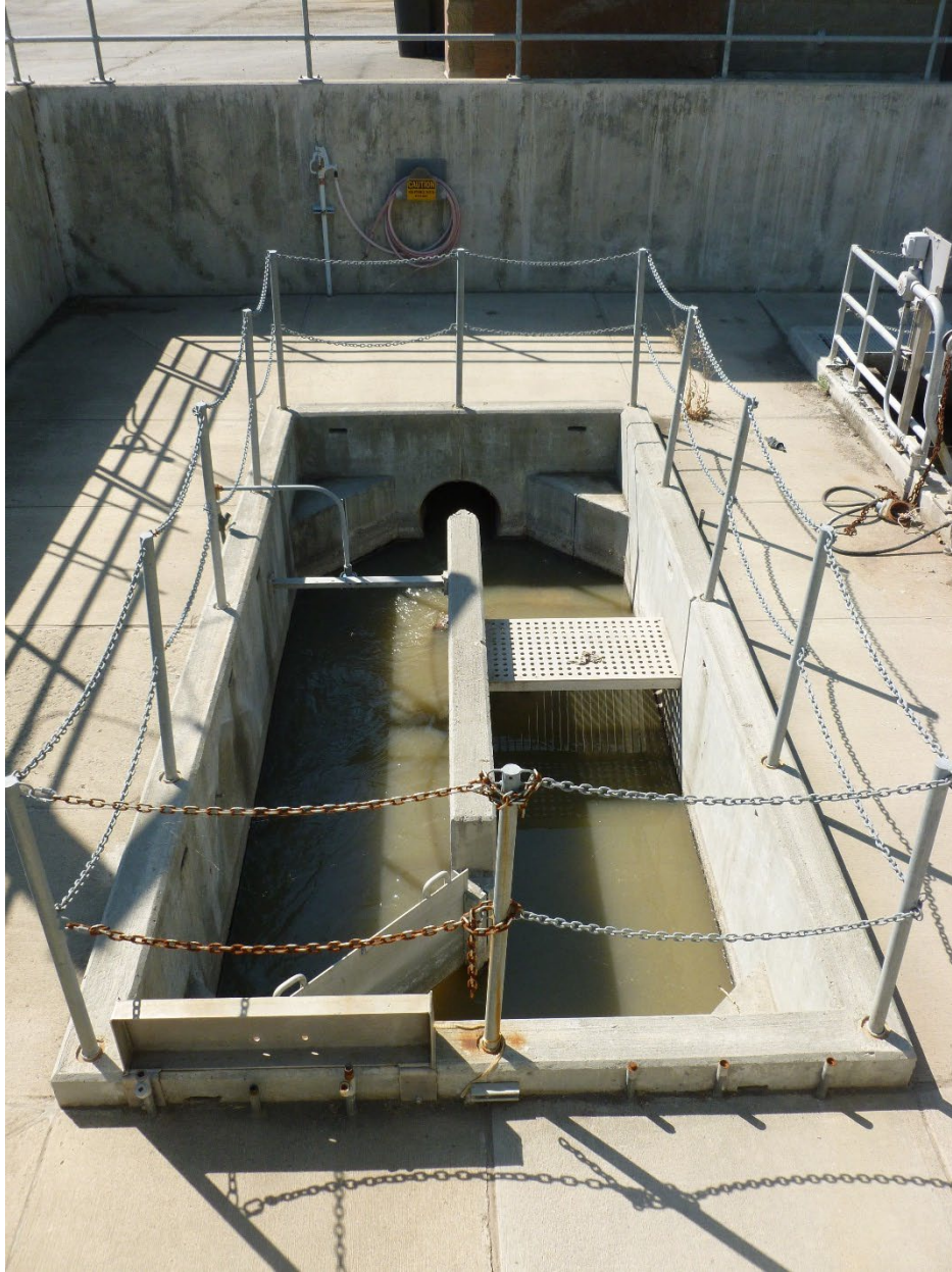
Photo 2 / P1010451 – Secondary Bar Screen
