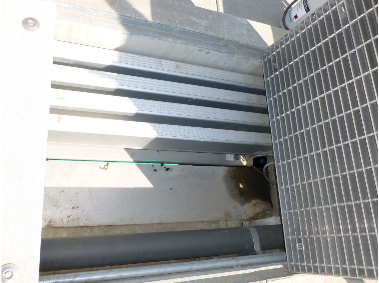
Photo 4 / P1010461 – UV Bank, interior
