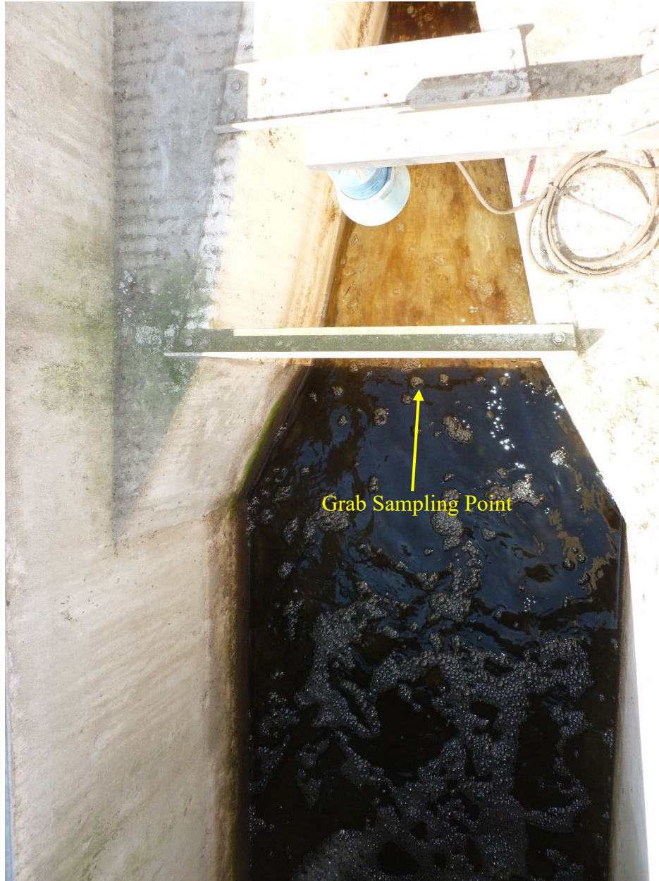
Photo 8 / P1010466 – Parshall Flume, grab sample location
