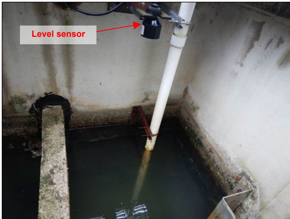
Photograph 32. Bayard WWTP. (DSCN9706) View of the level sensor in the chlorine contact chamber used to determine effluent flow rate.
