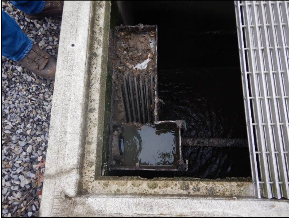
Photograph 43. Elk Garden WWTP. (DSCN9972) View of the influent bar screen in the first chamber of the flow equalization basin.
