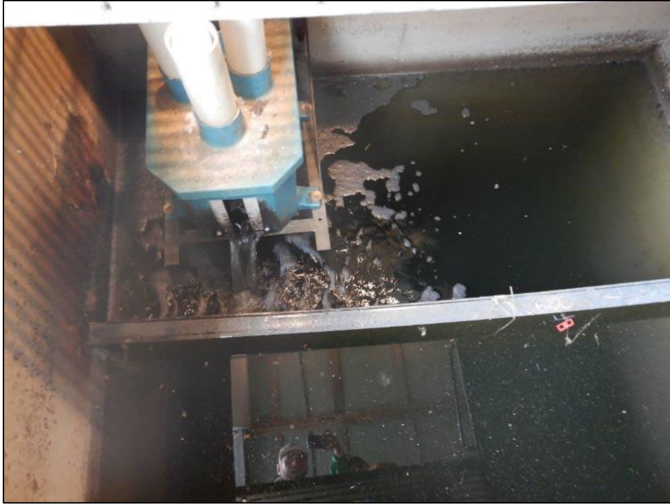
Photograph 59. Elk Garden WWTP. (DSCN0012) View of the chlorination unit and chlorine contact chamber. Floating debris was observed on the surface of the chlorine contact chamber.
