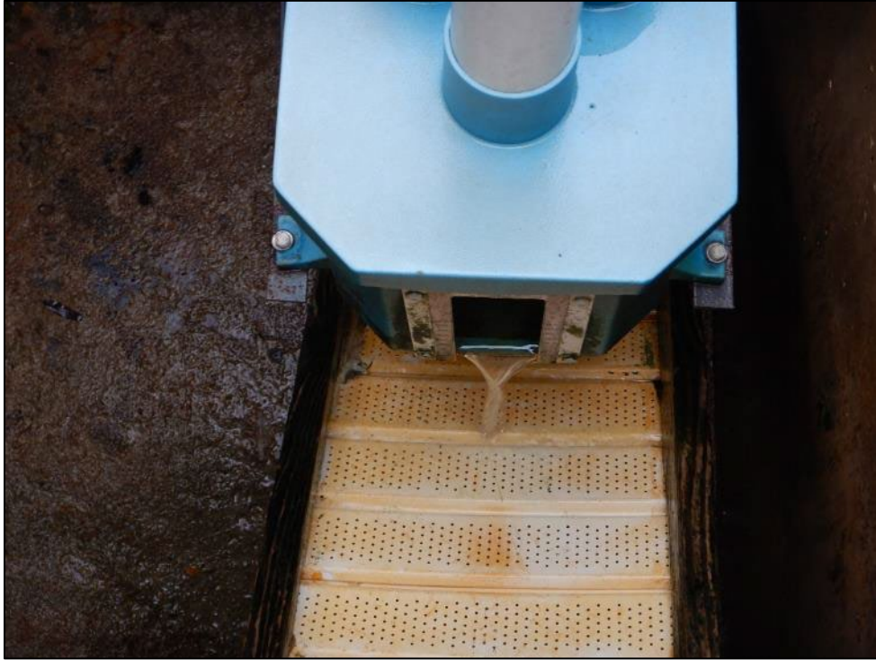
Photograph 35. Bayard WWTP. (DSCN9710) Close-up view of effluent flow out of the dechlorination unit. Effluent flows from this chamber to Outlet 001.
