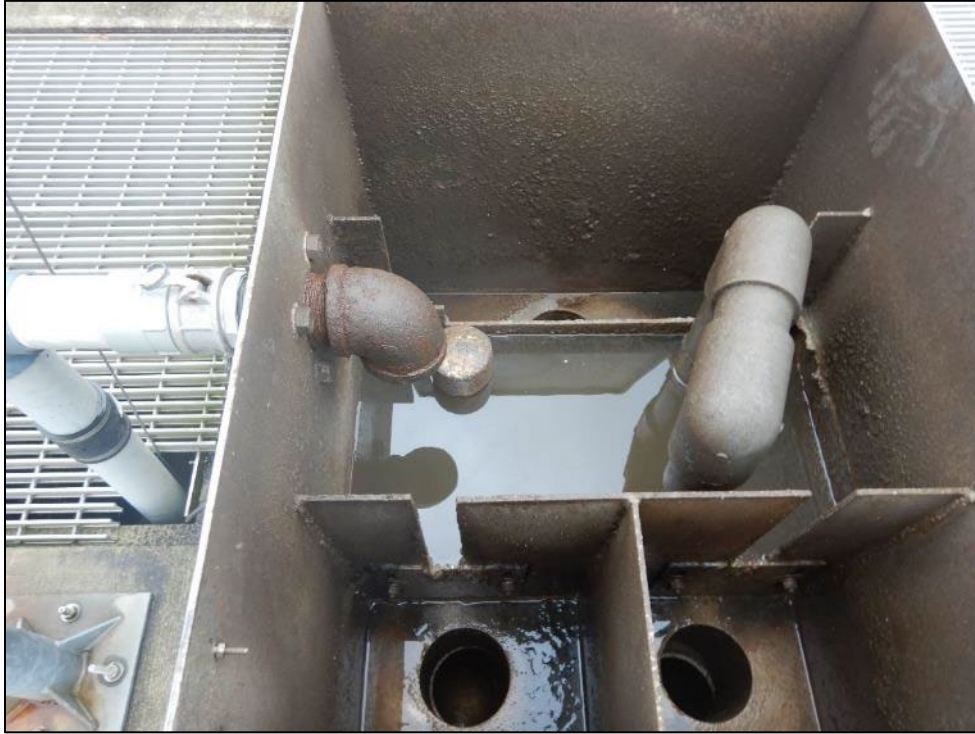
Photograph 45. Elk Garden WWTP. (DSCN9975) View inside the splitter box.
