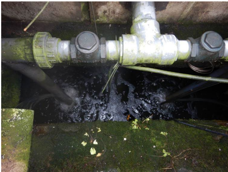
Photograph 54. Elk Garden WWTP. (DSCN9997) View inside the basin from which clarified wastewater is pumped to the sand filters.
