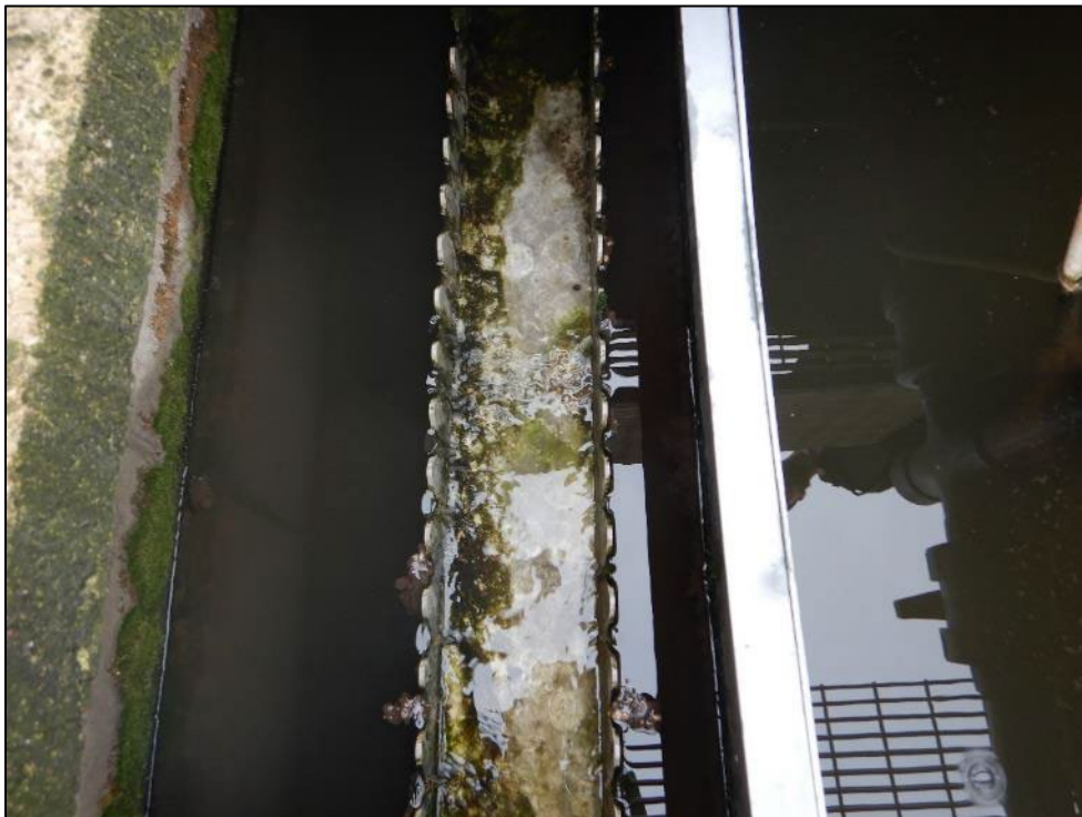
Photograph 50. Elk Garden WWTP. (DSCN9992) View of the north clarifier effluent weir. Biological growth was present on the weir and floating sludge was present adjacent to the weir.
