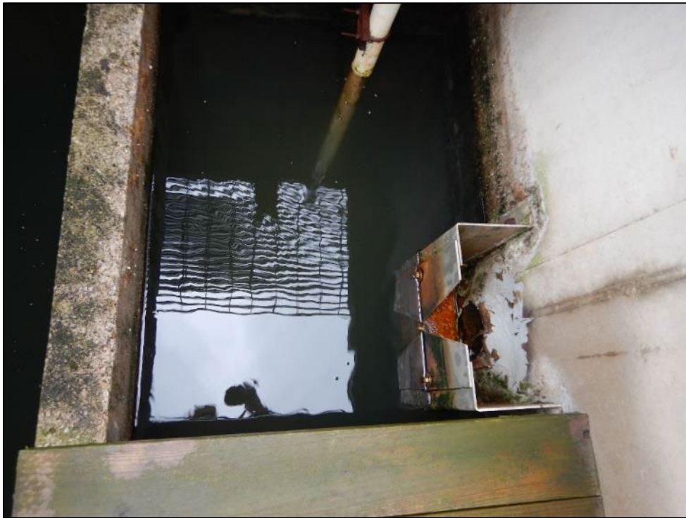
Photograph 30. Bayard WWTP. (DSCN9705) View of the chlorine contact chamber just prior to flowing to the dechlorination chamber. A pipe was present that was used to periodically pump settled solids to the equalization basin (four times per year per the General Manager).
