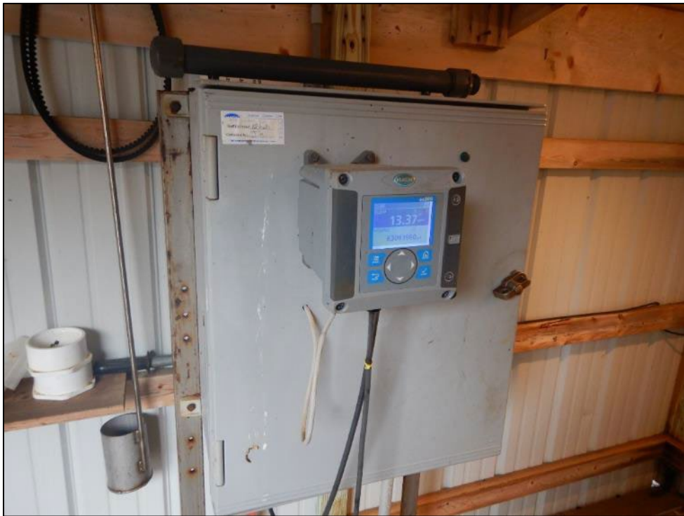
Photograph 62. Elk Garden WWTP. (DSCN0011) View of the effluent flow meter display, which stated the effluent flow was 13.37 gpm at the time of the inspection. The sticker on the cabinet stated the flow meter was last calibrated in December 2021.
