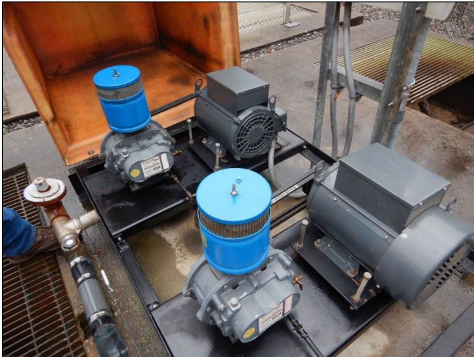
Photograph 4. Gormanian WWTP. (DSCN9626). View of the two blowers.
