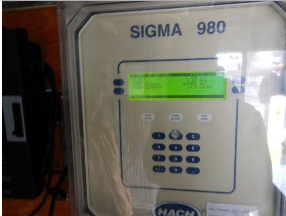
Photograph 33. Bayard WWTP. (DSCN9723) View of flow meter display. The display stated that the flow was 1.03 gpm based on a water level of 1.358 inches. The sticker on the display stated the meter was last calibrated in December 2021.
