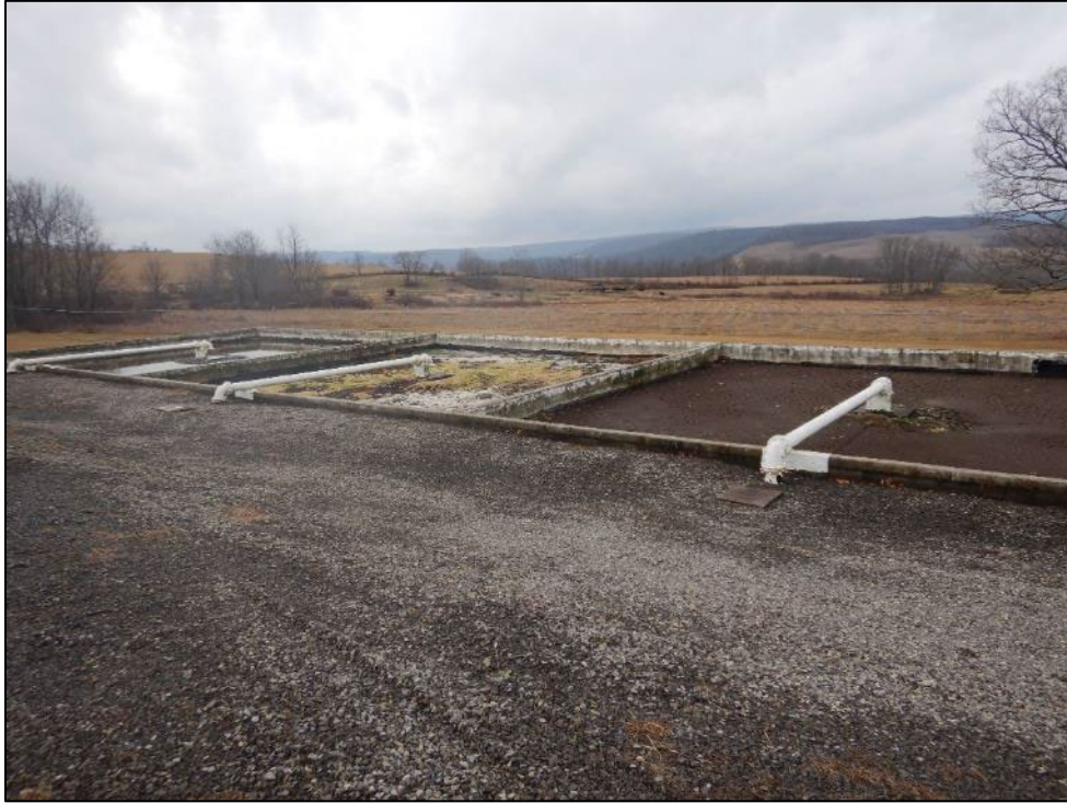
Photograph 55. Elk Garden WWTP. (DSCN0001) View of the three sand filters. The Permittee operates one filter at a time; the General Manager stated that each filter is capable of treating the rated capacity of the WWTP (50,000 gpd).
