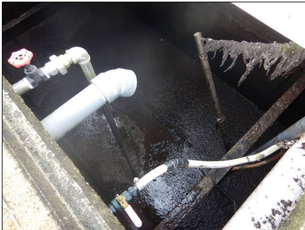
Photograph 52. Elk Garden WWTP. (DSCN9988) View inside the north sludge holding tank. The tank had been pumped out during the inspection; the Permittee had identified an air delivery line that needed to be repaired.
