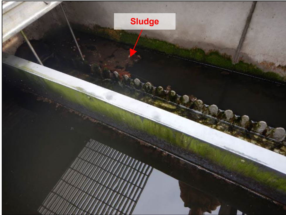
Photograph 51. Elk Garden WWTP. (DSCN9994) View of the north clarifier effluent weir. Biological growth was present on the weir and floating sludge was present adjacent to the weir.
