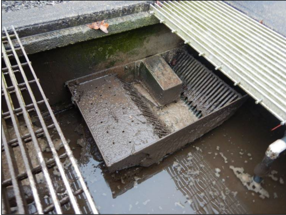
Photograph 3. Gormanian WWTP. (DSCN9614) View of the influent bar screen.
