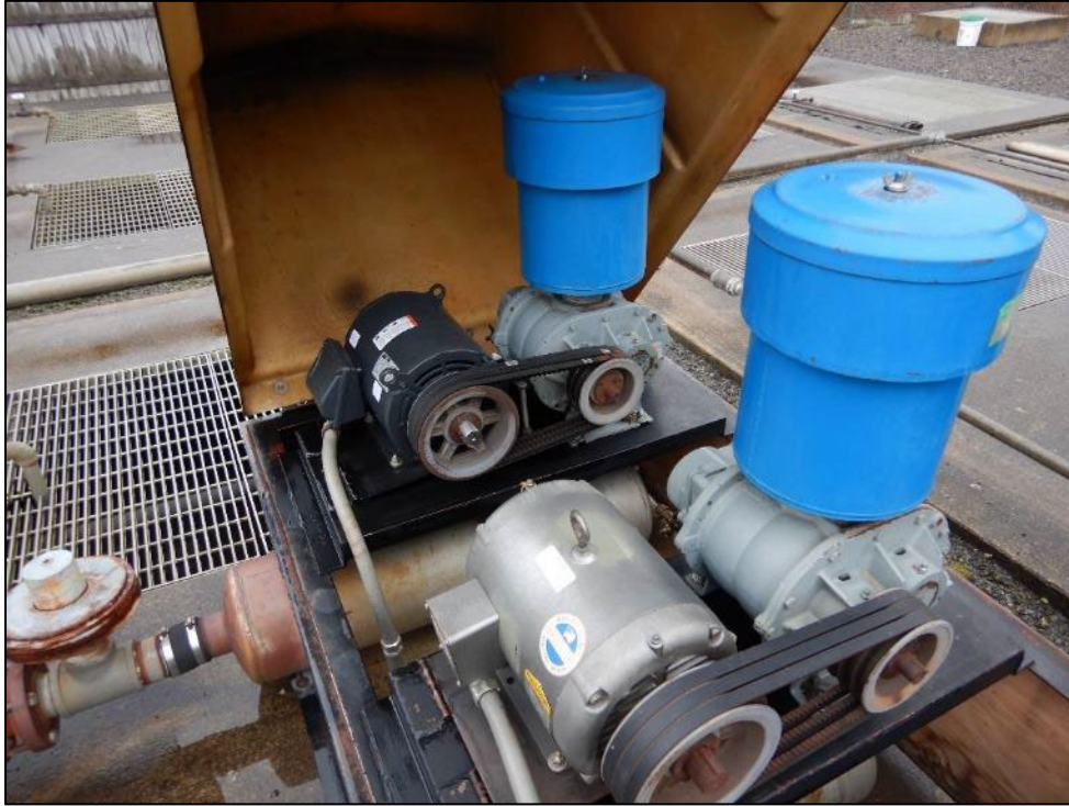
Photograph 23. Bayard WWTP. (DSCN9683) View of the two blowers.
