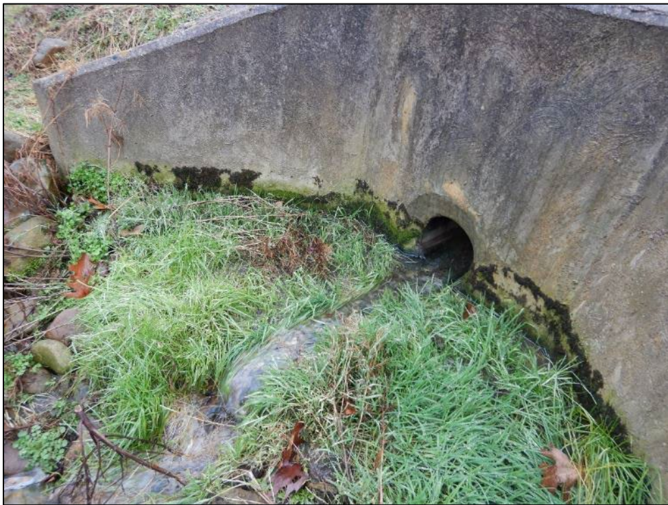
Photograph 38. Bayard WWTP. (DSCN9730) View of Outlet 001 pipe. The effluent appeared clear and free of solids and debris.
