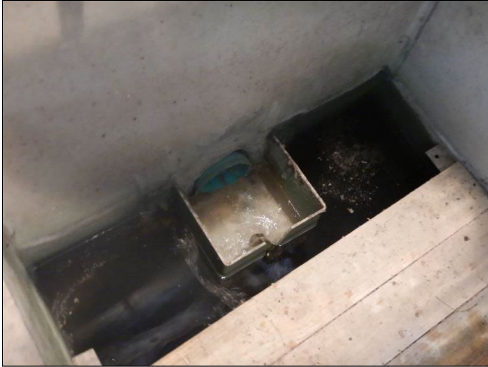
Photograph 61. Elk Garden WWTP. (DSCN0016) View of dechlorinated effluent flowing into a pipe that leads to Outlet 003.
