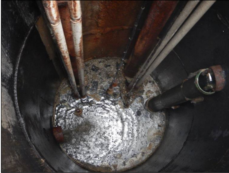
Photograph 17. Bayard WWTP. (DSCN9658) View inside the influent pump station wet well. Some fats, oils, and grease were present on the wastewater surface inside the wet well. The General Manager stated the floats are cleaned twice per year. There are two floats for pump operation (one for each pump) and two floats for level alarms (one high level and one low level).
