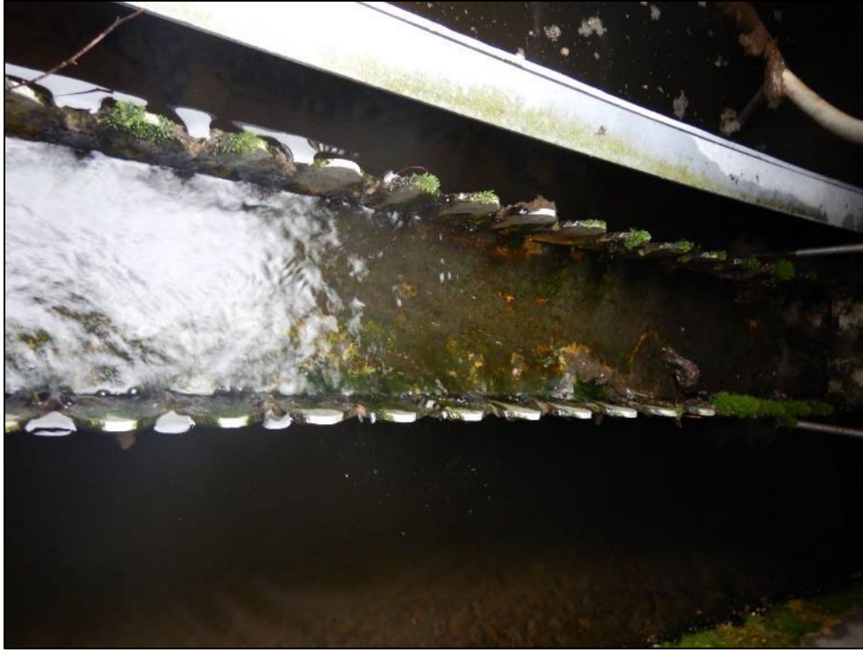
Photograph 49. Elk Garden WWTP. (DSCN9986) View of the south clarifier effluent weir. Biological growth was present on the weir.
