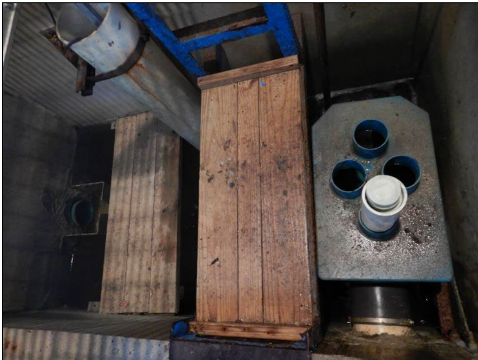
Photograph 60. Elk Garden WWTP. (DSCN0014) View of the dechlorination unit.
