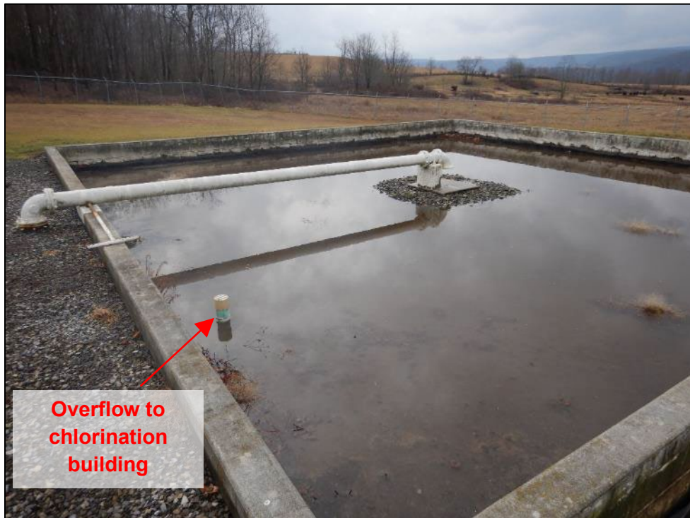
Photograph 58. Elk Garden WWTP. (DSCN0006) View of the southernmost sand filter which was in service at time of the inspection.
