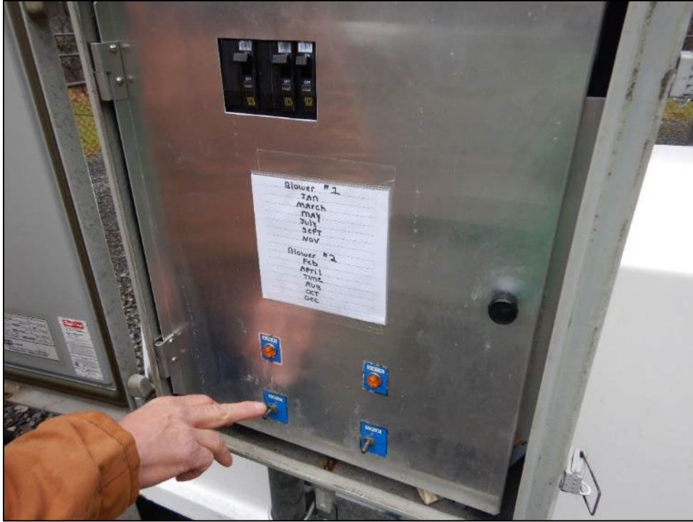
Photograph 5. Gormanian WWTP. (DSCN9624) View inside the blower control cabinet. A schedule was posted inside that indicated that each blower is cycled into the lead operating position every other month.
