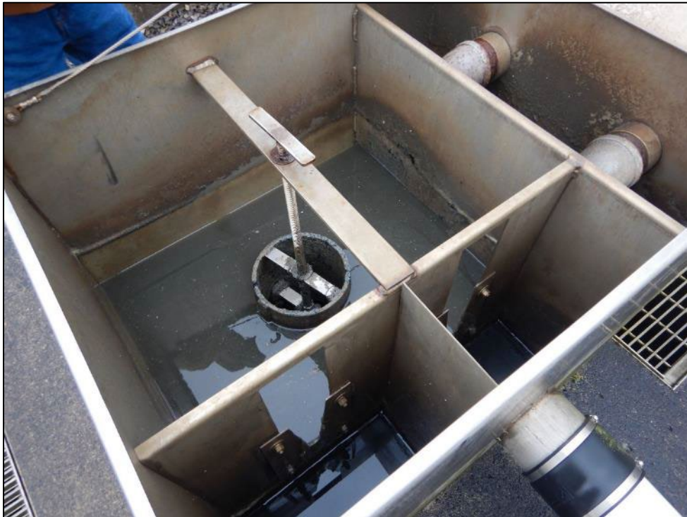
Photograph 20. Bayard WWTP. (DSCN9674) View inside the splitter box that sits above the equalization basin. The valve regulates hydraulic flow through the plant.
