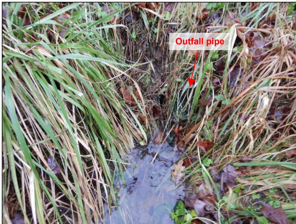
Photograph 14. Gormanian WWTP. (DSCN9643) View of Outlet 002. The outfall pipe is obscured from view by vegetation. The effluent appeared clear and free of solids and debris at the time of the inspection.
