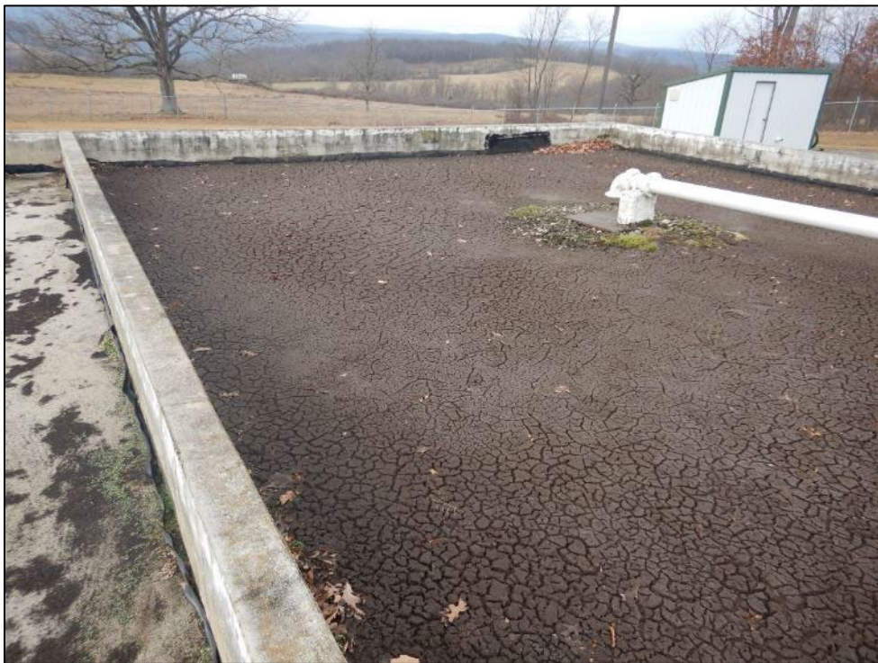
Photograph 56. Elk Garden WWTP. (DSCN0005) View of northernmost sand filter which was not in service at the time of the inspection. The Permittee was allowing the sludge to dry before manually removing it.
