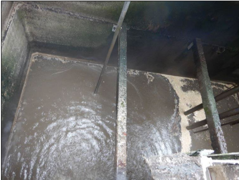
Photograph 44. Elk Garden WWTP. (DSCN9973) View inside the second chamber of the flow equalization basin. The basin is connected to the first chamber from pipes below the wastewater surface. The General Manager stated this chamber is aerated to prevent septic conditions from occurring.
