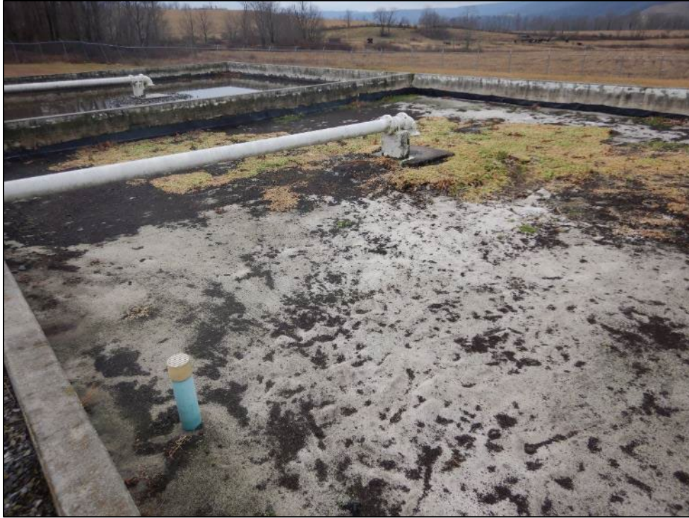
Photograph 57. Elk Garden WWTP. (DSCN0004) View of the sand filter shown in the middle of Photograph 56. The General Manager stated the standpipe shown in the foreground of the photograph is an overflow that flows to the chlorination building (each filter is equipped with such an overflow pipe).
