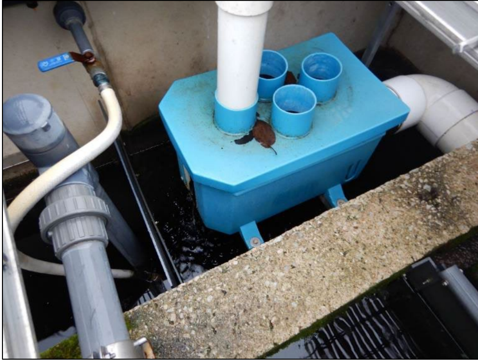
Photograph 9. Gormanian WWTP. (DSCN9619) View of the chlorination unit and chlorine contact chamber.
