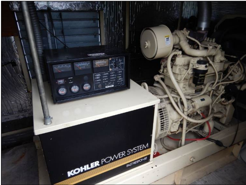
Photograph 40. Bayard WWTP. (DSCN9706) View of emergency backup generator unit for the WWTP.
