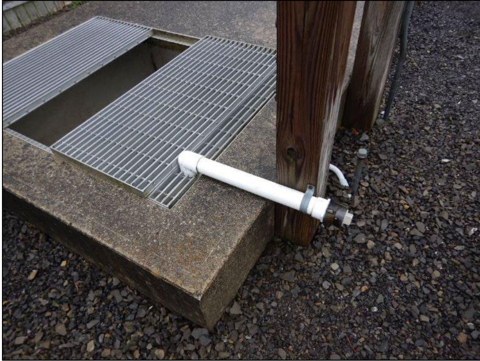
Photograph 31. Bayard WWTP. (DSCN9707) View of the pipe in the chlorine contact chamber used to transfer solids from the chlorine contact chamber to the equalization basin. The General Manager stated a trash pump is connected to the piping to transfer the solids.
