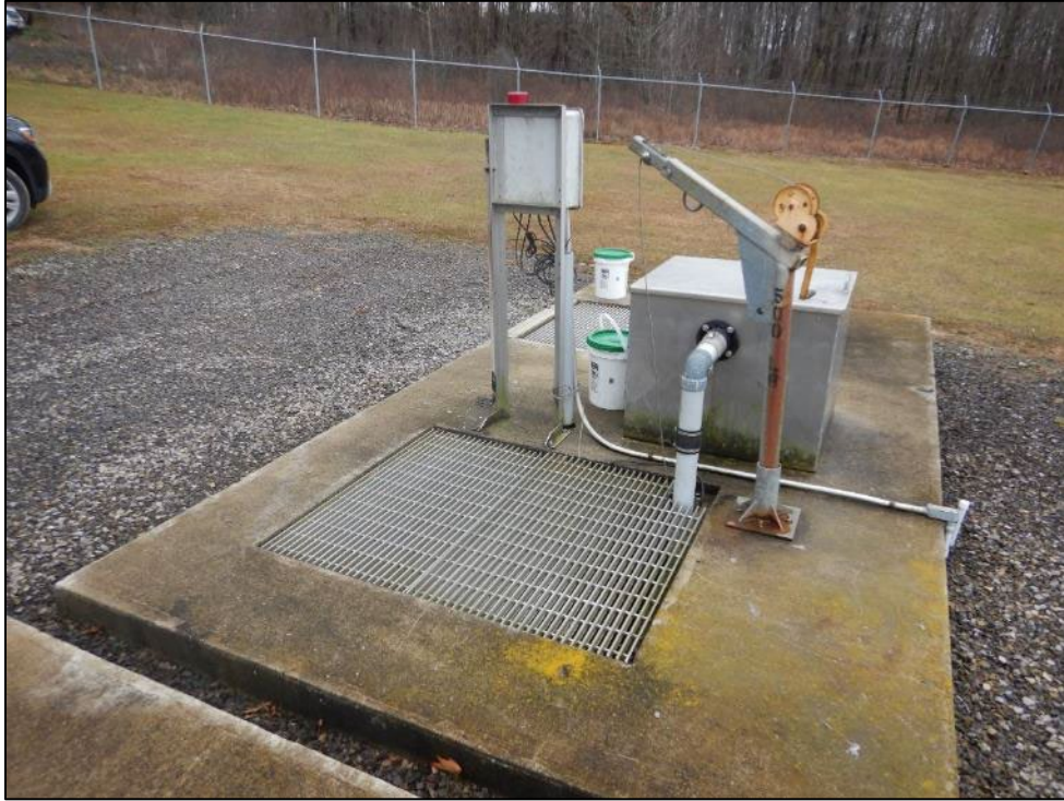
Photograph 41. Elk Garden WWTP. (DSCN9976) View of the first chamber of the influent equalization basin and splitter box.
