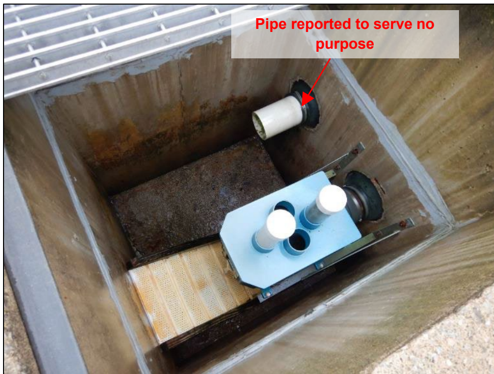
Photograph 34. Bayard WWTP. (DSCN9711) View inside the dechlorination chamber. The board underneath the dechlorination unit was installed to increase dissolved oxygen concentrations of the treated effluent. The General Manager stated the second pipe did not serve a purpose (it was a relic of the original plant design but never placed into service). He stated it was not an overflow pipe from a treatment unit upstream of the dechlorination chamber.
