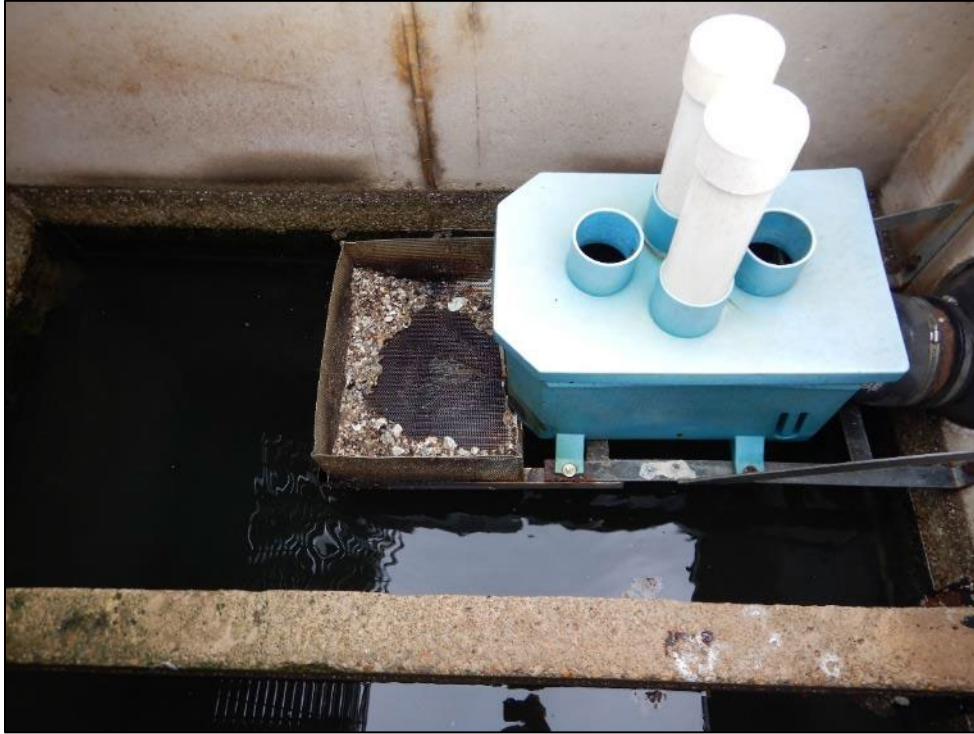
Photograph 29. Bayard WWTP. (DSCN9703) View of the chlorination unit. A screening mechanism had been installed post-chlorination to capture debris.
