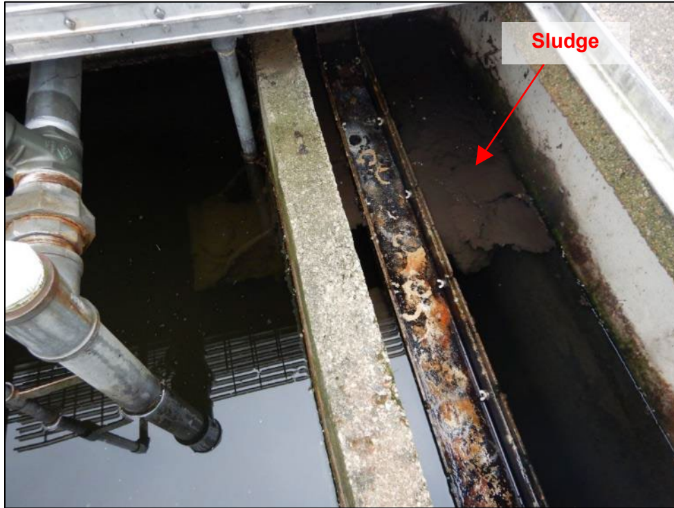
Photograph 25. Bayard WWTP. (DSCN9691) View inside the northern clarifier. Floating sludge was present adjacent to the effluent weir.
