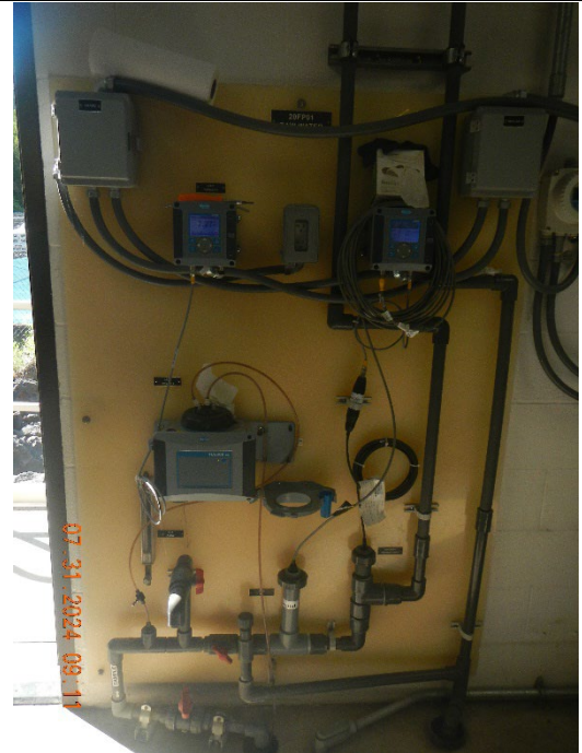
Photo #:06 (DSCN3845) Description: Photo of raw water monitoring equipment.
