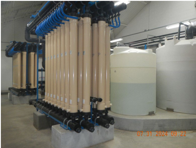
Photo #:07 (DSCN3846) Description: Photo of membrane filtration units.
