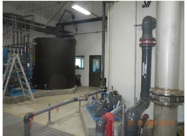
Photo #:08 (DSCN3847) Description: Photo of neutralization tank.
