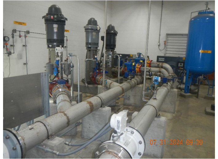
Photo #:10 (DSCN3849) Description: Photo of distribution pumps.
