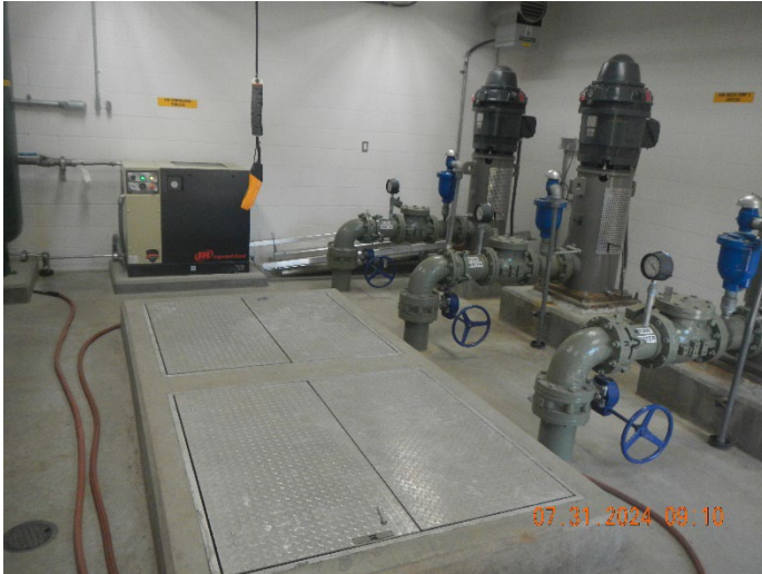
Photo #:05 (DSCN3844) Description: Photo of raw water pumps within the raw water pump station.
