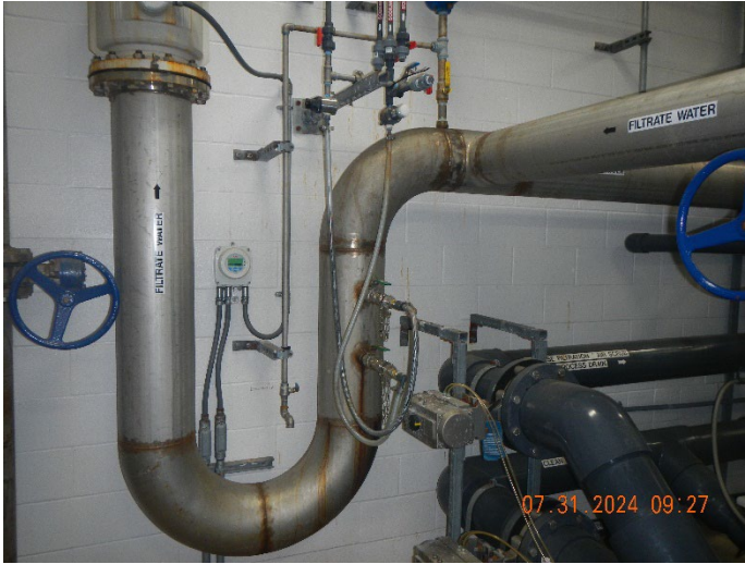
Photo #:09 (DSCN3848) Description: Photo of filtrate water piping.
