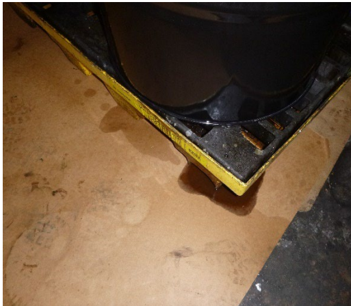
Photograph 27: release on cardboard and secondary containment in Aerosol Line SAA - P1030634.JPG
