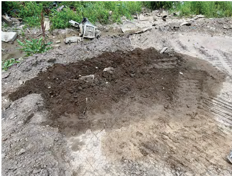
Photo 32 significant ground discoloration
