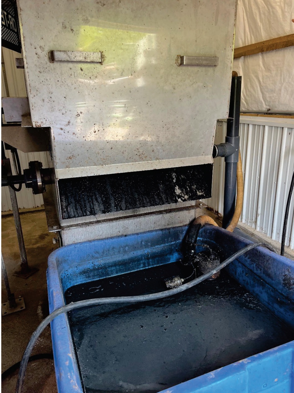
Photograph 2: The fine screen removes solids from the wastestream. The solids collected in the collection tub are pumped back to the equalization pump pit.
