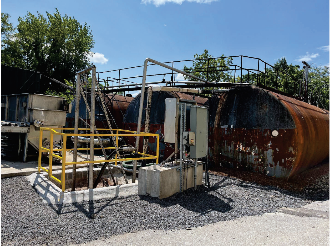
Photograph 4: The on-site treatment systems equalization tank (right) is to the right and two aeration tanks (left).
