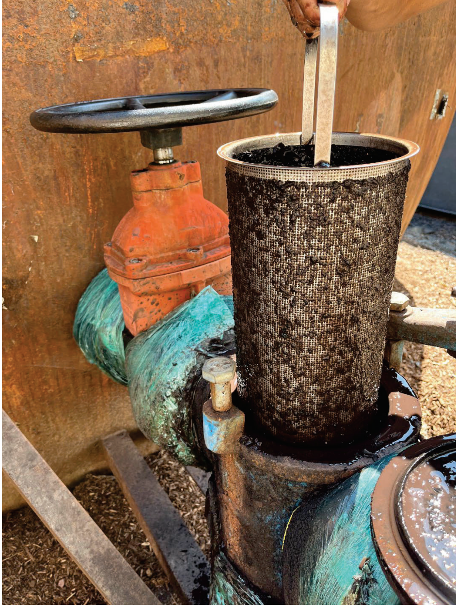
Photograph 3: The microscreen further screens out solids from the wastestream.
