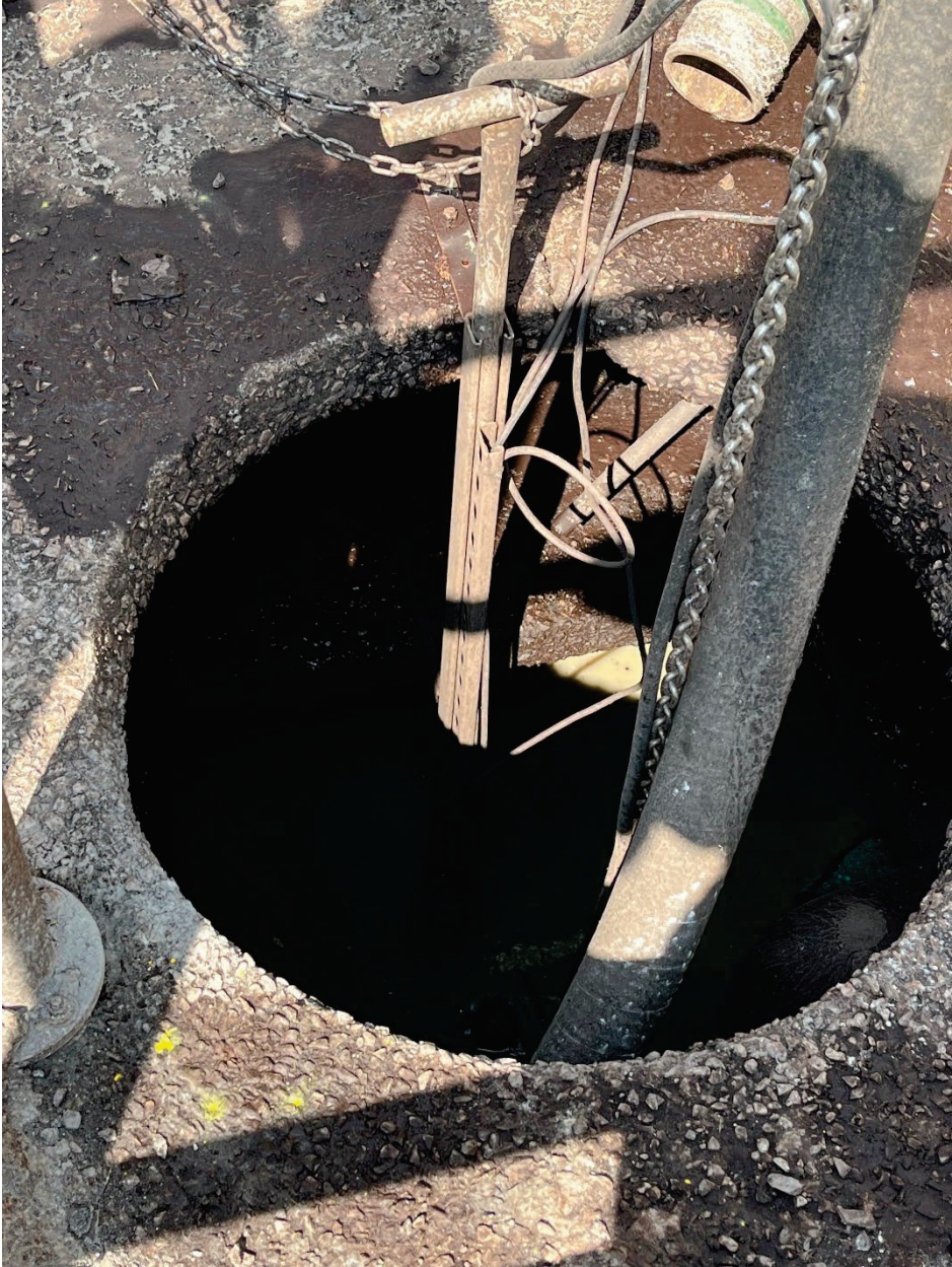
Photograph 1: The Equalization Pump Pit collects the facilities process water and storm water.
