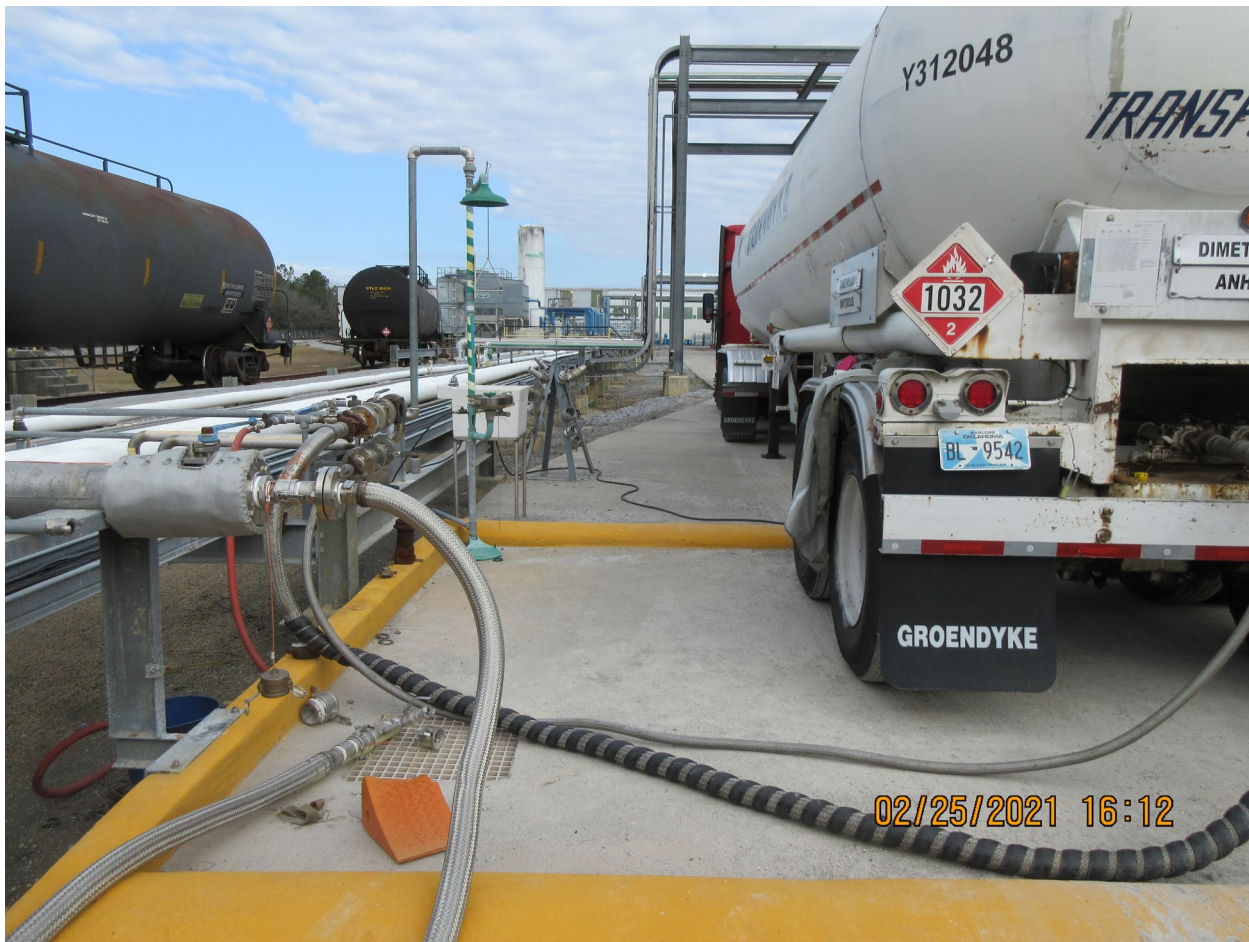
Photo 8 – Tanker Truck Loading Area #6
