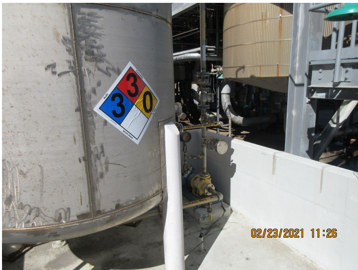
Photo 4 – Ancillary equipment for Tank-830
