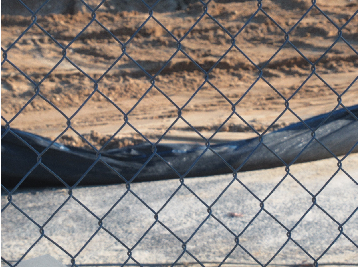
IMG_0287: Silt fence needing replacement.
