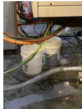
Photo-6 Molding Press 227/228 Open two 5-gallon Used Oil Container
