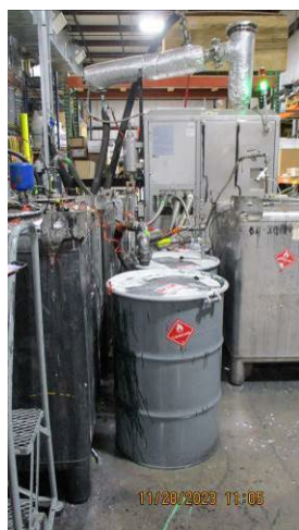
Figure 11: IMG_0231.JPG – Solvent Recycling System
