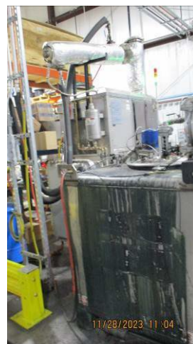
Figure 10: IMG_0230.JPG – Solvent Recycling System
