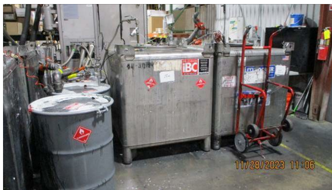
Figure 12: IMG_0232.JPG – Solvent Recycling System
