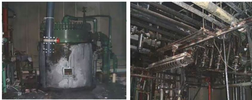
Figure. An example of a fire accident caused by static electricity
