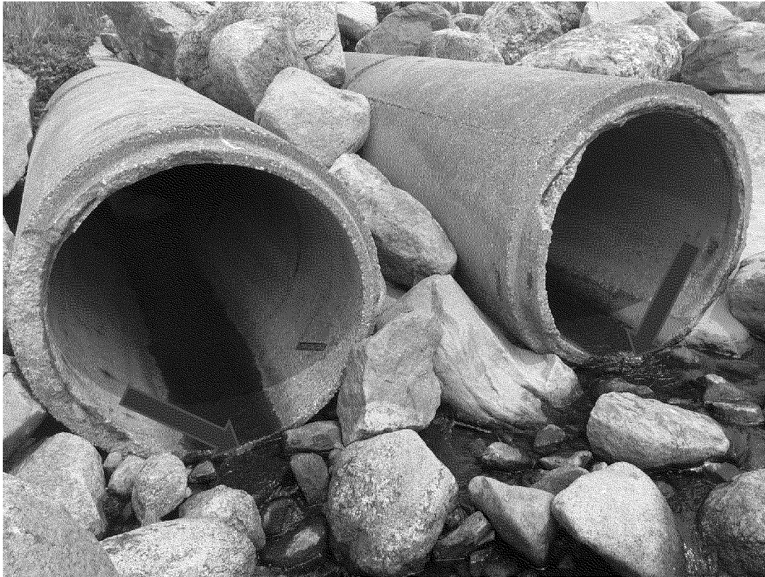
SB07 (left) & SB08 (right): Pair of concrete outfalls at the northern end of Scarborough Beach near the ruins. Sample collection points indicated by red arrows.
