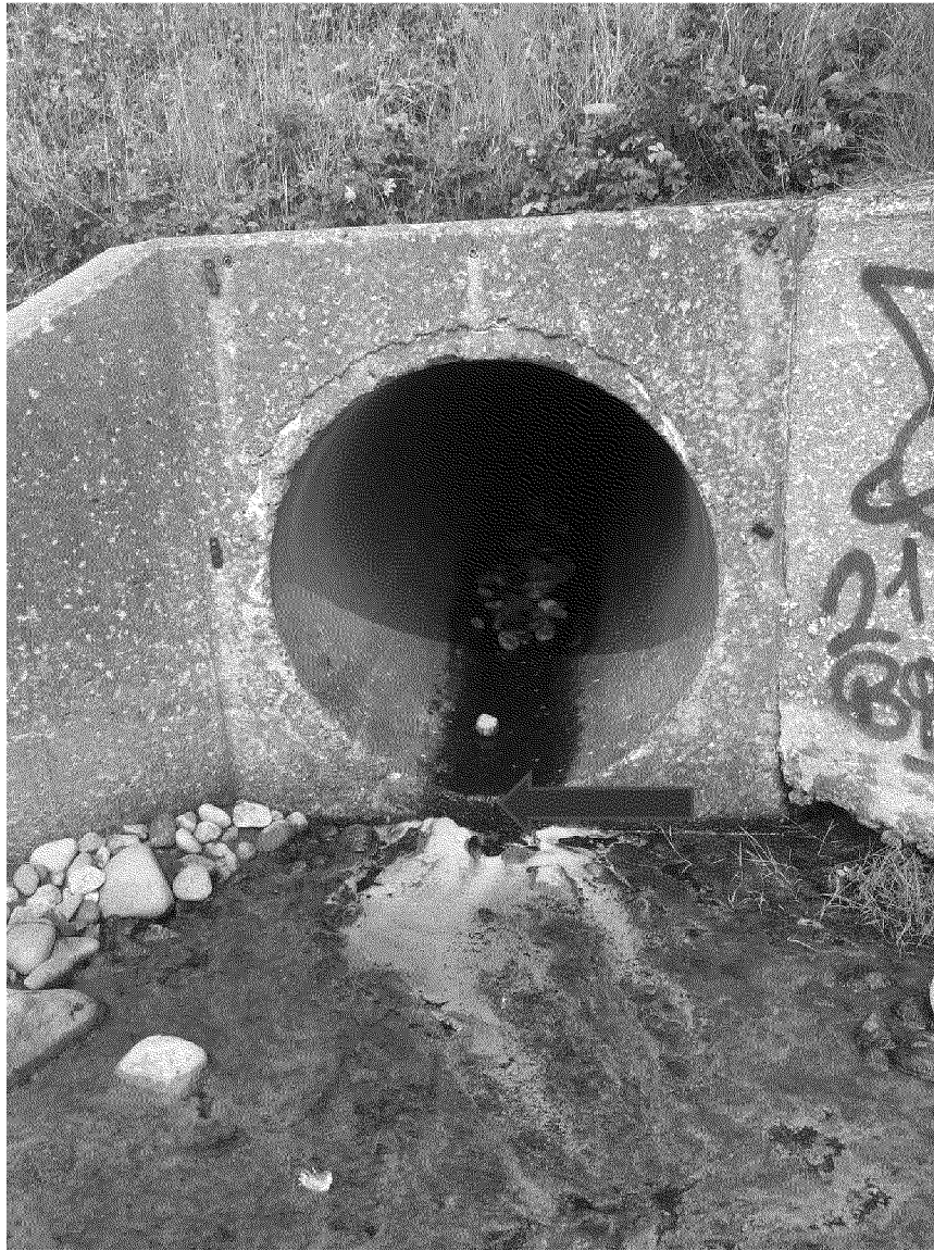
SB02: Close-up of SB02. Note the green algae growth and orange suds in the pool downstream of the pipe. Sample collection point indicated by a red arrow.
