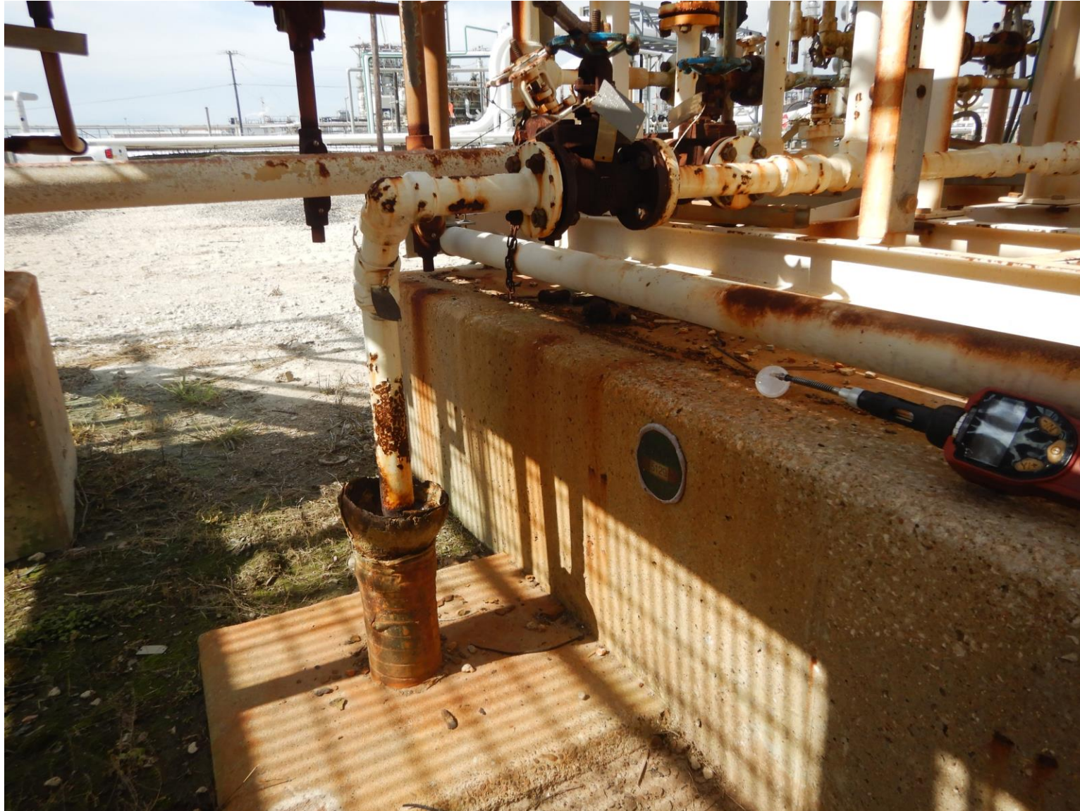
Photo 1163: WWTP F-220 seal pot drain 5/3/23 10:01 DSCN1163.jpg
