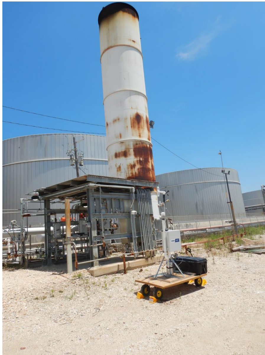
Photo 1155: EPA 1A Location near Dock 18 Thermal Oxidizer facing NE 5/1/23 12:37 DSCN1155.jpg
