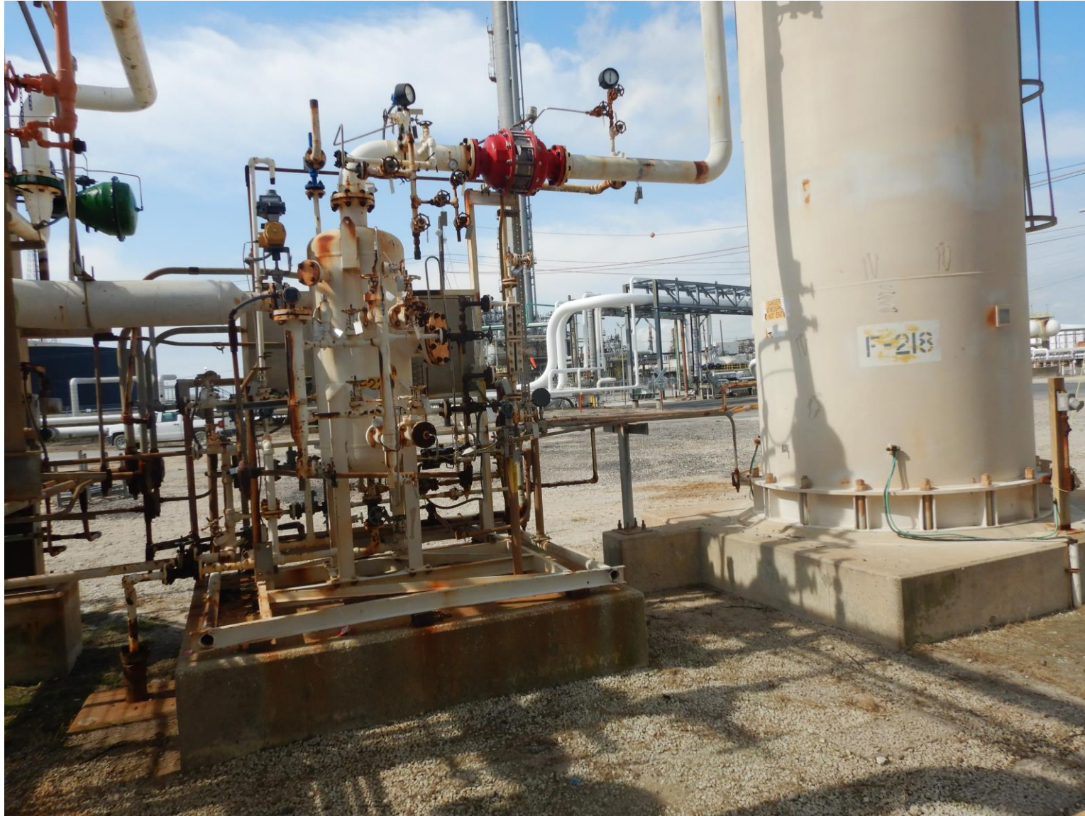
Photo 1164: WWTP thermal oxidizer and F-220 seal pot (zoomed out) 5/3/23 10:07 DSCN1164.jpg
