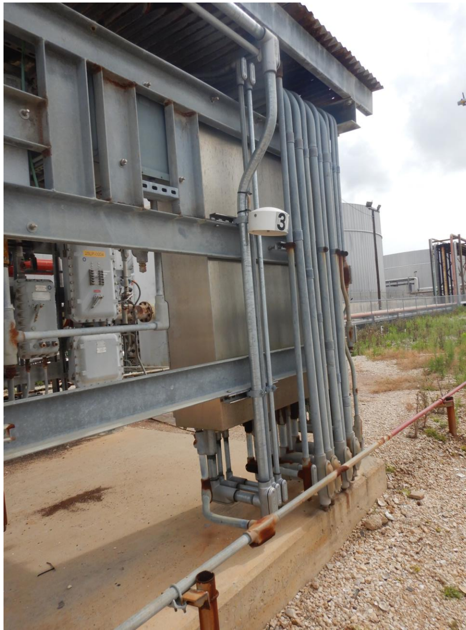
Photo 1160: Shelter 31 placement after facility corrected 5/2/23 10:28 DSCN1160.jpg
