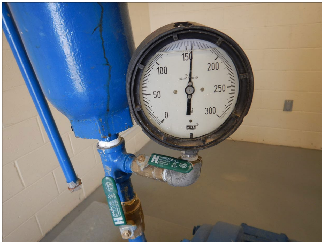
Photograph 22. W0002 Pump Line Pressure Gauge View of an additional pressure gauge on the W0002 pump line, immediately prior to the raw water being transferred to the W0001 building. The W0002 pump was not operating during the inspection. This gauge also read approximately 158 psi.
