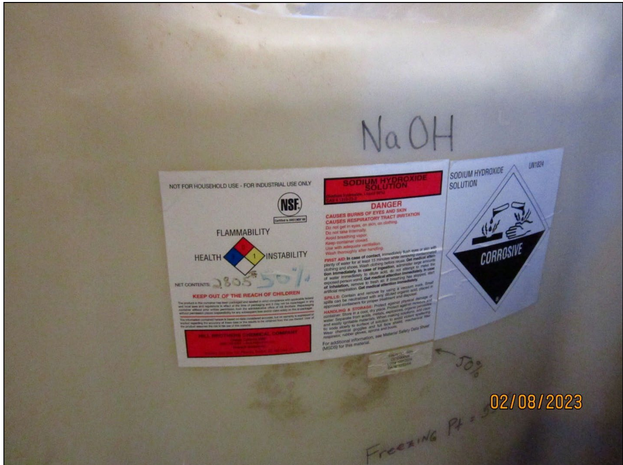
Photograph 32. Sodium Hydroxide Tote, Sodium Hydroxide Storage/Pump Room View of the sodium hydroxide (caustic soda) storage tote in the sodium hydroxide room. The tote was labeled with a marker stating a freezing point of 53° F.
