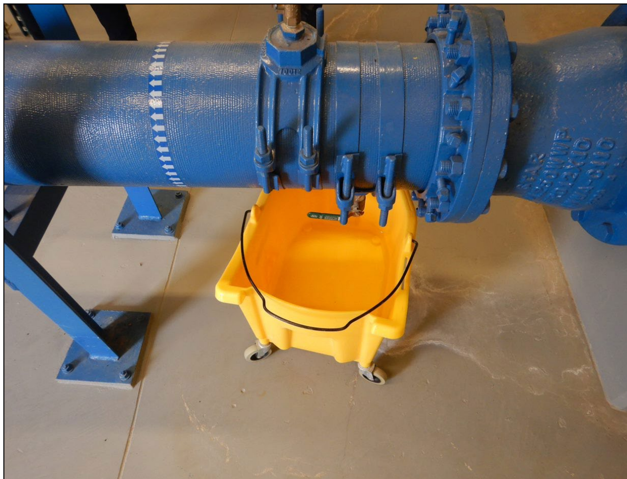
Photograph 23. W0002 Pump Line Sample Tap View of the W0002 pump line and raw water sample tap that was leaking into a bucket during the inspection. Operators indicated that they had the parts on hand to make the repair.
