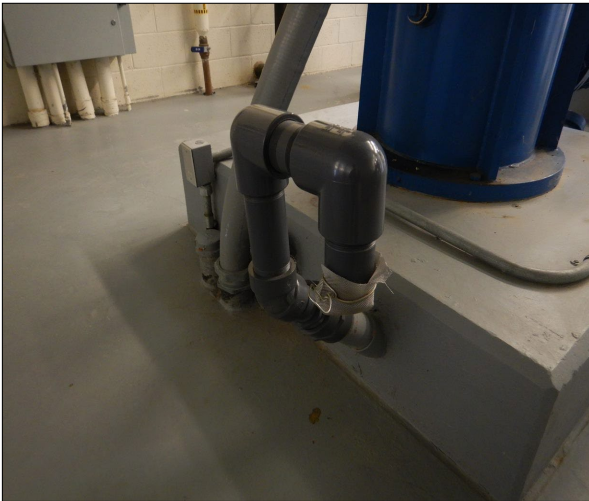
Photograph 14. W0002 Air Relief Valve View of a screened air relief valve at Wellhead Casing No. 2.
