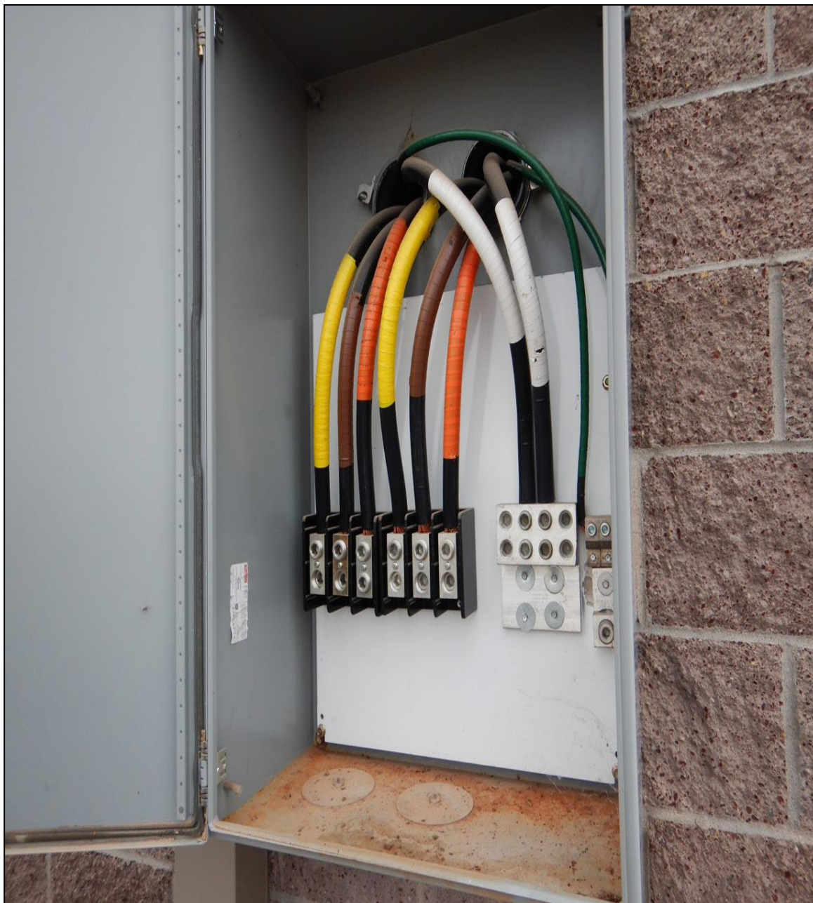
Photograph 25. Switch Gear MCC Box, W0002 Building View of the inside of the switch gear connection cabinet where a trailer generator could be wired up to provide power in the event of a power loss/failure.
