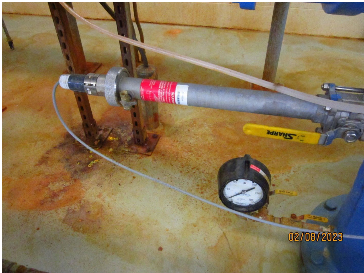
Photograph 50. pH Probe, Treatment Room View of the “finished water” pH probe located at the end of the treatment system, after chemical injection. There was also a pressure gauge present at this location which was reading 0 psi. Brown staining can also be seen on the floor and infrastructure in this image.
