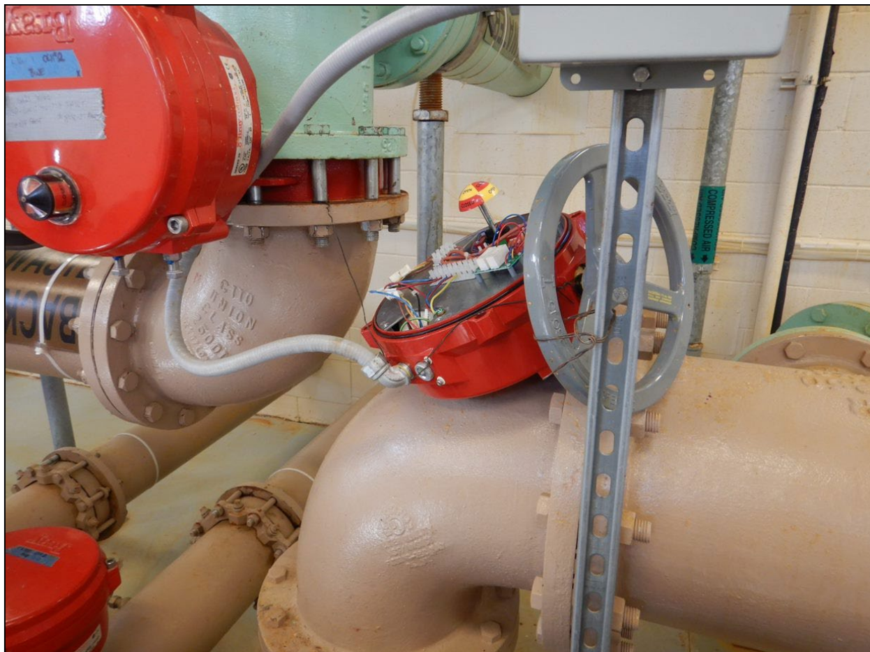
Photograph 41. Failed Effluent Valve Actuator, Treatment Room View of the failed actuator to the failed effluent valve in the treatment room. The actuator was supported by bailing wire above the valve waiting on repair.
