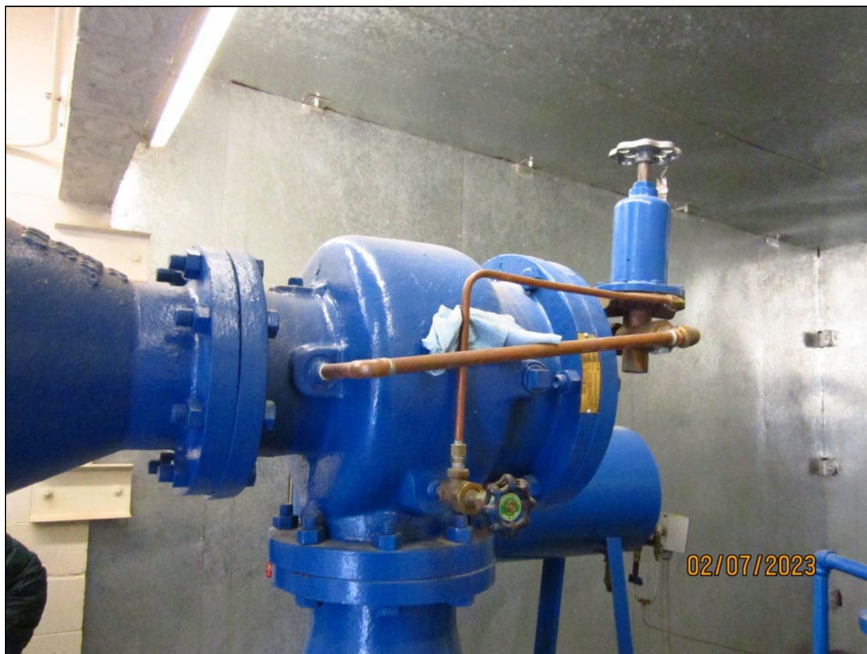
Photograph 13. W0002 PRV View of the PRV on the pump-to-waste line extending from the W0002 pump raw water line.
