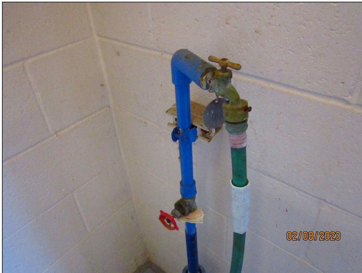
Photograph 31. Hose Bib, Ferric Chloride Room View of a hose bib in the ferric chloride room. The bib contained backflow prevention. The hose bib was discolored/stained brown.
