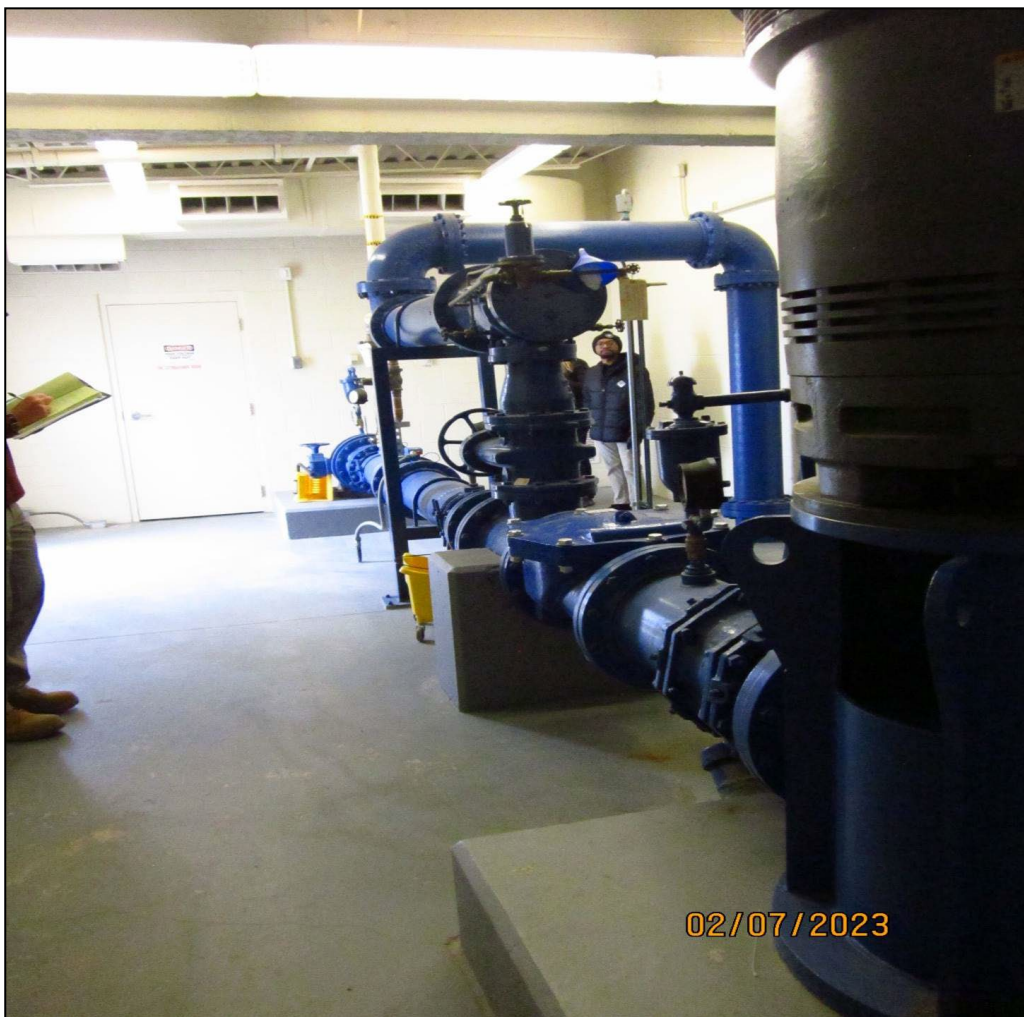
Photograph 12. Well No. 2 (W0002) View of the W0002 line, including the pump, air relief valves, check valve and pump-to-waste line that had an isolation valve.
