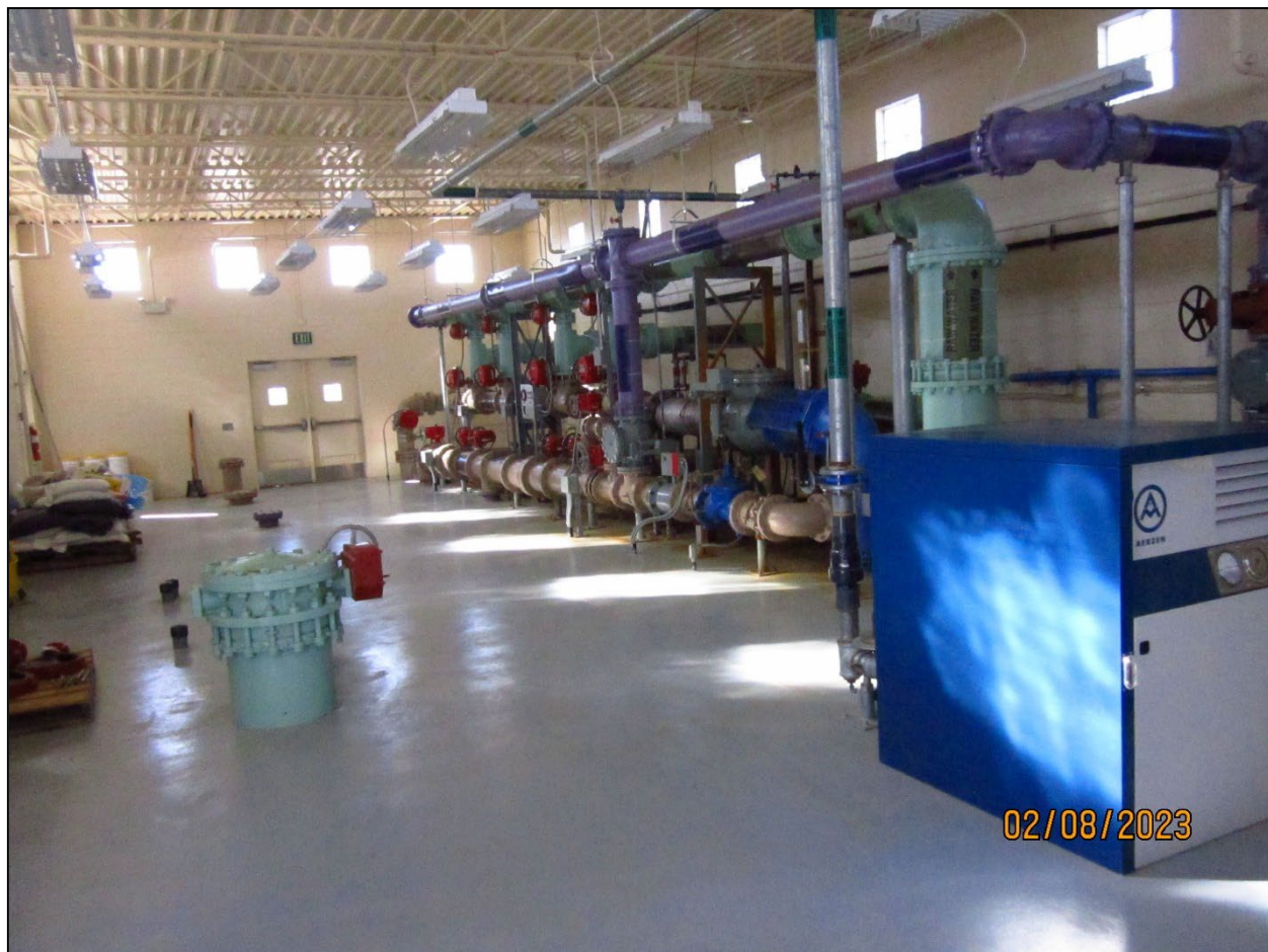
Photograph 37. Treatment Room View of the treatment room for the Sandia Resort and Casino PWS. The filter units were located on the exterior of the building.
