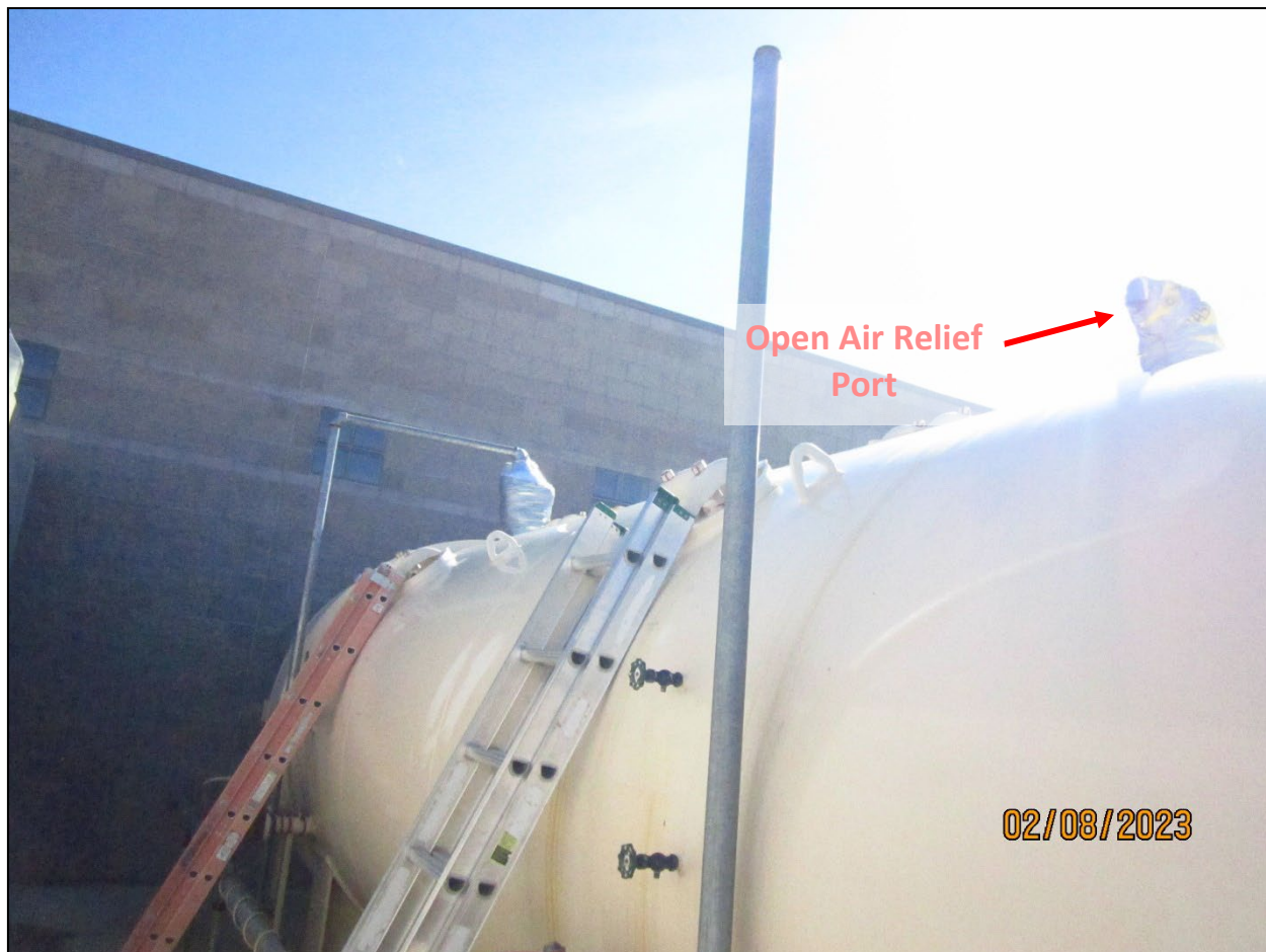
Photograph 47. Filter Unit No. 2 View of mixed media (anthracite, sand, and gravel) Filter No 2. The air relief port at the right of the image was recently replaced and did not contain a screen over its opening or an extension line so that releases would not drain on tank.
