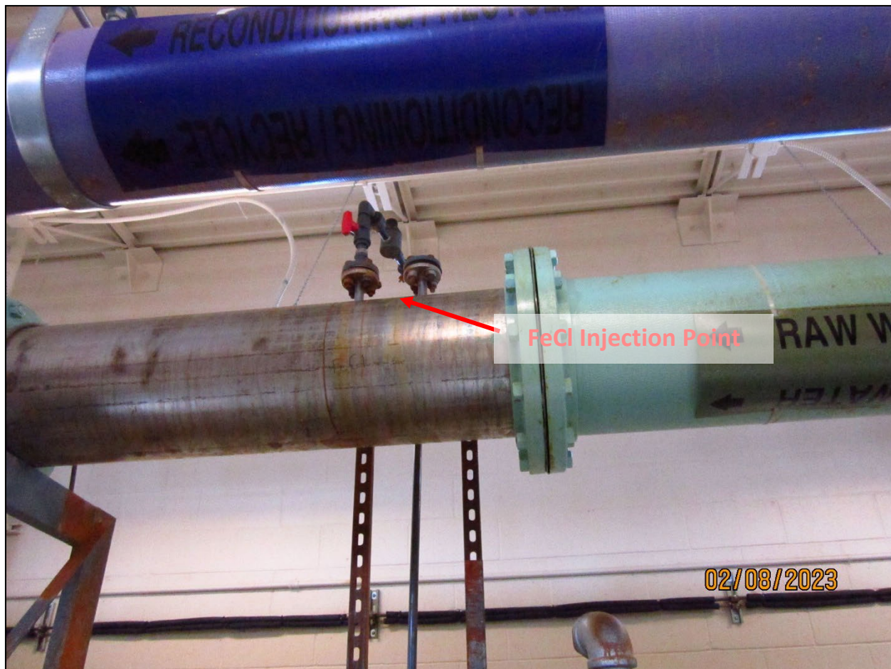
Photograph 44. Ferric Chloride Injection, Treatment Room View of the ferric chloride injection point in the treatment system prior to filters. There was brown staining/rust around the injection point.
