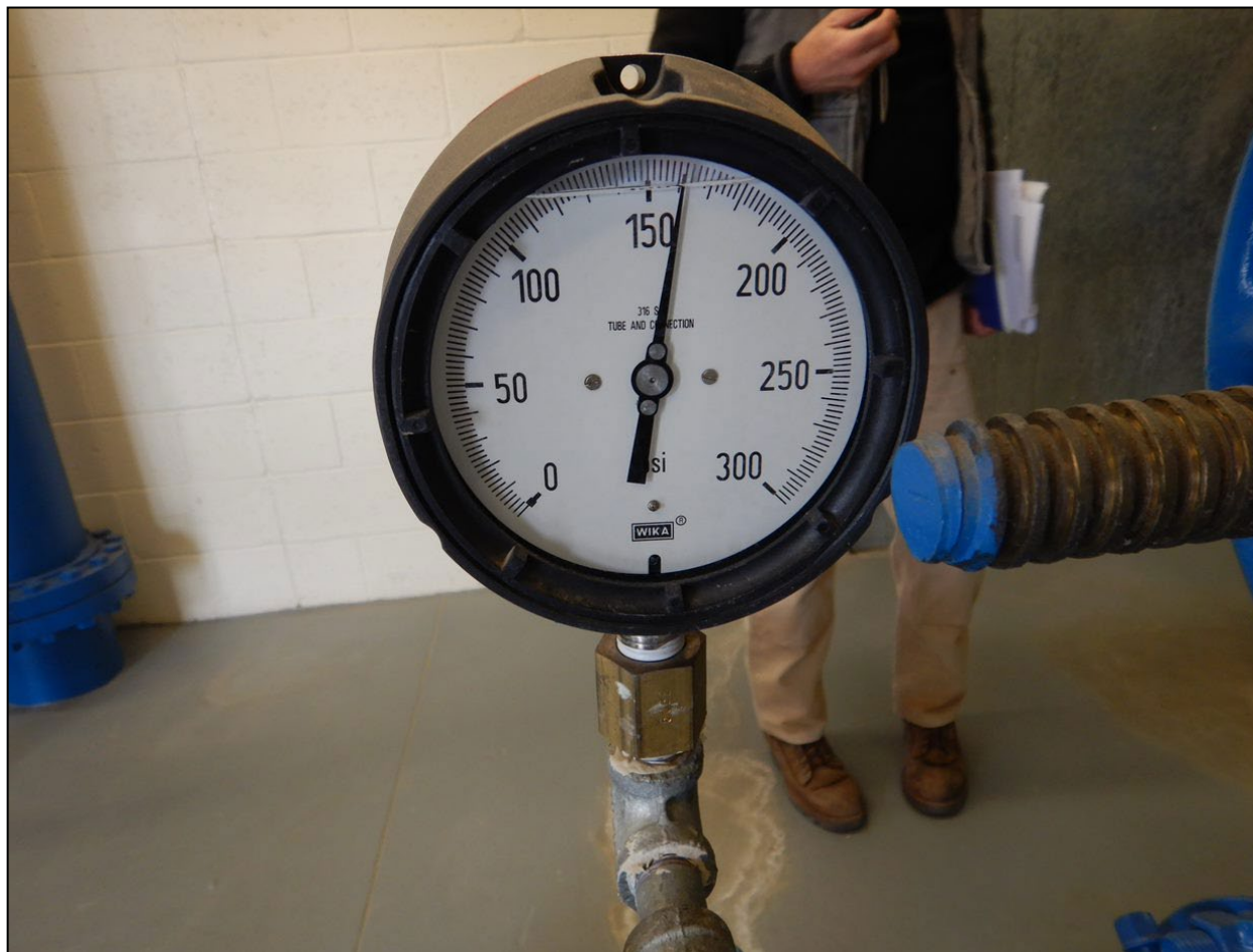
Photograph 21. W0002 Pump Line Pressure Gauge View of one of the pressure gauges on the W0002 pump raw water line, downstream of the check valve. The W0002 pump was not operating during the inspection. The gauge read approximately 162 psi.
