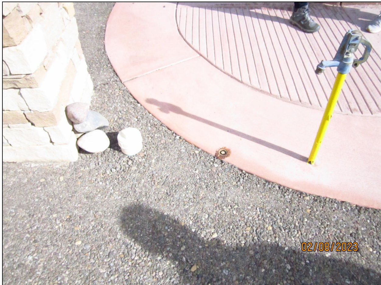
Photograph 64. RV Potable Water and Sanitary Sewer Clean-Out Hookups, Casino Area View of one of the four RV parking spot potable water and sewer hookups outside of the casino. The RV parking spots were each serviced with a potable water and sewer connection. The potable water connections did not contain backflow prevention. The sanitary sewer clean-out locations at each parking spot were within three feet of the potable water connections.
