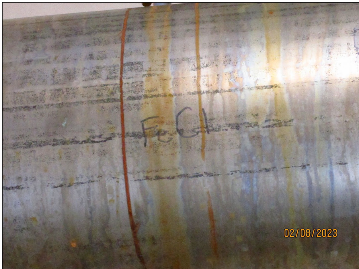
Photograph 45. Ferric Chloride Injection, Treatment Room Close up view of the ferric chloride injection pipe. The injection point was labeled with black marker, and there was brown staining/corrosion around the injection point that appears to drip downward.
