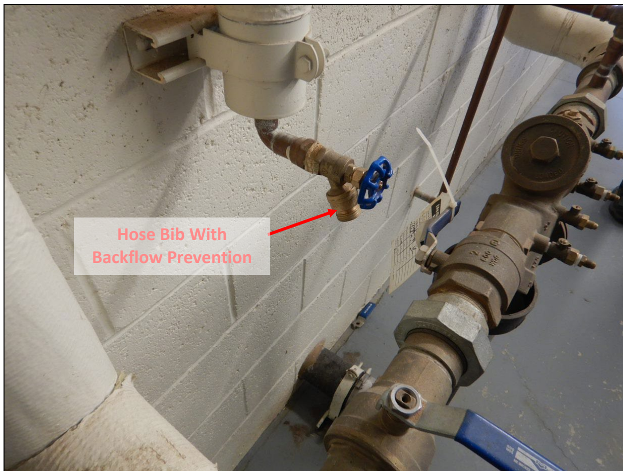
Photograph 17. Hose Bib, W0002 Building Hose bib with vacuum backflow protection and the backflow assembly for the non-potable water line servicing the well house.
