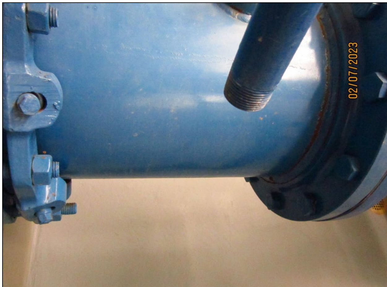
Photograph 4. Air Relief Valve, W0001 Line Close up view of an unscreened air relief valve discharge on the W0001 pump line.
