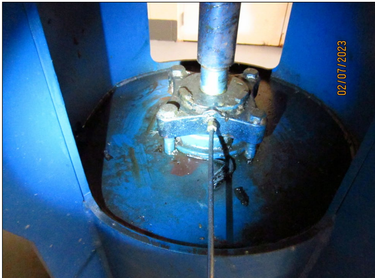
Photograph 2. Well No. 1 (W0001) Pump View of the food-grade lube line connection to the pump in the W0001 building. Some excess lube was observed.
