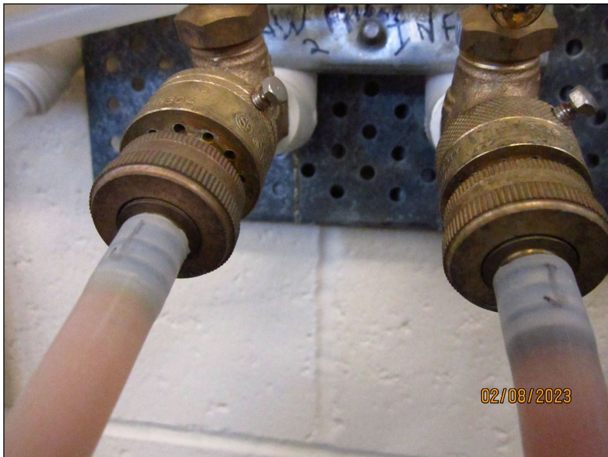
Photograph 53. Filter Nos. 1 and 2 Influent Sample Ports Close up view of the Filter Nos. 1 and 2 influent sample ports. The ports were stained brown from ferric chloride. The sample ports contained backflow prevention.
