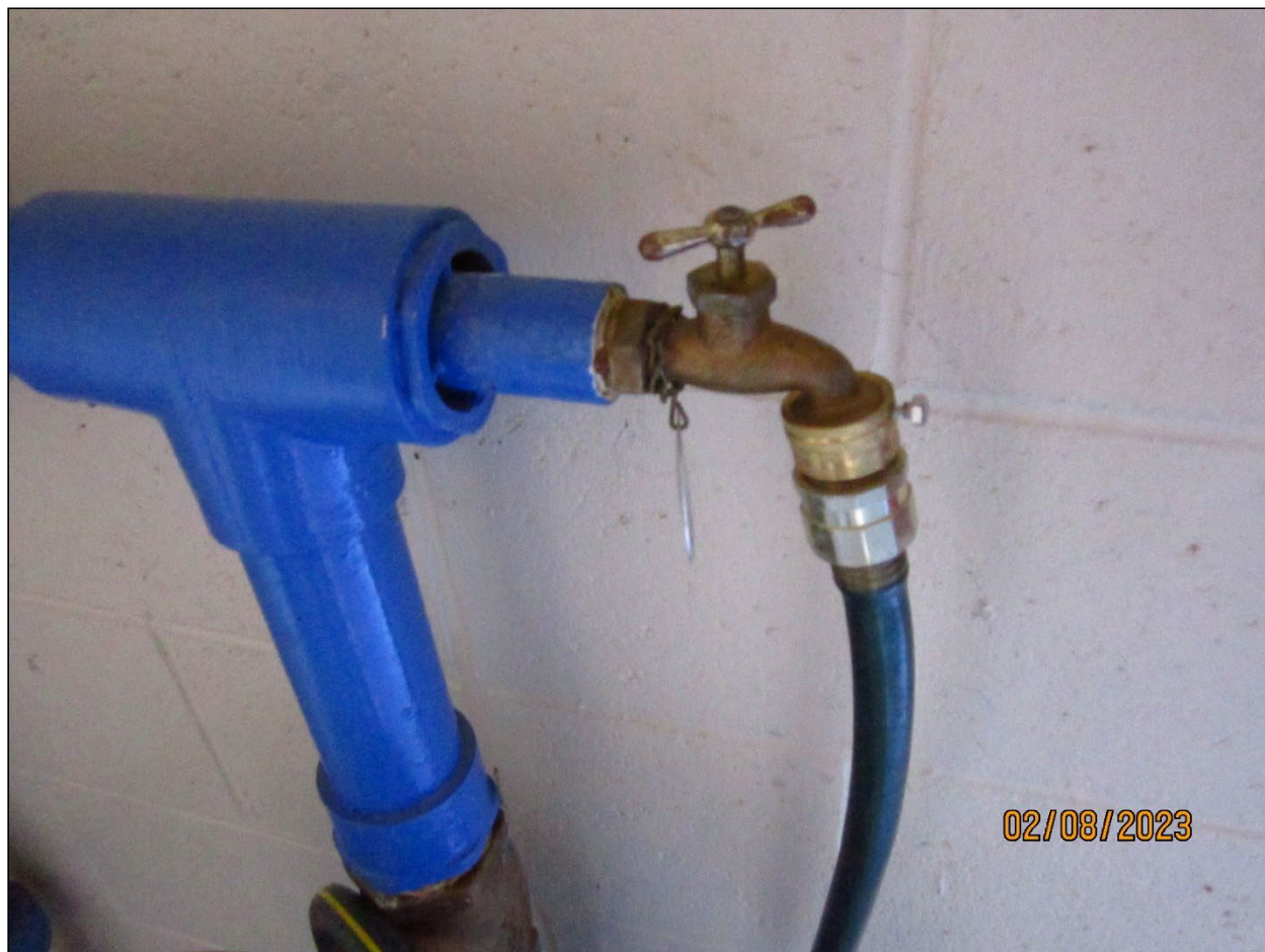
Photograph 35. Hose Bib, Sodium Hydroxide Storage/Pump Room View of a hose bib inside of the sodium hydroxide storage room. The bib contained backflow prevention.
