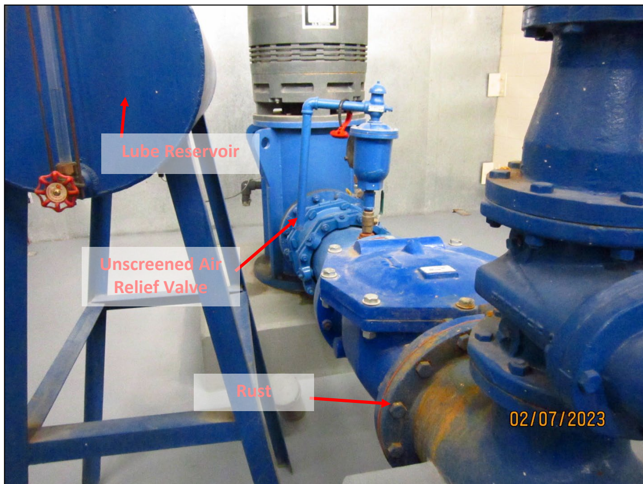
Photograph 3. Air Relief Valve, W0001 Line View of an unscreened air relief valve on the W0001 pump line. Also visible in this image is rust (immediately under the PRV) at the point where the W0001 line connects to the pump-to-waste line.
