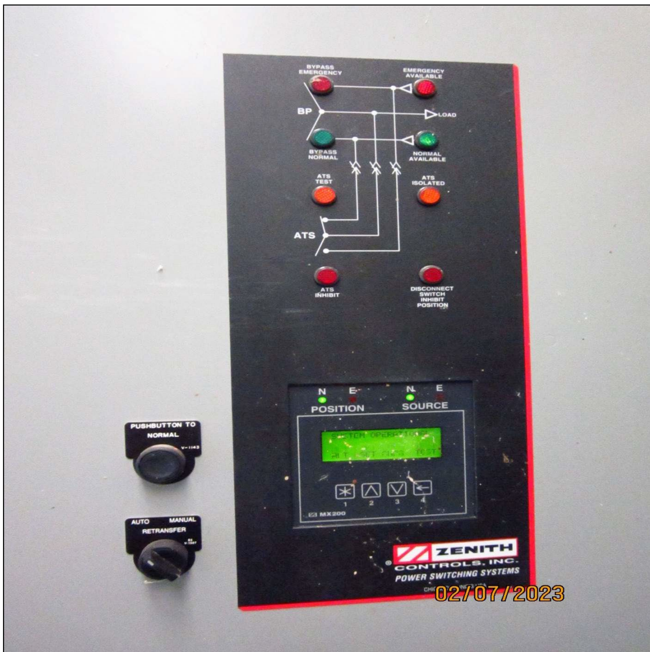
Photograph 24. Switch Gear Control Cabinet, W0002 Building View of a switch gear control cabinet that was present in the W0002 building.
