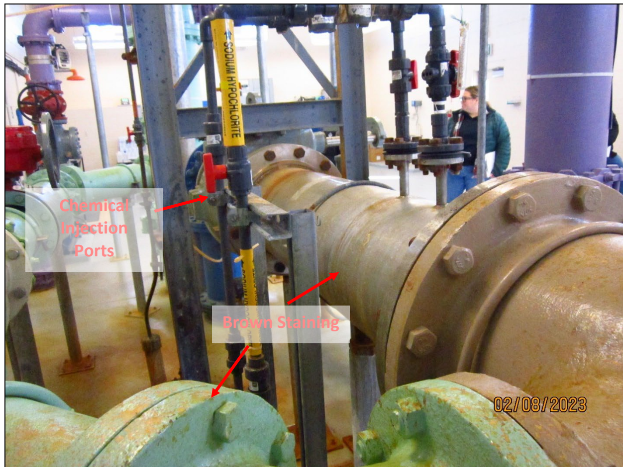
Photograph 48. Chemical Injection Point, Treatment Room View of the chemical injection point on the chemical mixing line. The system's process flow diagram indicates that the caustic soda injection is upstream of the sodium hypochlorite when in reality the opposite was observed. The caustic soda line was not labeled. Also visible in this image is brown staining on the pipes/infrastructure around the chemical injection point.
