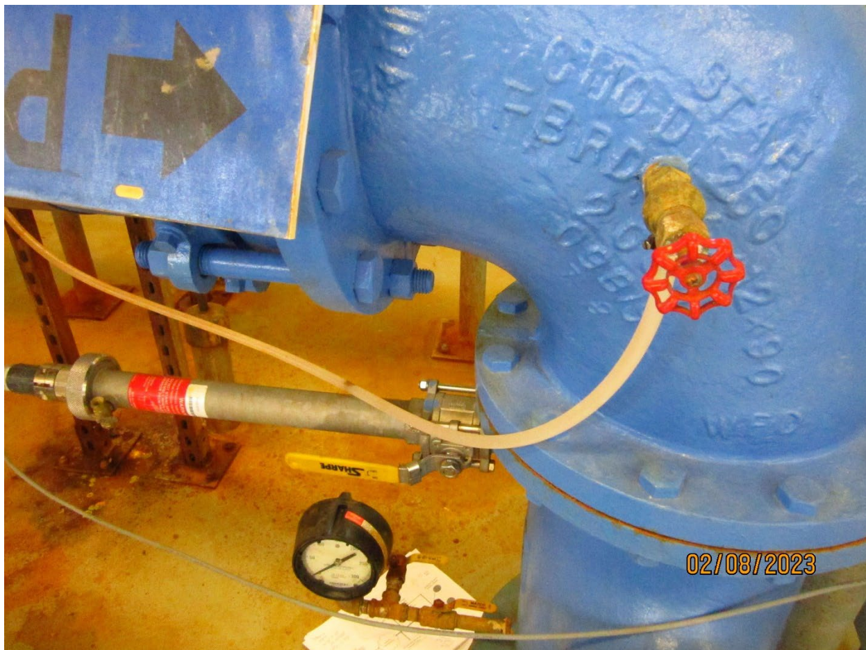
Photograph 51. Sample Tap, Treatment Room View of a finished water sample tap at the end of the treatment system. This sample point represents the water treated by Filter Nos. 1 and 2, as well as the water contributed by the raw water bypass line.
