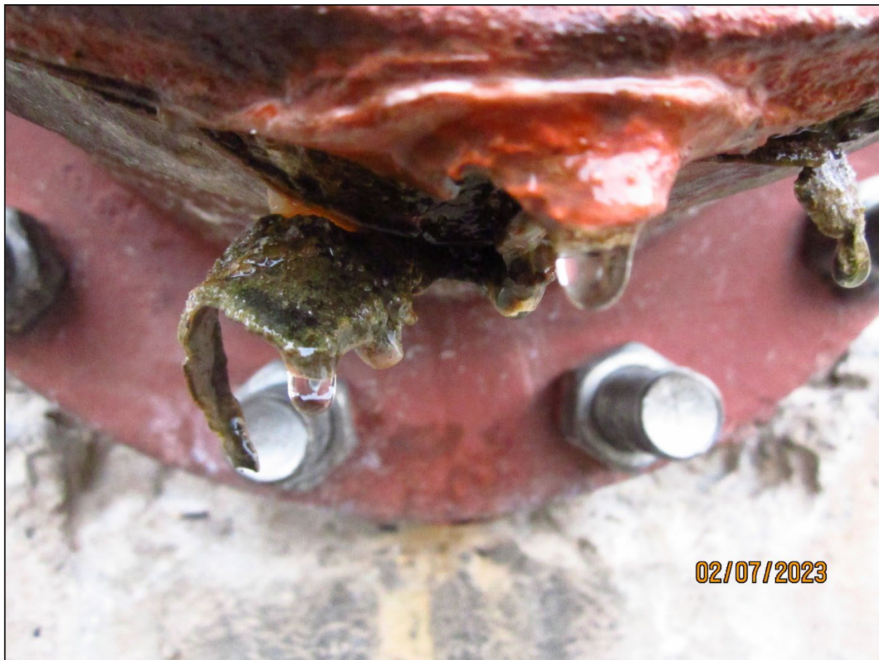
Photograph 11. W0001 Pump-to-Waste Discharge Pipe Close up view of the underside of the W0001 pump-to-waste discharge pipe. Water was dripping out of the pipe even when the flapper was closed. There appeared to be bio growth/debris attached to the bottom of the pipe.
