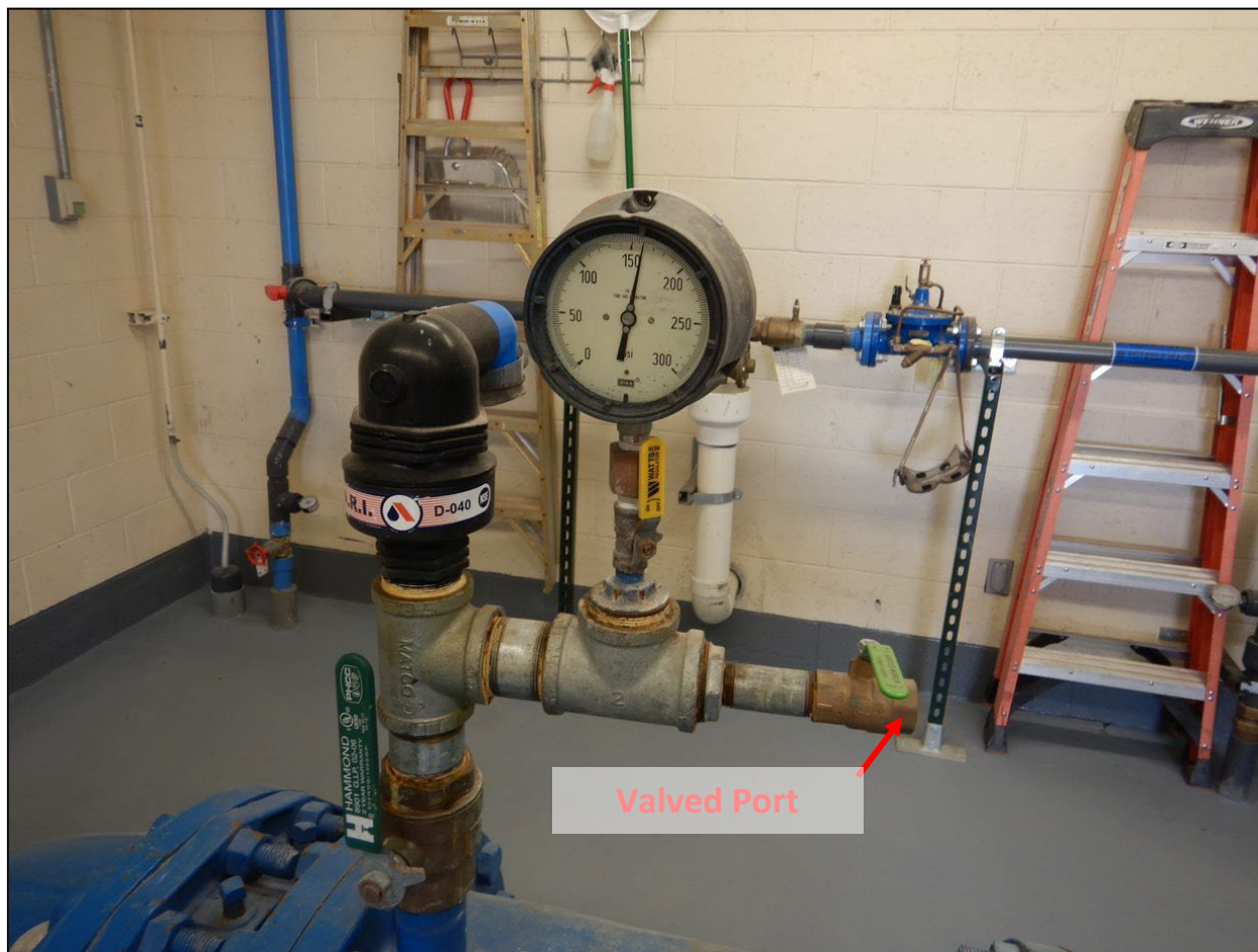
Photograph 6. Operational Valve on Air Relief Valve/Pressure Gauge Port, W0001 Line View of an air relief valve with an additional operational port with valve. The operational valve contained a pressure gauge and an open port that was unscreened and did not contain backflow prevention.
