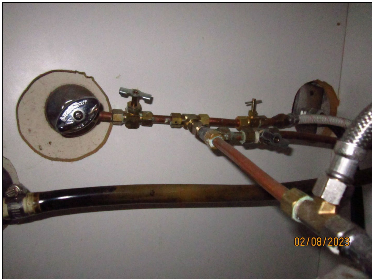
Photograph 62. "Poker Pit" LCR Sample Point, Casino View of the copper lines at the Poker Pit LCR010 sampling point at the Casino. All of the visual piping joints were copper compression joints, and no solder was observed.
