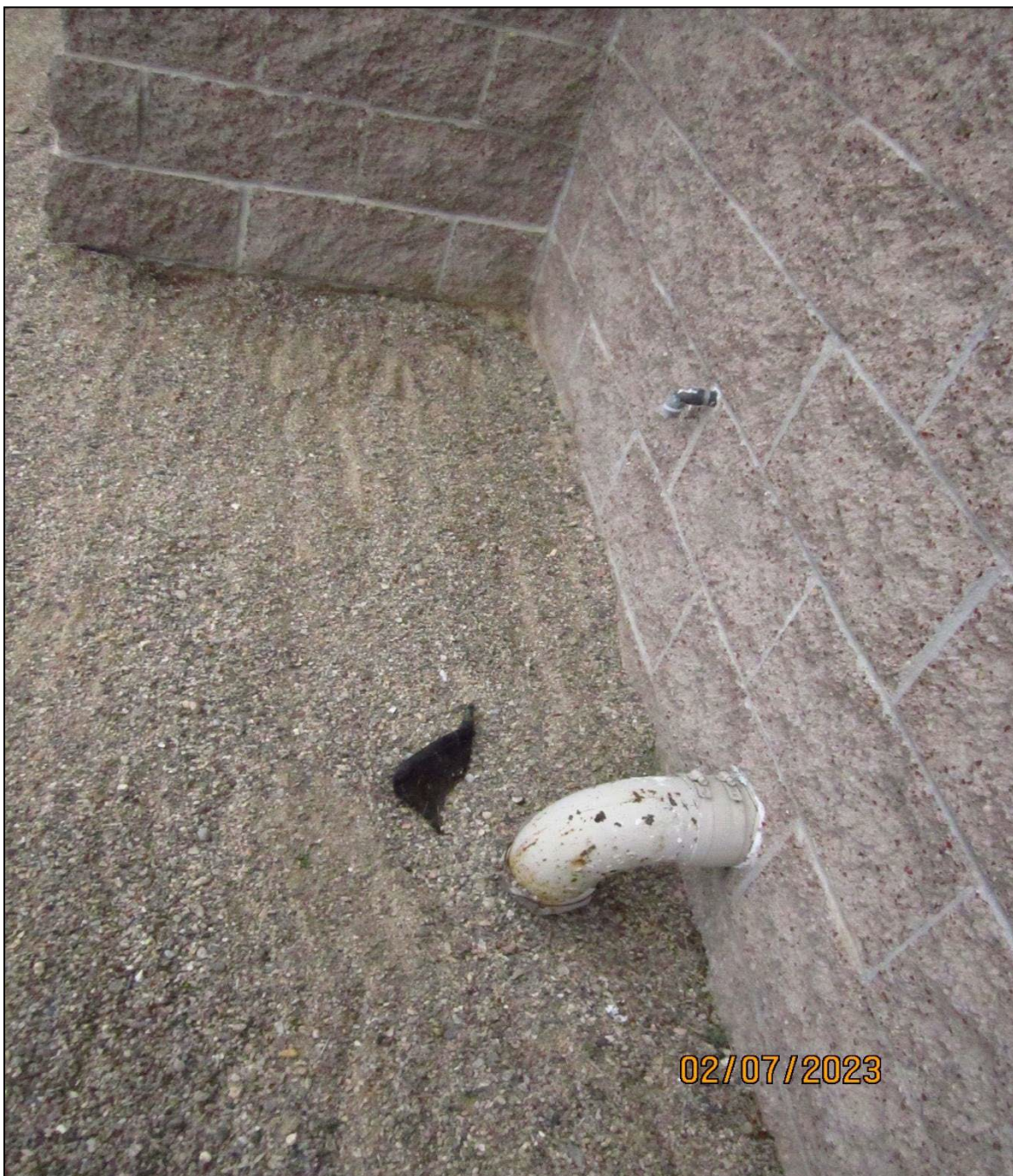
Photograph 16. Check Valve Release Pipe (W0002 Building) View of the check valve release pipe leading to the outside of the W0002 building. The opening of the pipe was screened.
