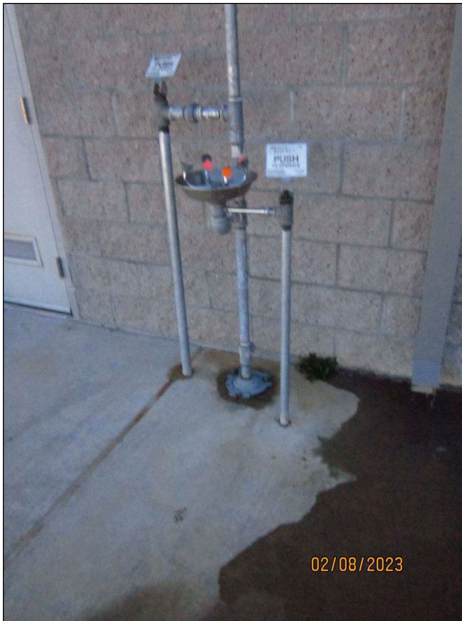
Photograph 36. Emergency Shower/Eyewash View of the emergency shower/eyewash station located between the two chemical rooms. The station was not winterized.
