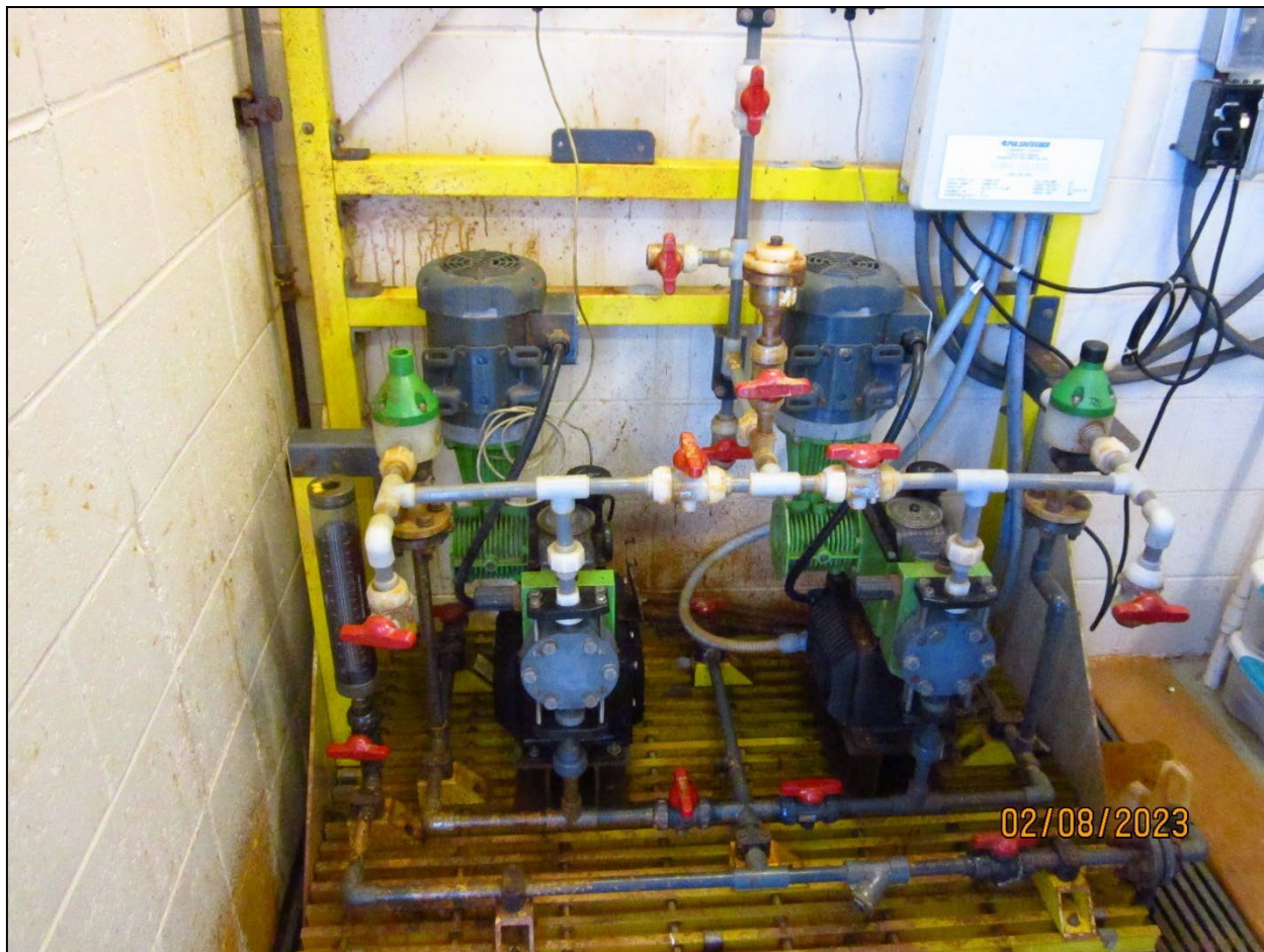
Photograph 30. Ferric Chloride Pumps/Pump Skid View of the two ferric chloride pumps in the ferric chloride room. The pumps were positioned on a skid over secondary containment. There was brown staining on the walls, pumps, and skid, indicating past spills or leaks.
