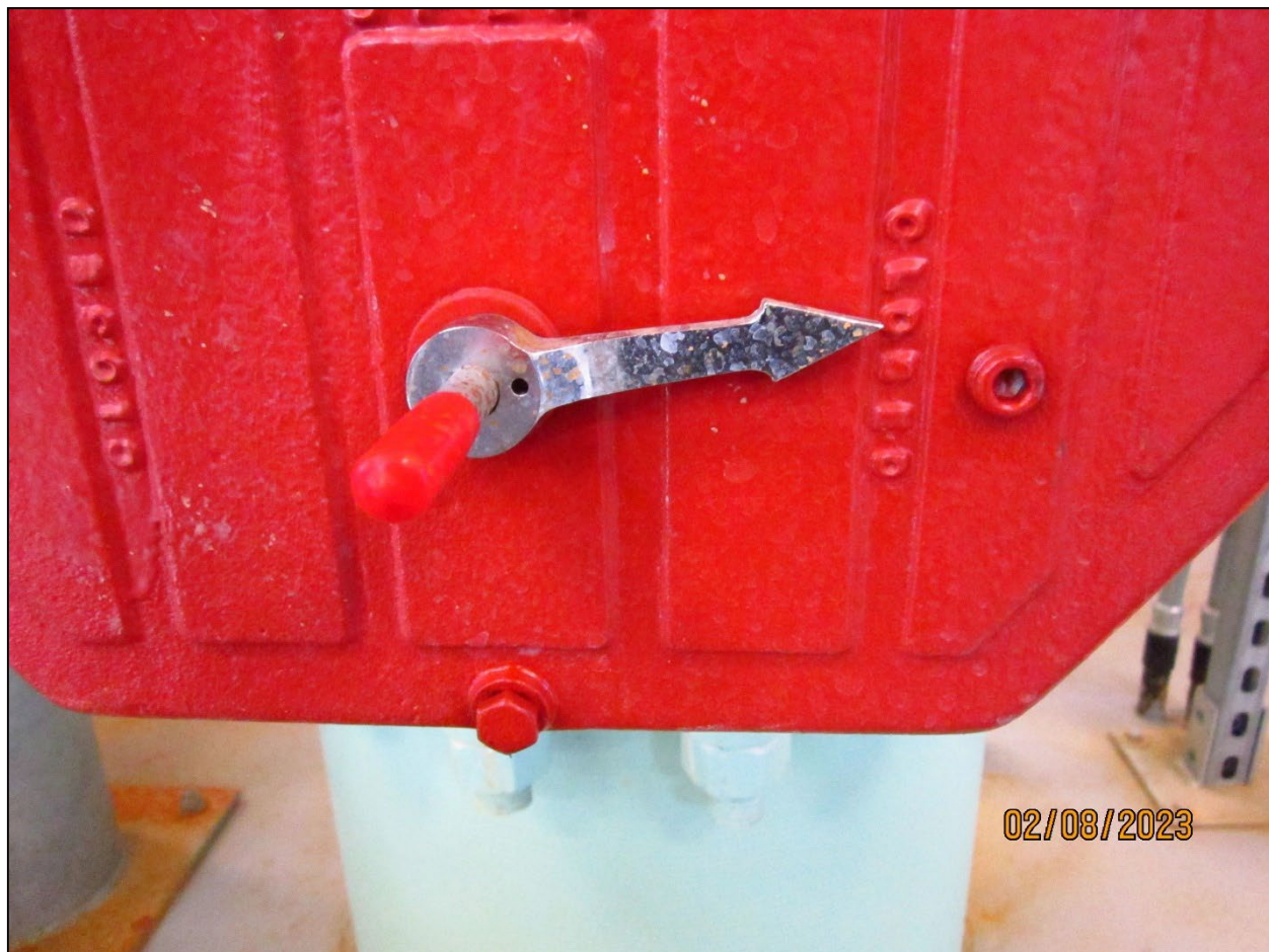
Photograph 43. Control Valve, Raw Water Influent Line Close up view of the control valve on the raw well water influent line into the treatment system. The valve was in the “closed” position.
