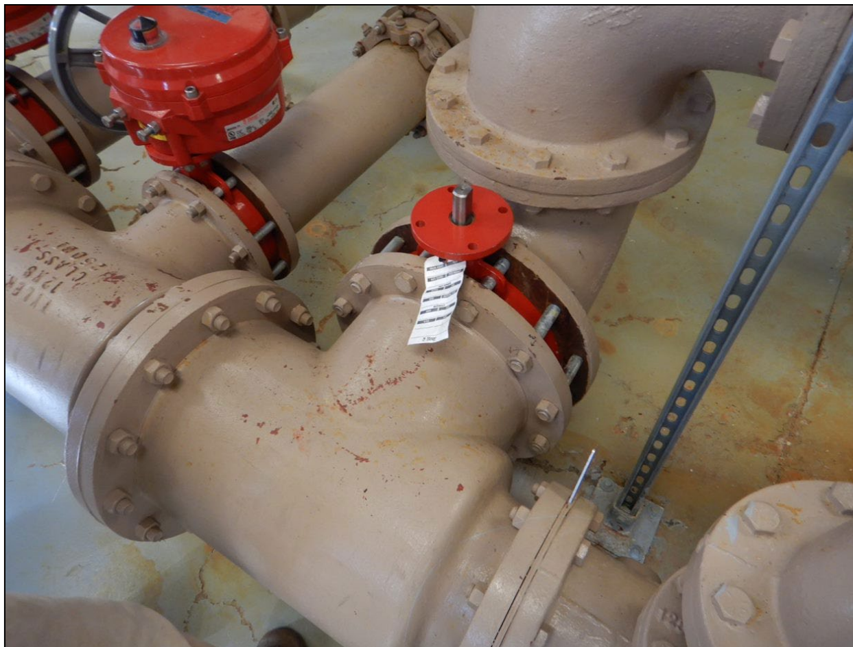
Photograph 40. Failed Effluent Valve, Treatment Room View of the failed effluent valve in the treatment room. This valve is on the filter produced water discharge main line, immediately prior to produce water blending with bypassed water and receiving final chemical treatment.
