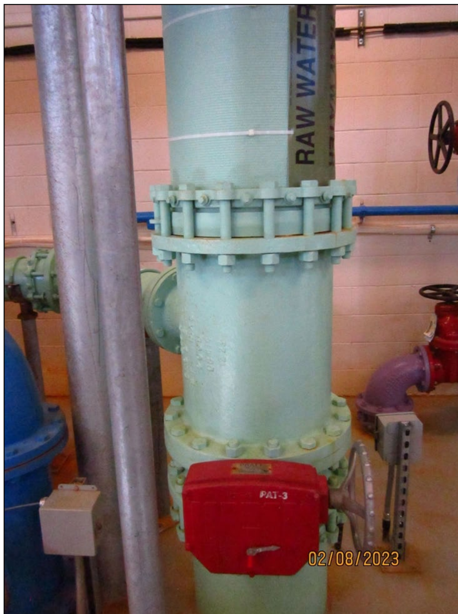
Photograph 42. Raw Water Influent Line, Treatment Room View of the raw well water influent line in the treatment room. Water enters through this line before the bypass line, filtration units, and chemical addition treatment.
