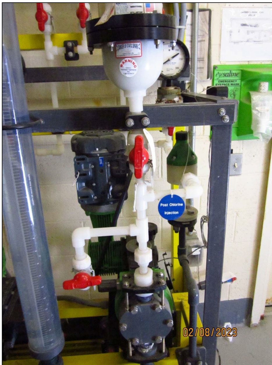
Photograph 28. Chlorine Pump, W0001 Building View of one of the two chlorine pumps associated with the ClorTec unit, located in the W0001 building. Two pumps were present, one for pre-chlorination and one for post-chlorination.
