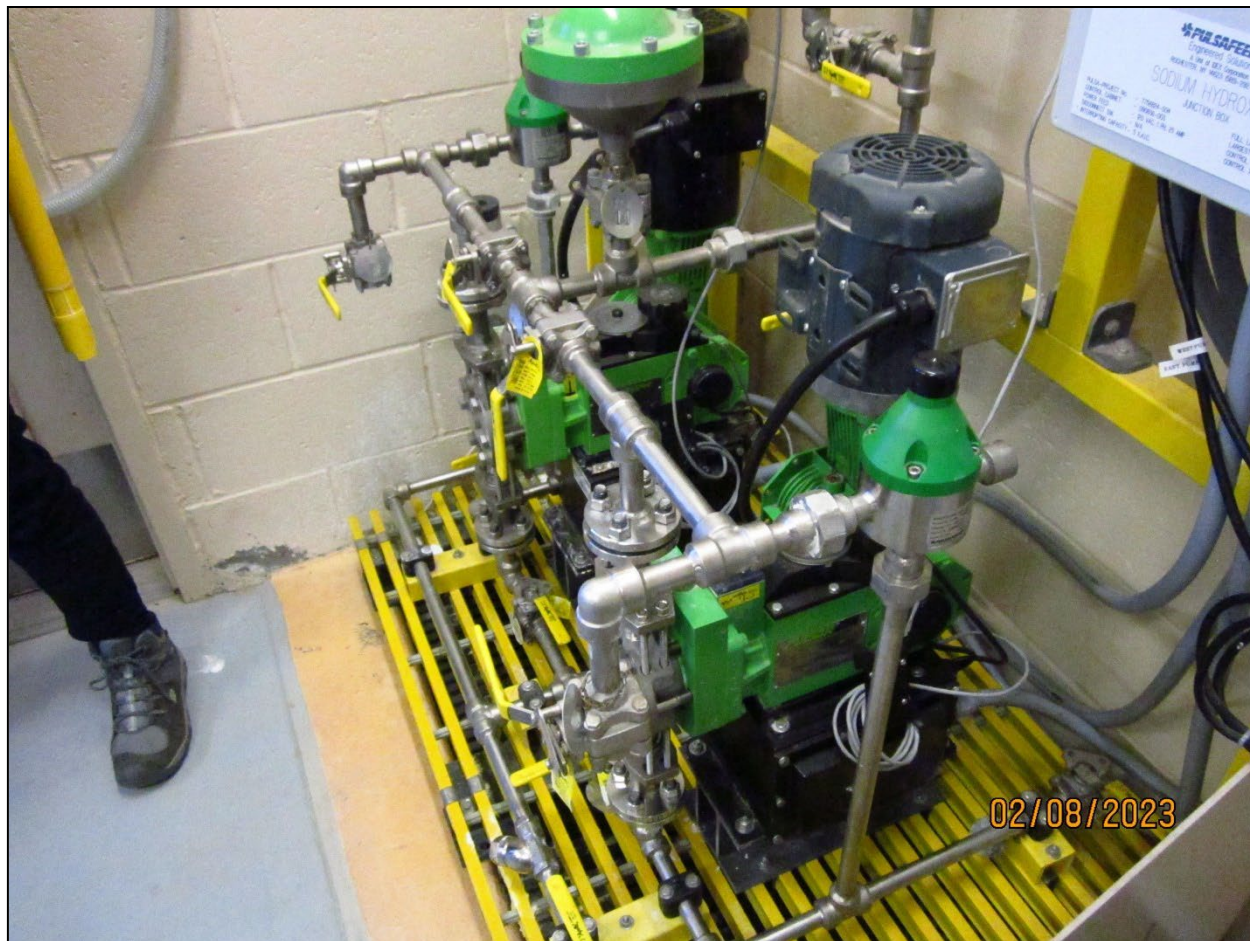
Photograph 34. Sodium Hydroxide Pumps, Sodium Hydroxide Storage/Pump Room View of the sodium hydroxide pumps in the room. The pumps were positioned on a pump skid over secondary containment. There did not appear to be signs of spills/leaks.
