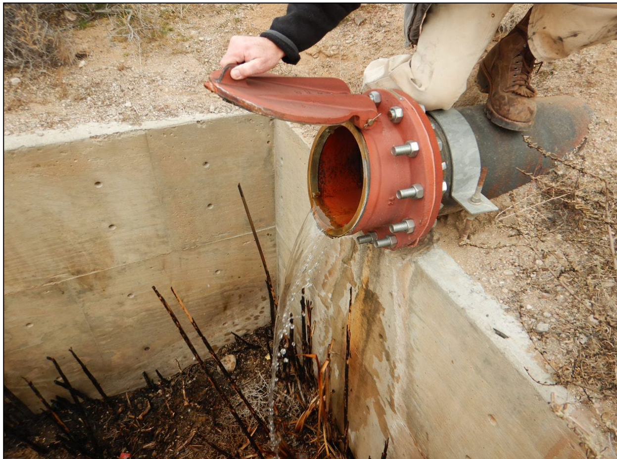
Photograph 10. W0001 Pump-to-Waste Discharge Pipe View of the open flapper on the discharge port west of the W0001 building. Water was continuously flowing out of the pipe when the flapper was open. There was approximately one inch of water in the pipe, and we observed a flow of approximately 3-4 gallons per minute.
