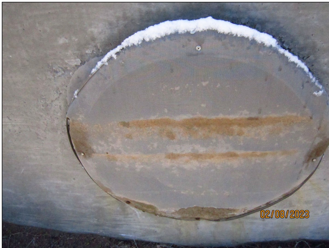
Photograph 61. ST001 Tank Overflow Outfall Close up view of the overflow outfall pipe screen. There was mud/dirt at the bottom of the screen, and there appeared to be four different water mark levels on the screen.
