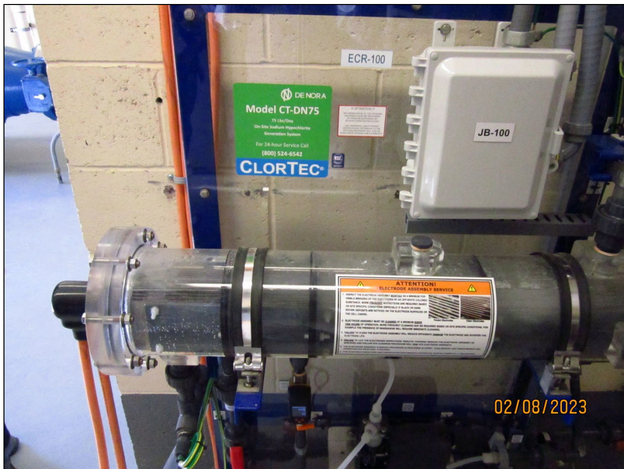
Photograph 27. ClorTec Unit, W0001 Building View of the ClorTec unit, located in the W0001 building. The unit converts brine to a hypochlorite solution used for disinfection of raw and produced water.
