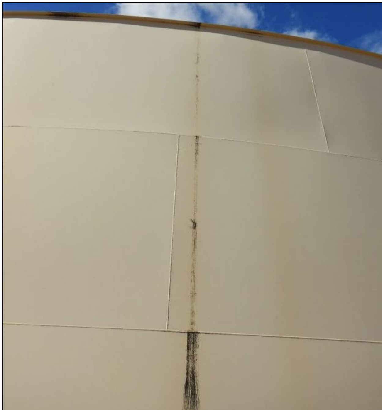
Photograph 56. Sandia Casino Tank (ST001) View of the side of the ST001 tank. The tank had spots where it appeared that water on top of the tank ran off causing algal growth.
