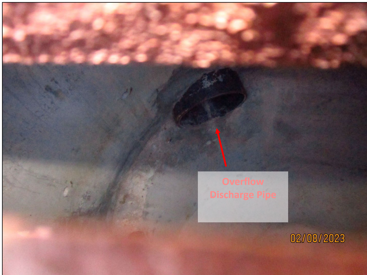
Photograph 58. Underground ST001 Overflow Pipe Discharge View of the ST001 overflow pipe discharge point below grade into the drainage basin. The opening of the overflow pipe was unscreened.
