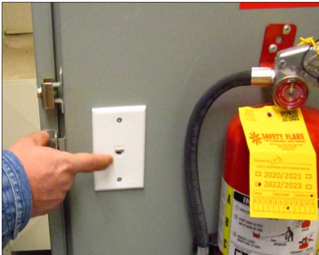
Photograph 26. Communications Jack, W0002 Building View of a newly installed communications jack so that a laptop computer could be used to observe and control W0002 operations.
