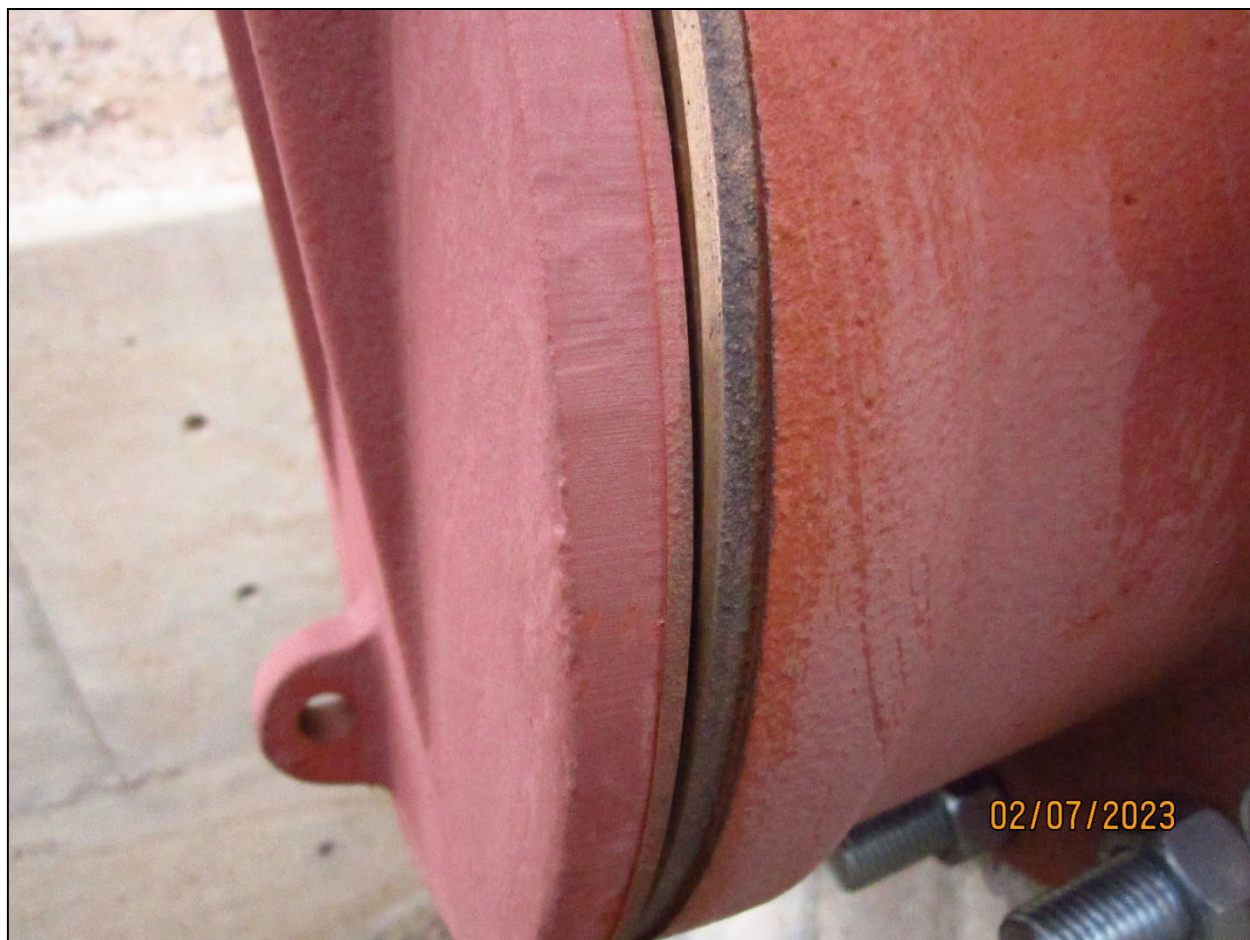
Photograph 20. W0002 Pump-to-Waste Discharge Pipe Opening (Flapper) Close up view of the W0002 discharge flapper that had a tight seal with no space for insect or debris entry.
