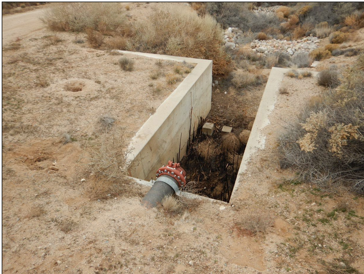
Photograph 9. W0001 Pump-to-Waste Discharge Pipe View of the pump-to-waste discharge pipe and outfall area west of the W0001 building. There appeared to be cattails growing in the discharge basin, and the ground was wet. It appeared that the cattails had been recently burned. Water was dripping from the pipe, even with the flapper valve in the closed position.
