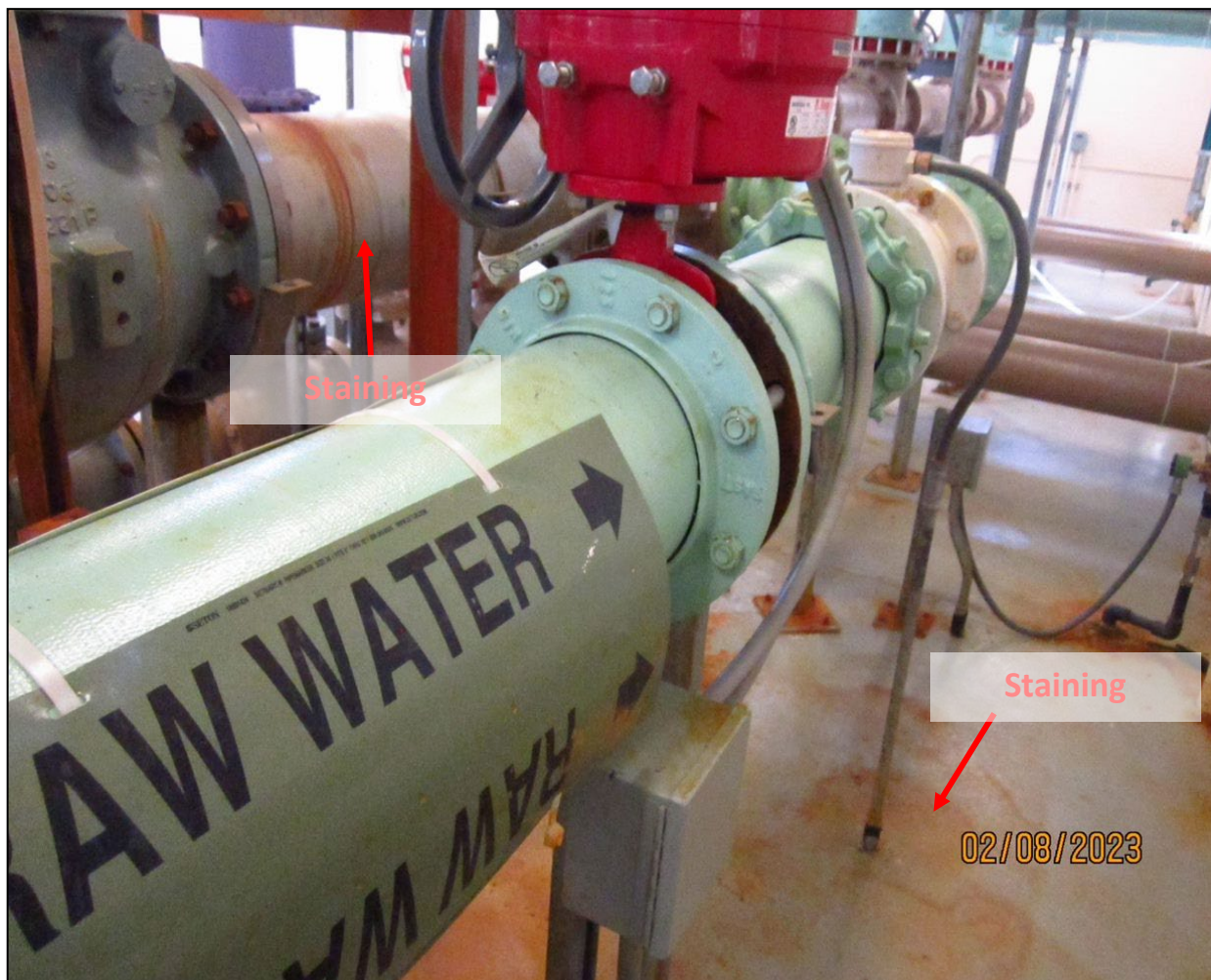
Photograph 46. Raw Water Pipe, Treatment Room View of the raw water bypass pipe in the treatment room. This pipe runs beneath the ferric chloride injection point, and there was evidence of brown staining and corrosion on the floor, piping, and nuts and bolts, possibly indicative of a ferric chloride spill.
