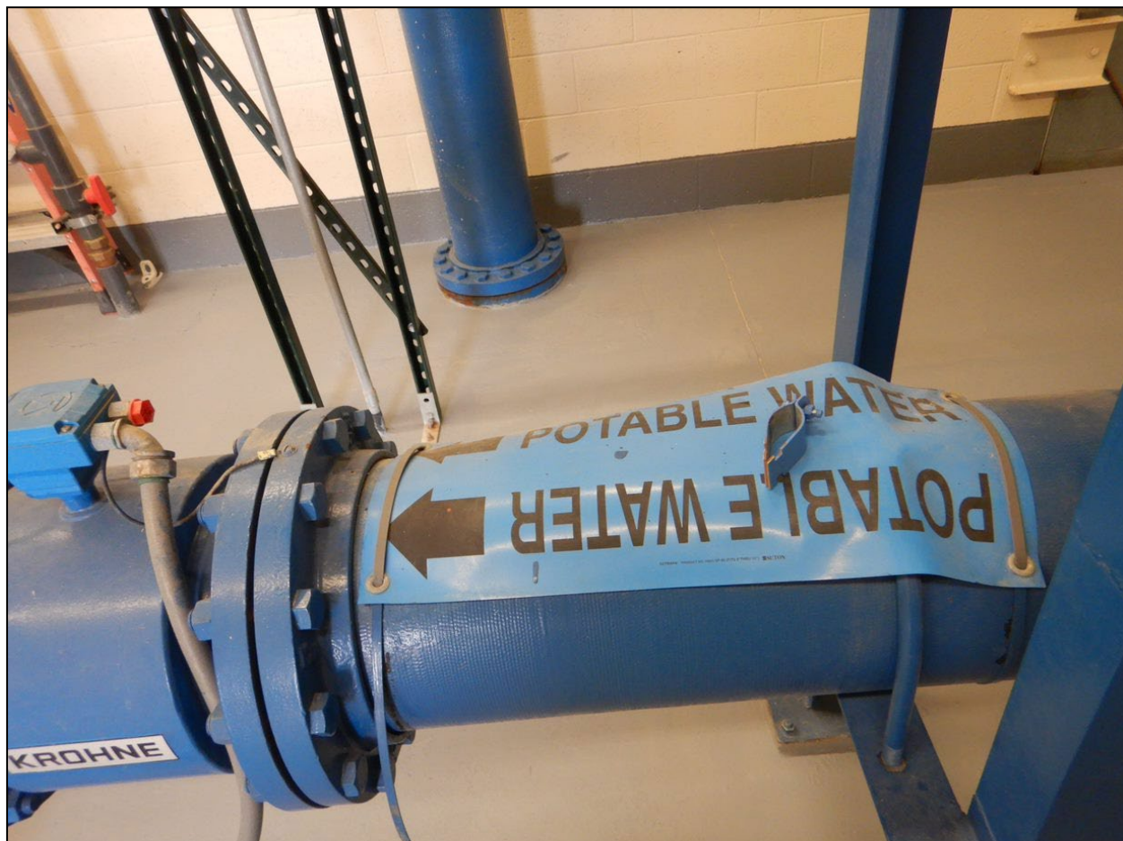
Photograph 7. Incorrect Sign W0001 Line View of a sign that read “potable water” on the W0001 pump line. This line actually conveys raw well water from Casino Well No. 1 to the connection with the raw water from Casino Well No. 2 and then to the water treatment system. The sign was removed after the operator was asked to confirm the raw water flow route.
