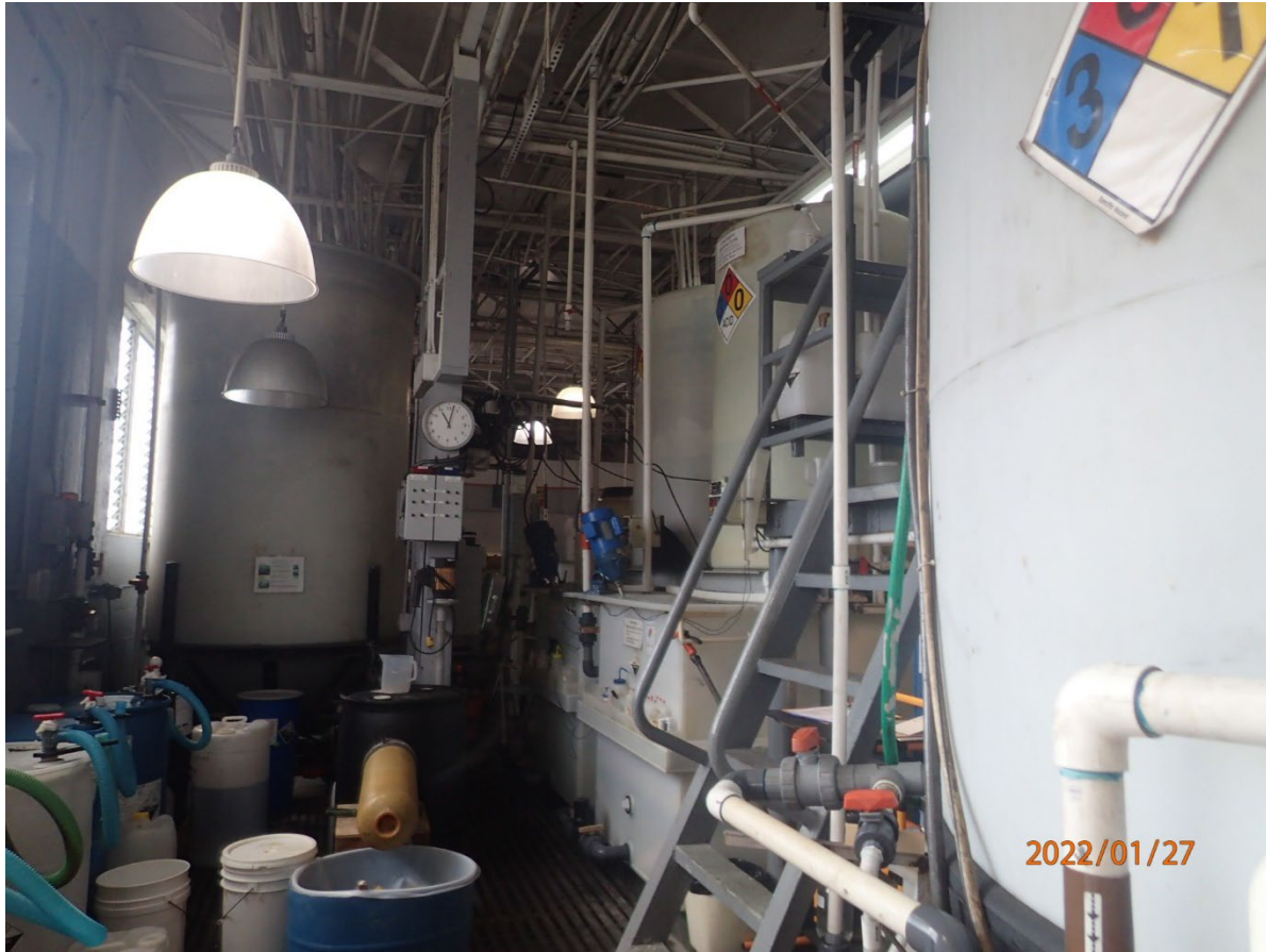
Photo 2: Wastewater Pre-treatment Plant.
