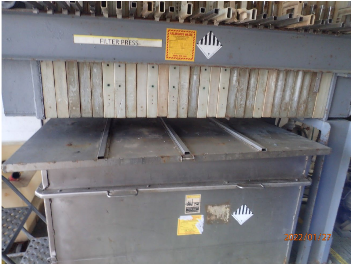
Photo 3: Dewatered F006 filter cake is collected beneath the filter press in an open-top metal 5'x4'x4' container. CAA1.
