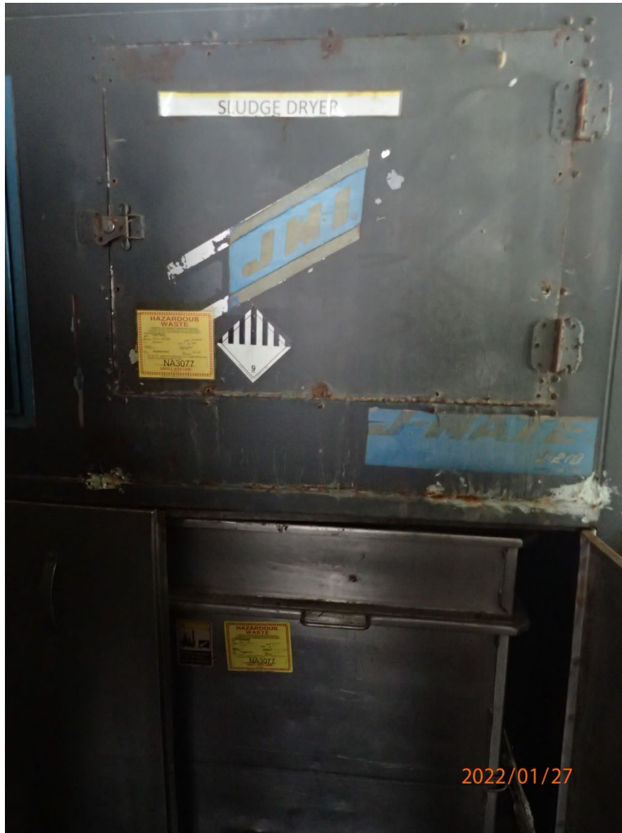
Photo 4: Electrically heated sludge dryer: JWIJ-MATE J-210. CAA1.
