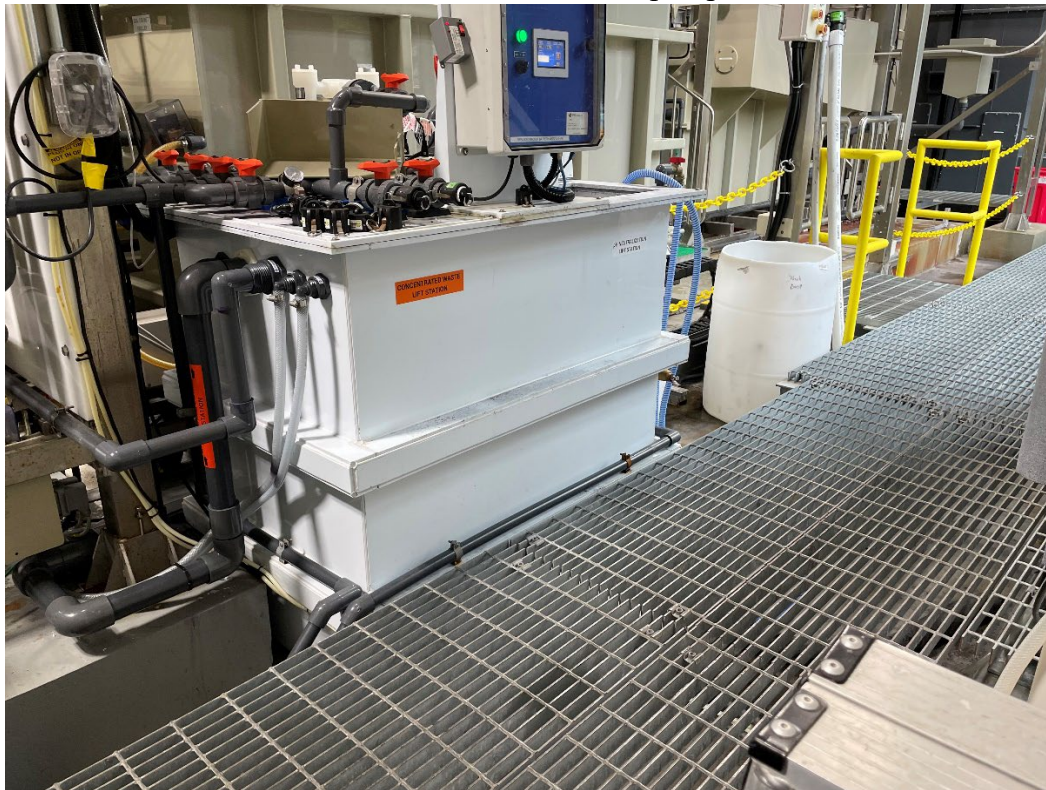
Photo #4. Process waste streams from the rinse baths are pumped to the master lift station.
