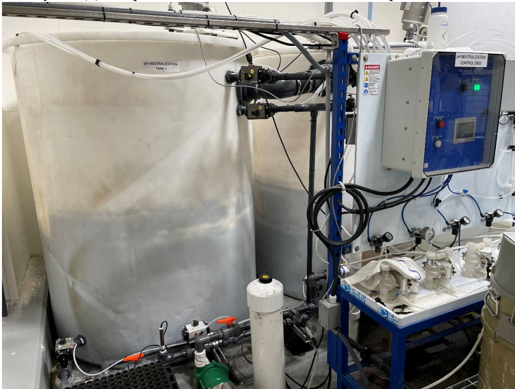
Photo #5. Only one (1) of 2 pH Neutralization Tanks is used to treat process wastewater.
