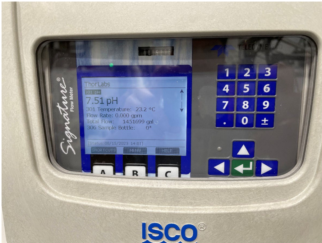
Photo #2. No calibration stick was observed on the flow meter/recorder.
