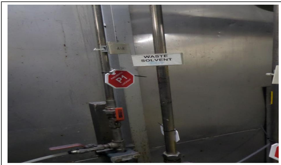
Hyundai. Kettle Purge Line # Area. Inspectors observed red octagonal shaped lockout tags and yellow diamond shaped tags designated with the letters C, P, E or RC and followed by a number (1, 2, or 3) secured by plastic cable ties to the tanks and the tank's ancillary equipment (valves, pumps, flanges, connectors, electrical and pneumatic equipment). Photograph 15 taken July 26, 2021 at 3:50 p.m.
