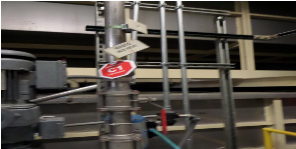
Hyundai. Kettle Purge Line 1 Area. Inspectors observed red octagonal shaped lockout tags and yellow diamond shaped tags designated with the letters C, P, E or RC and followed by a number (1, 2, or 3) secured by plastic cable ties to the tanks and the tank's ancillary equipment (valves, pumps, flanges, connectors, electrical and pneumatic equipment). Photograph 11 taken July 26, 2021 at 3:44 p.m.
