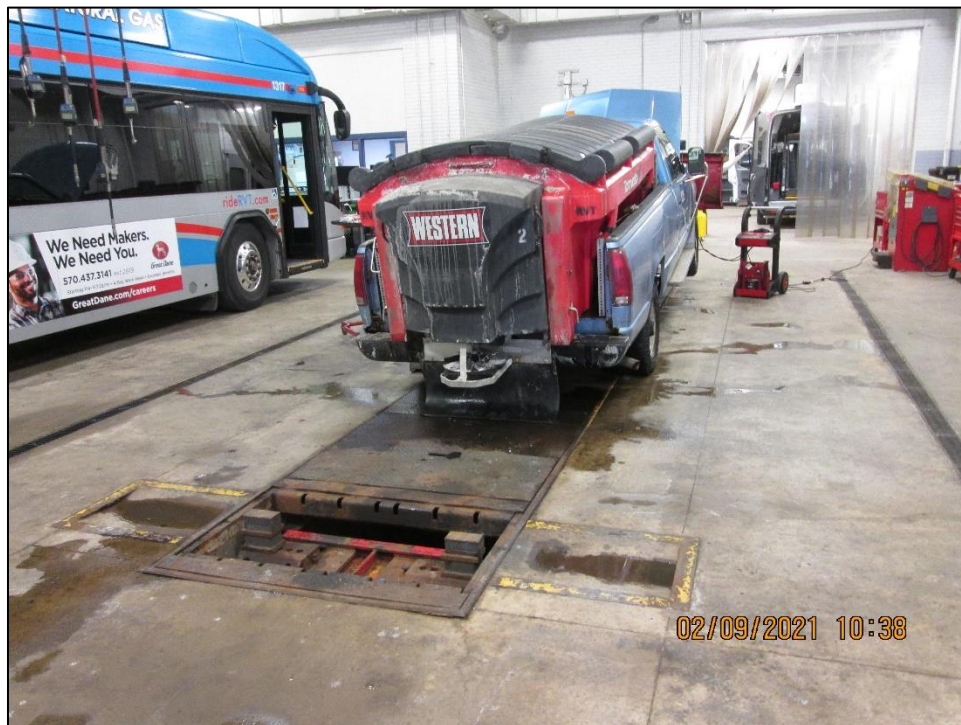
Photograph 16. View of a maintenance area inside the bus maintenance building. City representatives stated that the floor drains flow to an oil/water separator.
