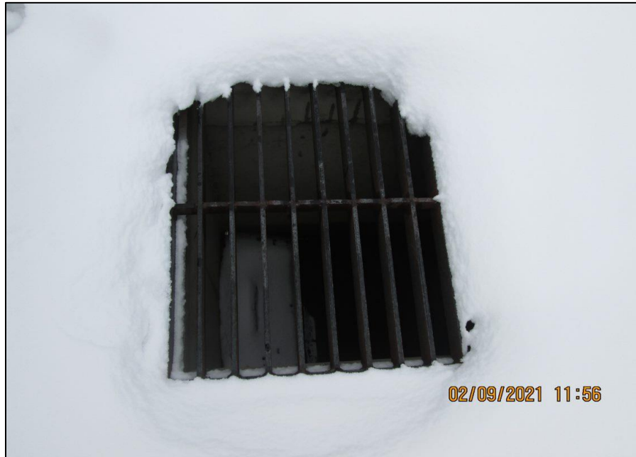
Photograph 27. View of the SMP storm drain located in the middle portion of the Grey Fox Rentals parking lot.
