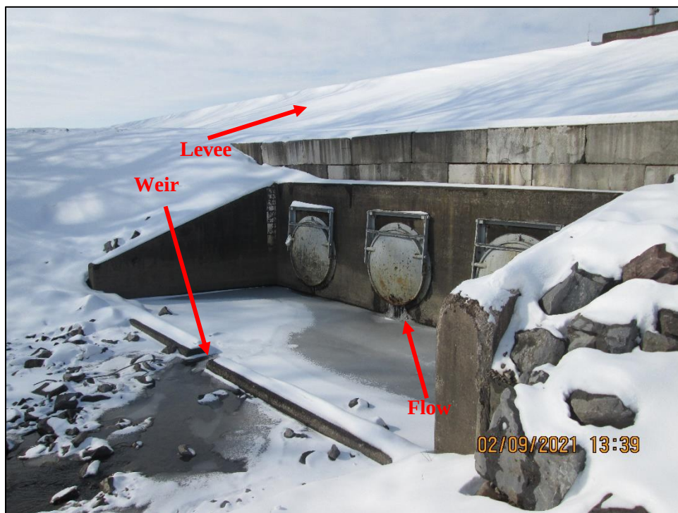
Photograph 39. View, facing northwest, of the Outfall WB01 headwall. The EPA Inspection Team observed three pipe flap gates with flow from the central pipe.
