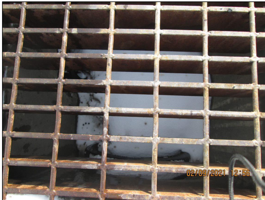
Photograph 32. Closer view inside the storm drain from Photograph 31. Note the presence of snow in the bottom of the drain.
