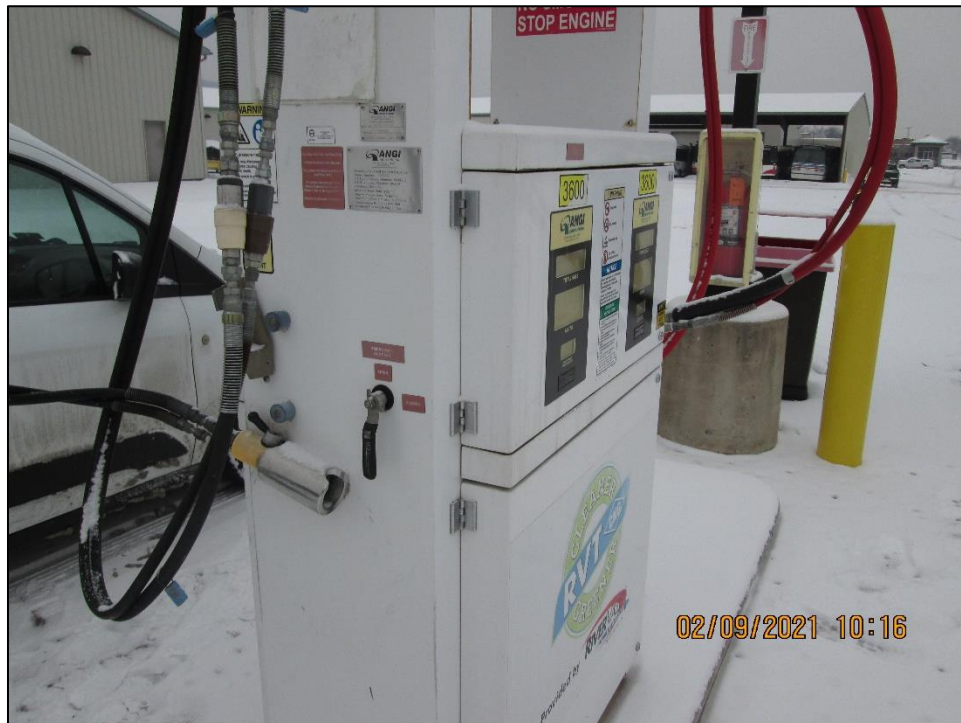
Photograph 9. View, facing east, of a public access compressed natural gas fueling station located near the southwest corner of the Municipal Complex.
