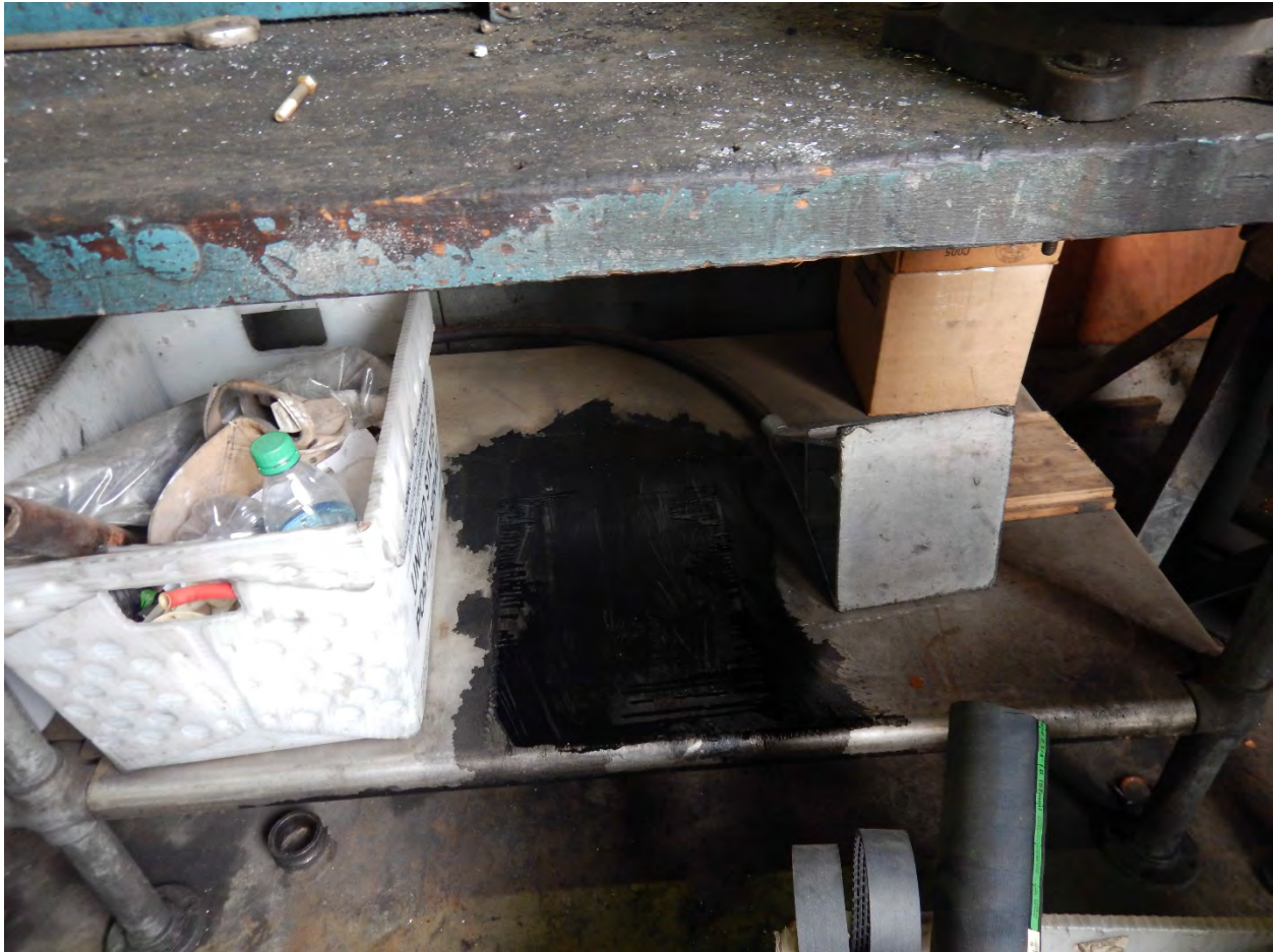
# 238 – Used Oil Spill
