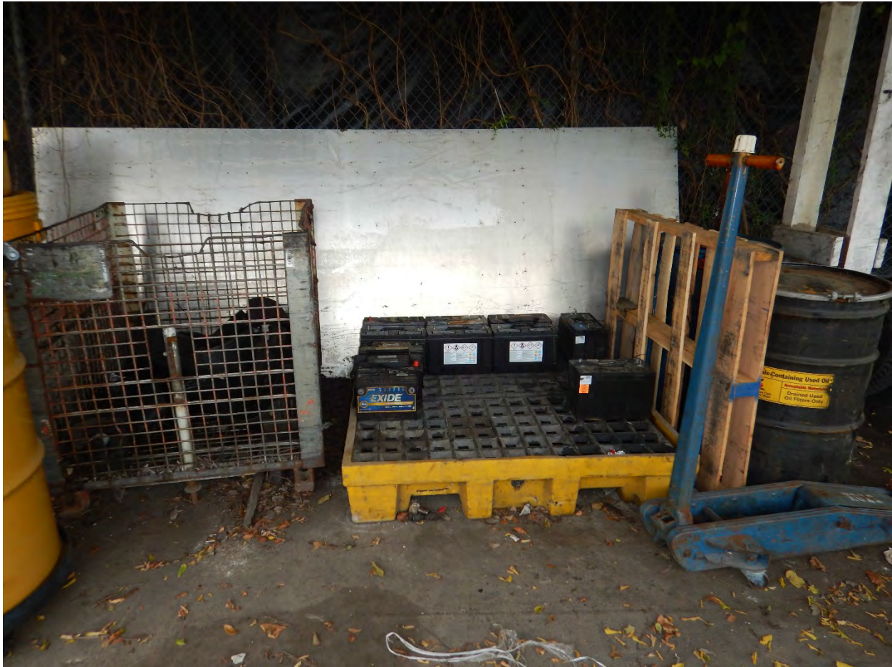
# 254 – Underground Storage area – Used Batteries not labeled
