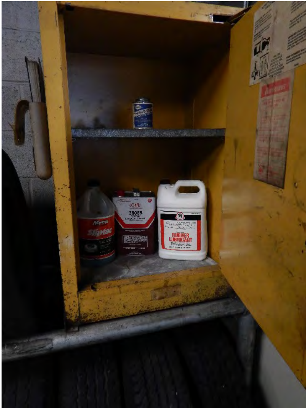
# 207- Storage of materials in flame proof locker
