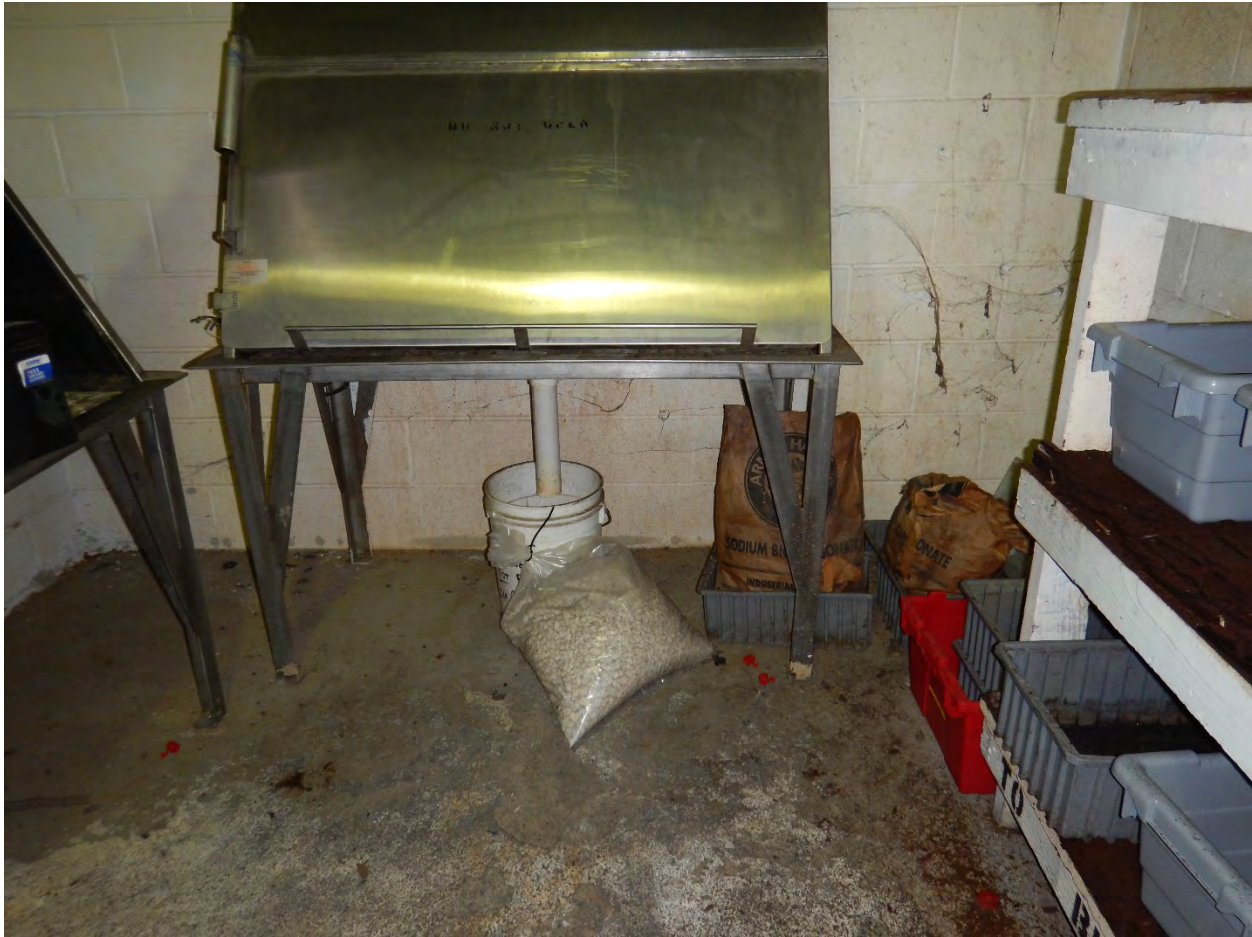
#213 – Bags of Sodium Bicarbonate in Battery Room
