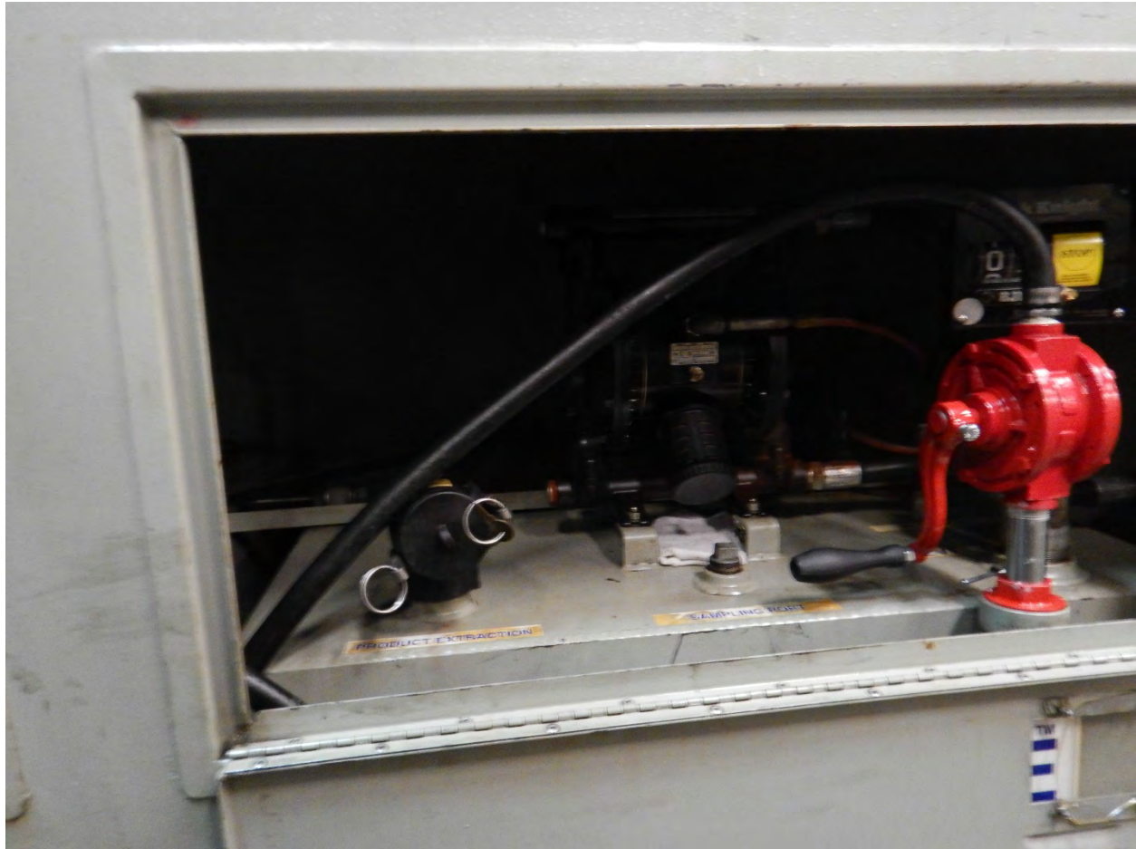
# 279 – Waste Pump – AntiFreeze
