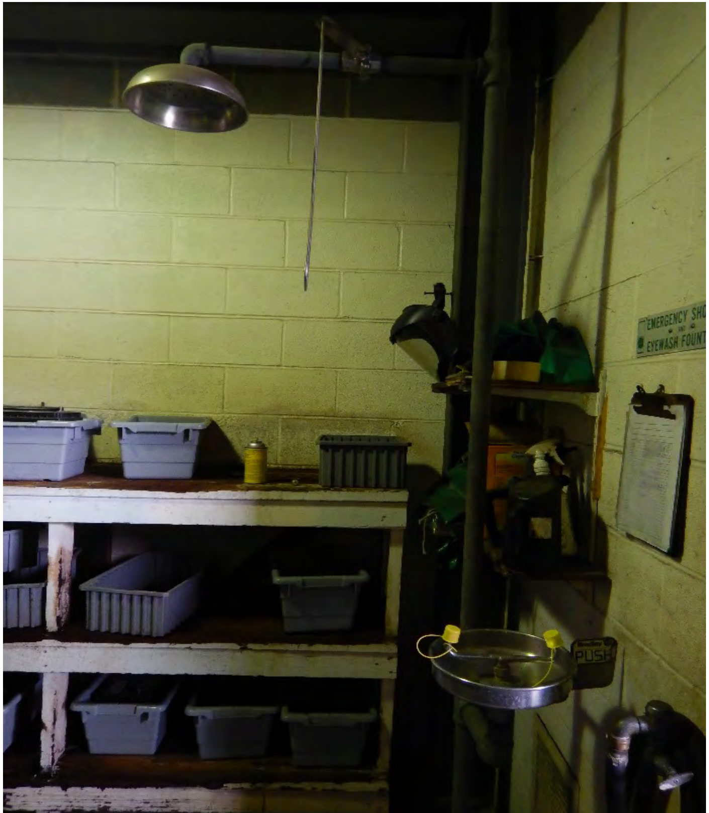
#210 – Eye Wash / Shower Station
