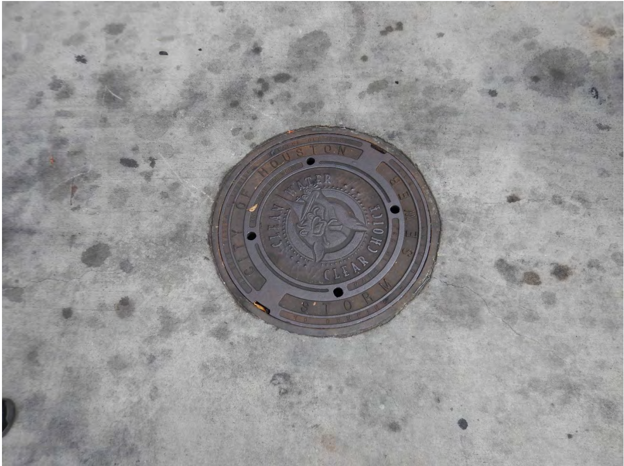
# 252 – Underground Storage Tank Cover
