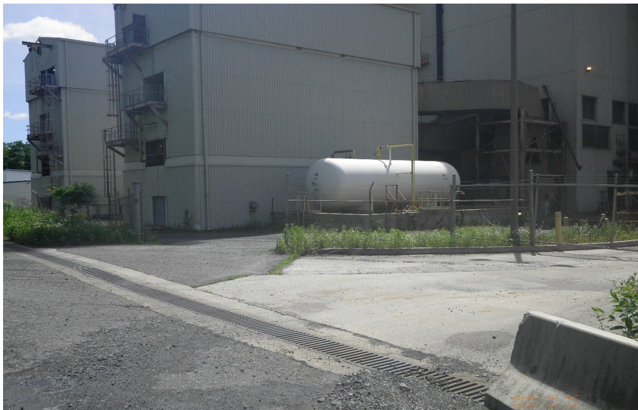
5. Ammonia Tank for Injection into Boilers for NOx Control – Panther Creek Generating – 6/8/22
