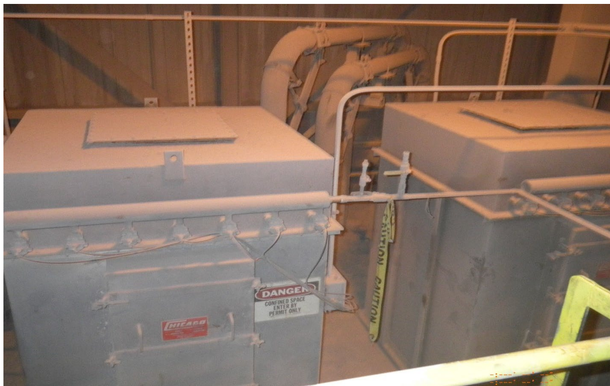
9. Two Limestone Pulverizer Dust Collectors – Panther Creek Generating – 6/8/22
