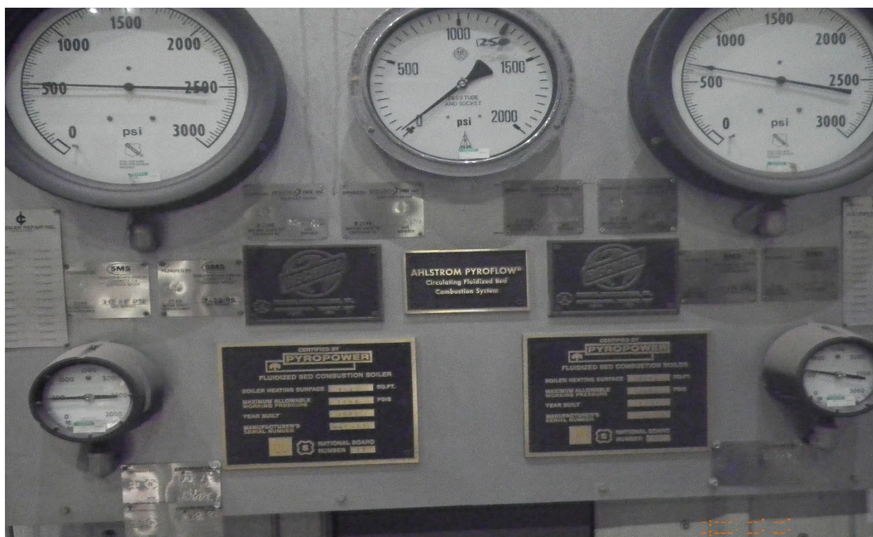
12. Boiler 1 and Boiler 2 Nameplates – Panther Creek Generating – 6/8/22
