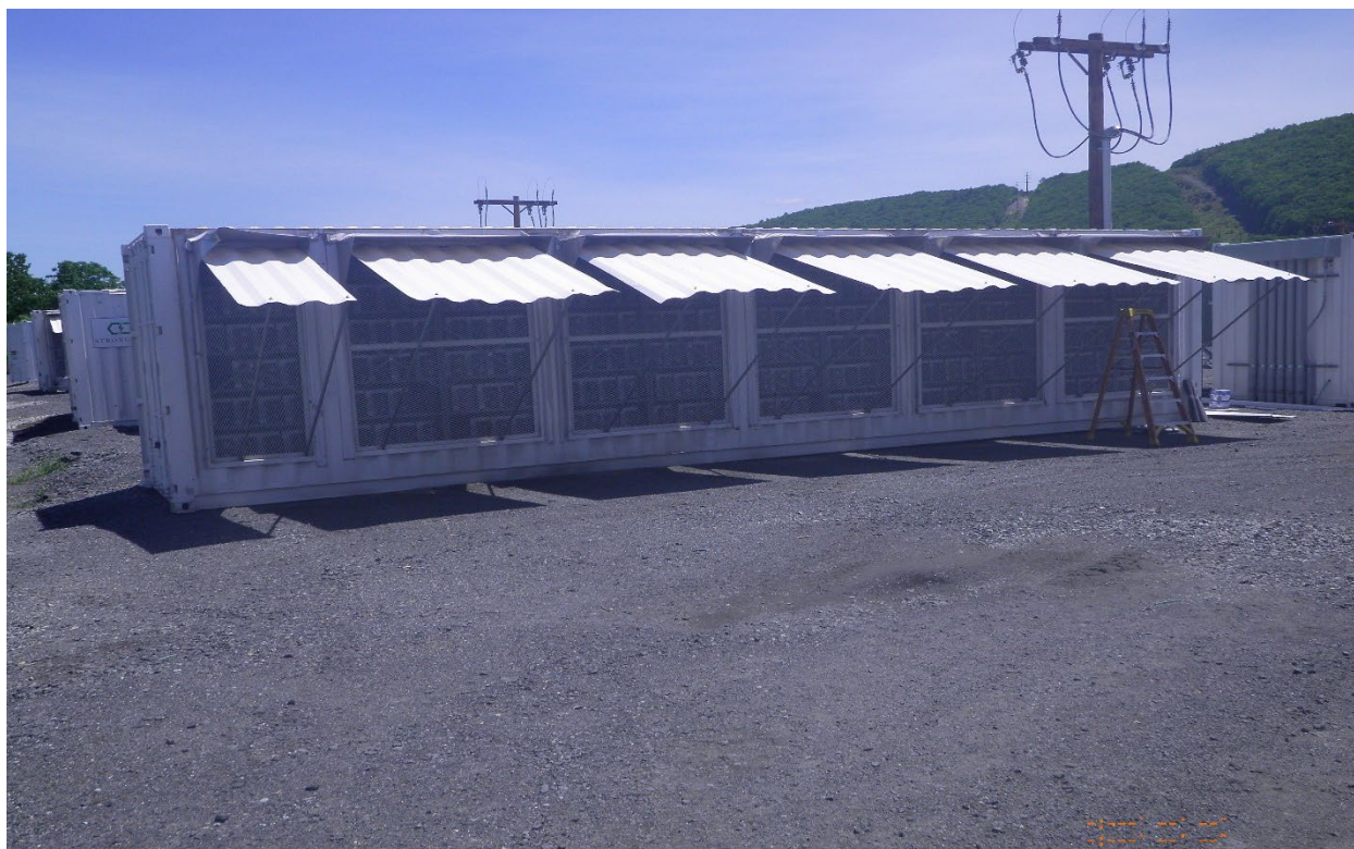
18. Outside View of Storage Container at Data Center – Panther Creek Generating – 6/8/22
