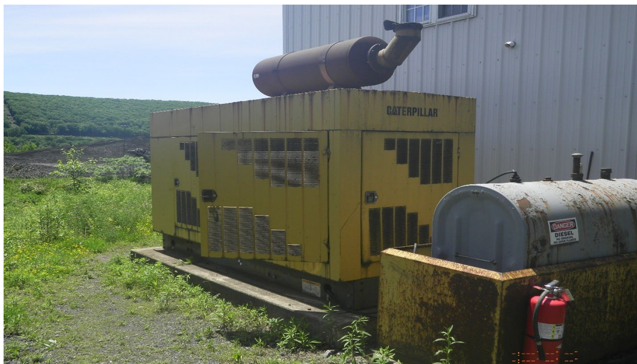
20. Outside View of Caterpillar Emergency Generator and Fuel Tank – PantherCreek Generating – 6/7/22
