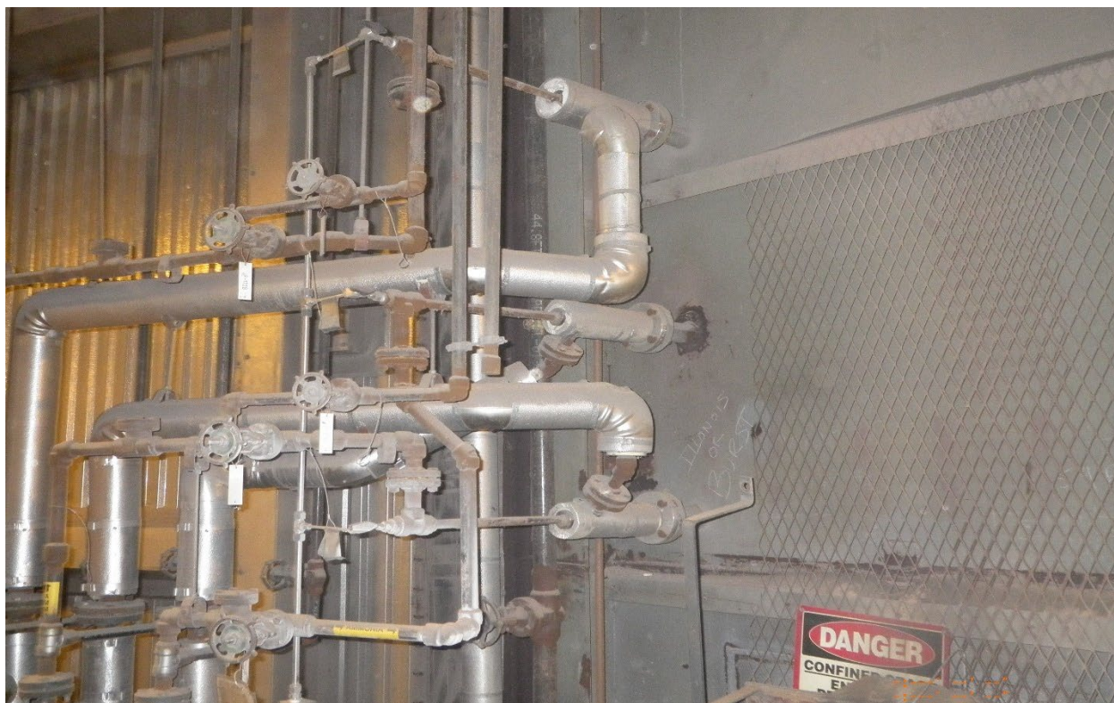
7. Ammonia Injection Ports – Panther Creek Generating – 6/8/22
