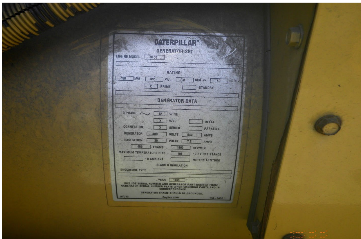
19. Caterpillar Emergency Generator Nameplate – Panther Creek Generating – 6/8/22
