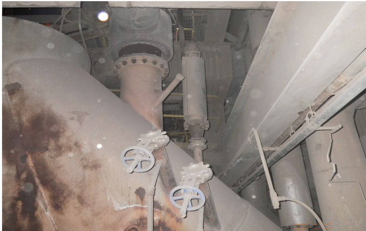
10. Coal And Limestone Injection Boiler 2 – Panther Creek Generating – 6/8/22
