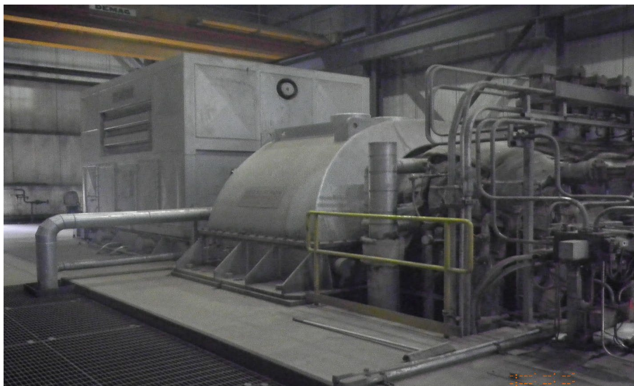
13. Steam Turbine – Panther Creek Generating – 6/8/22
