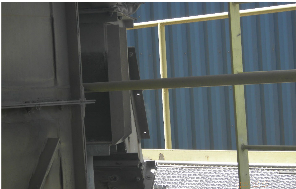
8. Fugitive Emission Point from Bucket Elevator – Panther Creek Generating – 6/8/22
