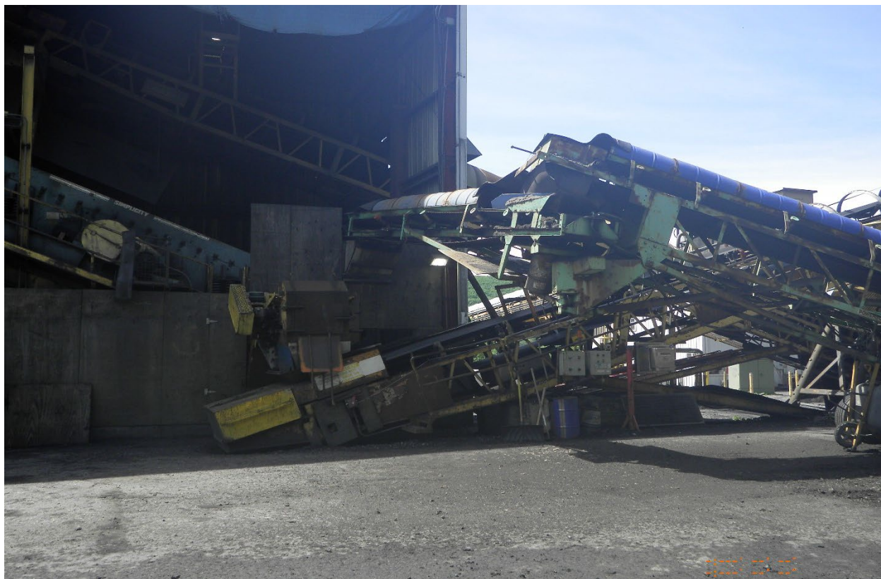
3. Conveyor from Coal Pile to Crusher Building – Panther Creek Generating – 6/8/22
