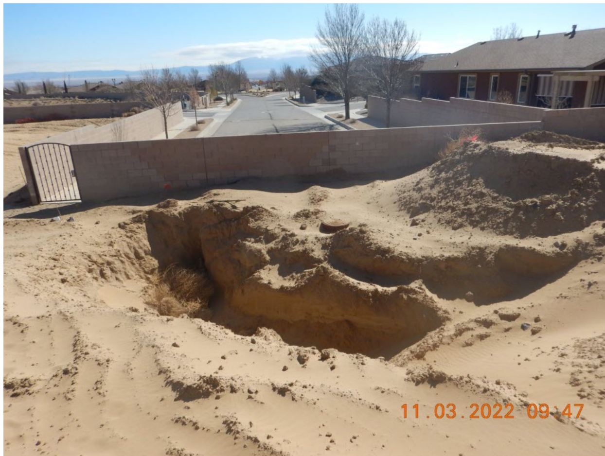
View of unstabilized excavation and embankment located along eastern side of development. (DSCN2151). Note: The Jubilee subdivision is in the upper portion of the photograph. Photographed by D. Esparza
