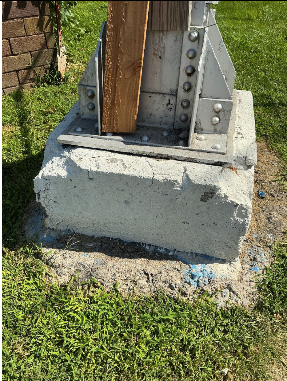
Deterioration of the concrete foundation supporting one of the legs of the 75,000-gallon Cone Tower.
