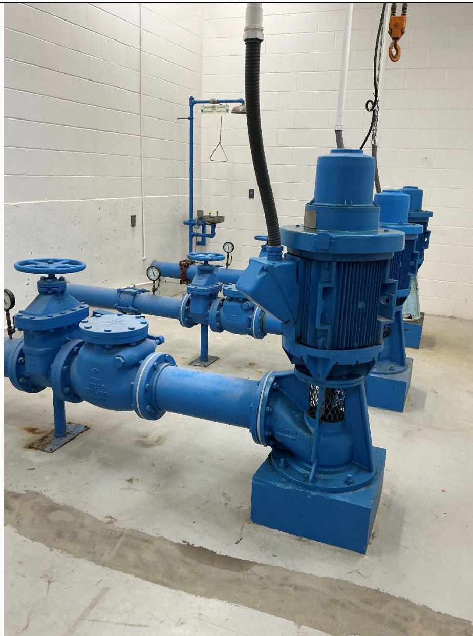
WTP high service pumps.
