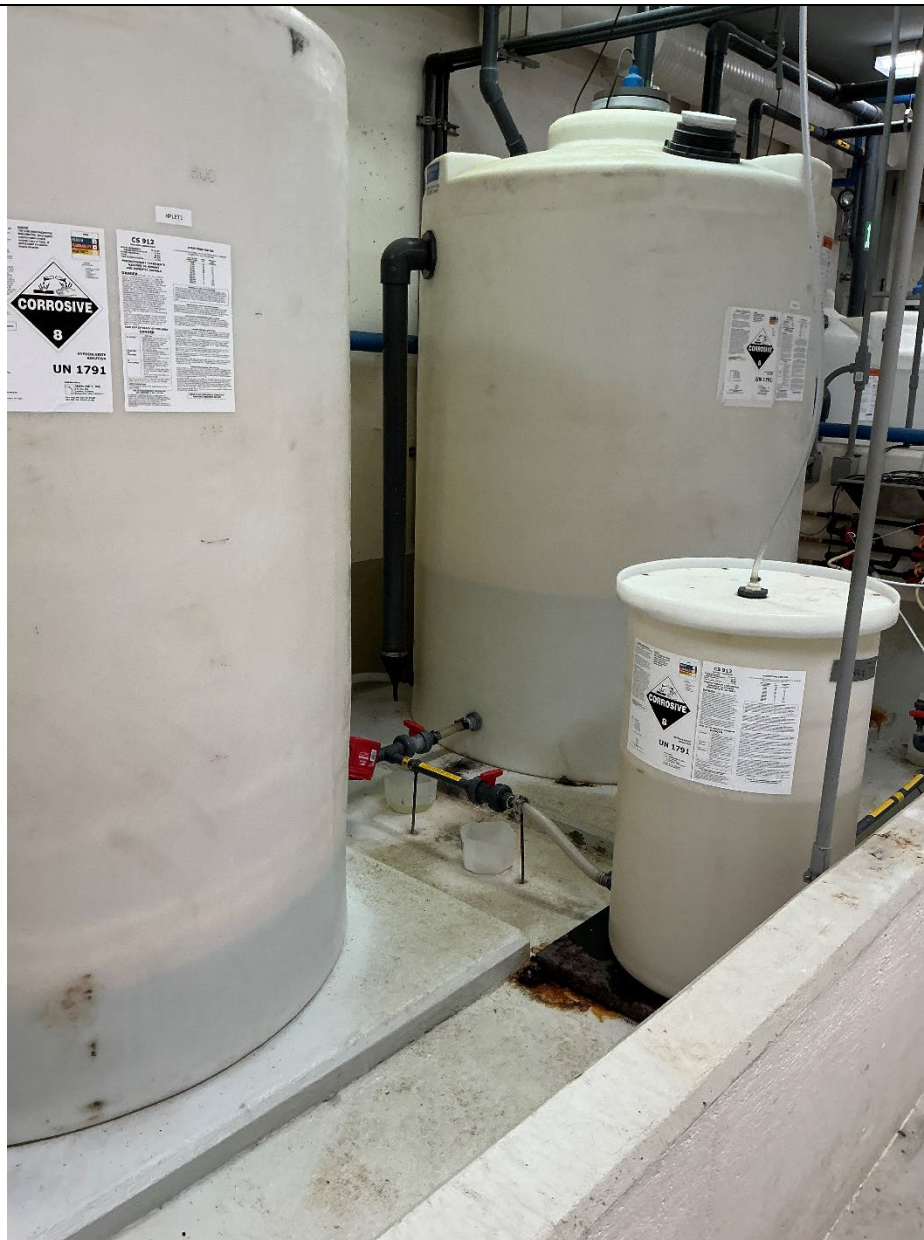
Coagulants with secondary containment.
