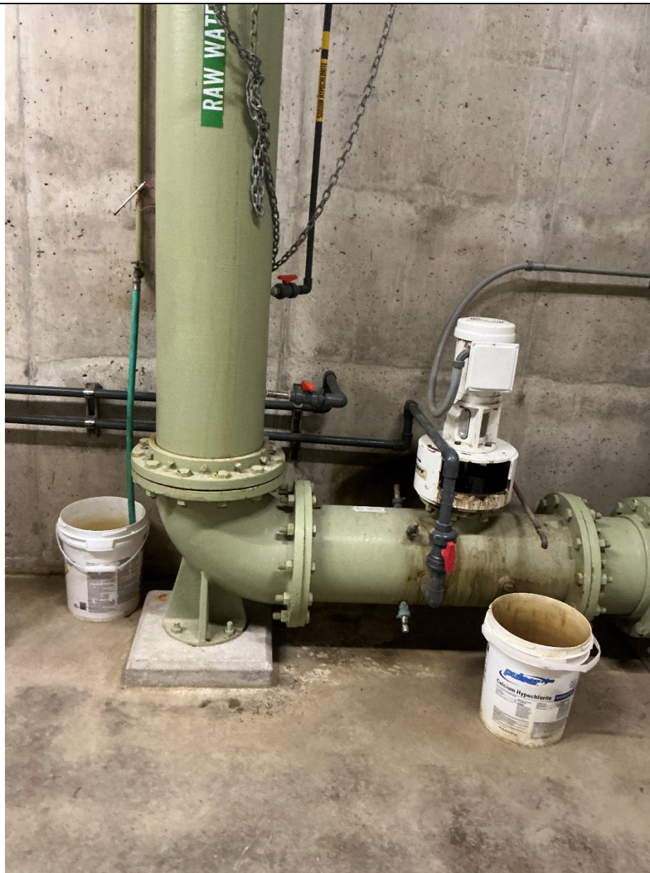
Water Treatment Plant raw water entry point and first sampling location.
