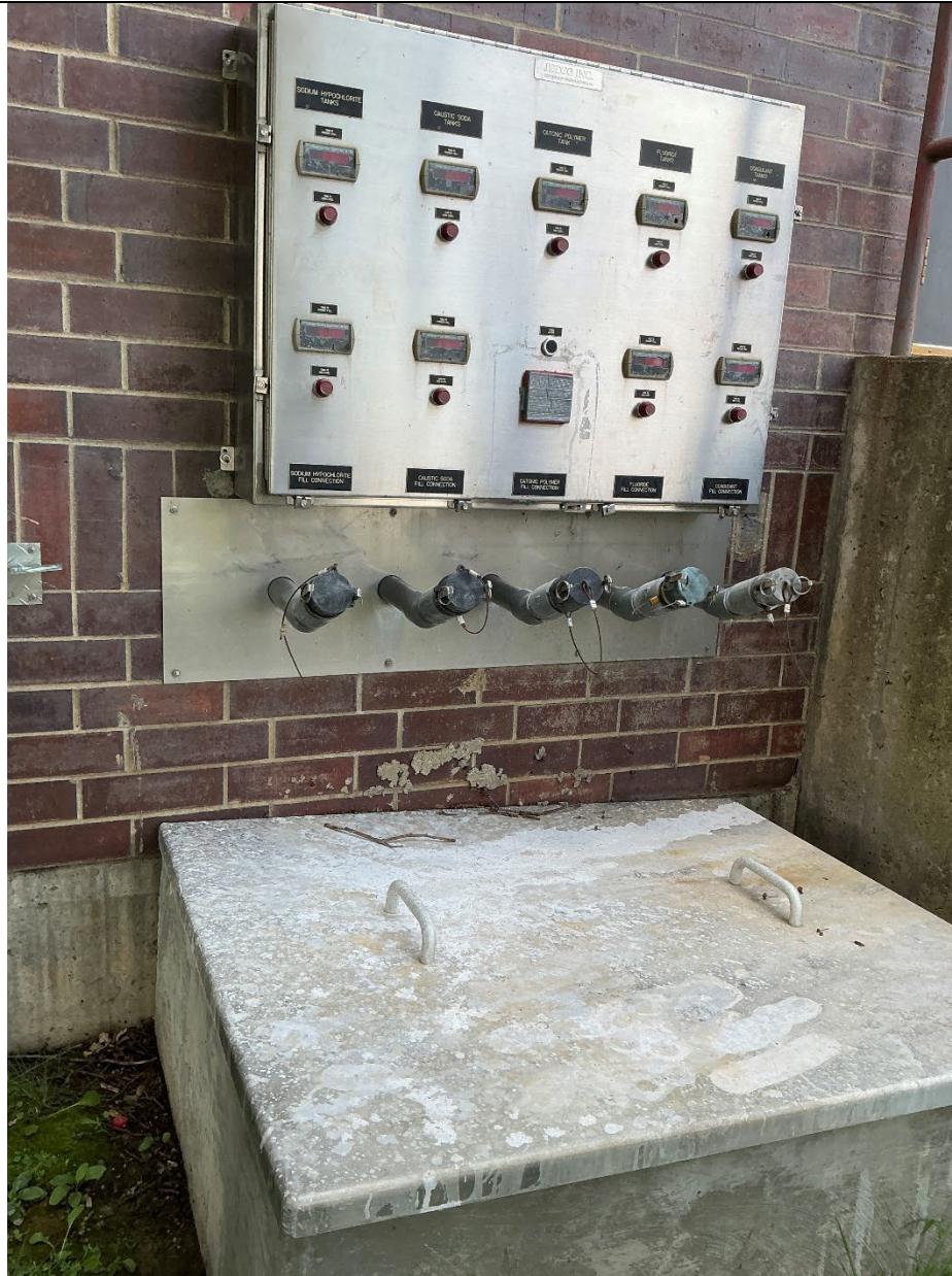
Bulk fill chemical station with inadequate protections.
