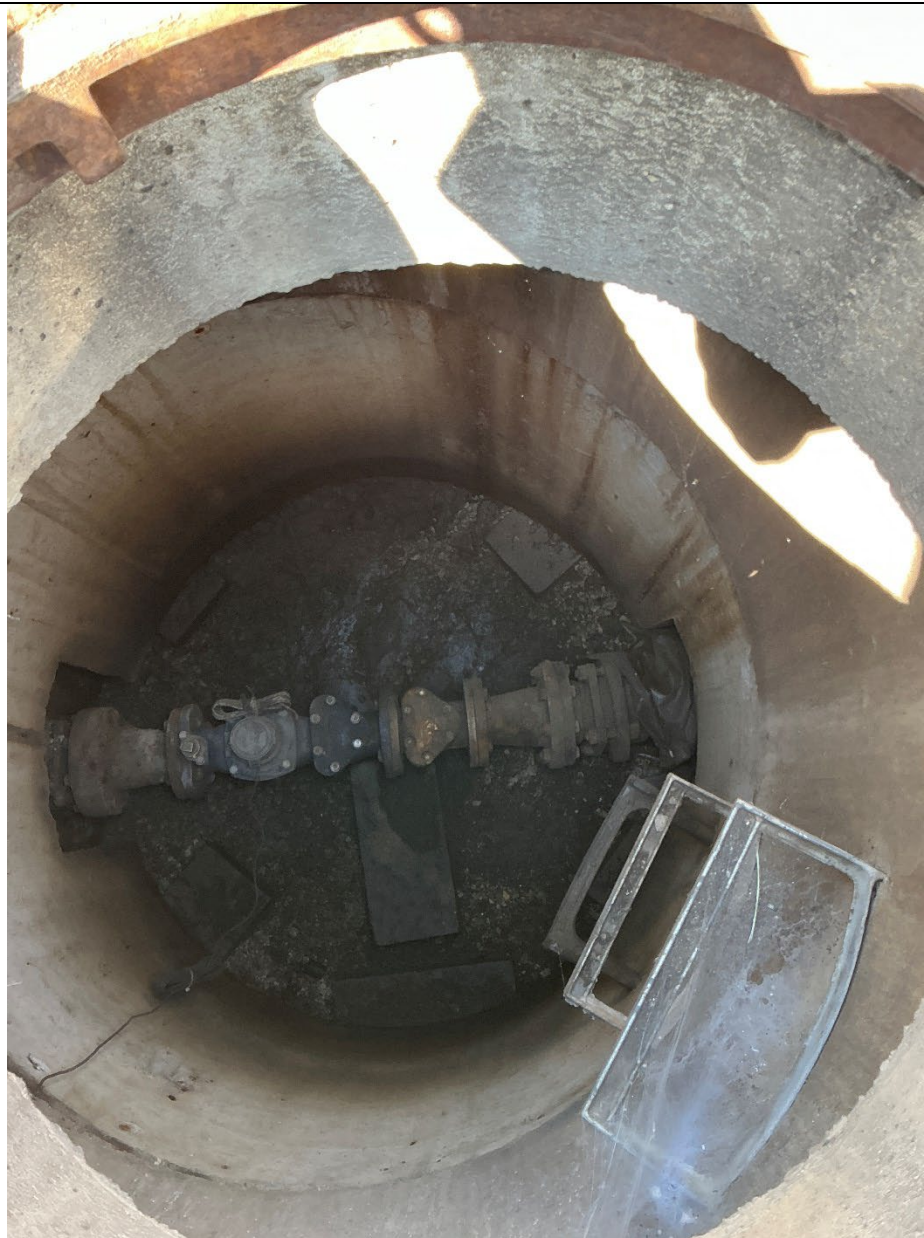
Meter pit connection with the SIRWA system. Owned by SIRWA.
