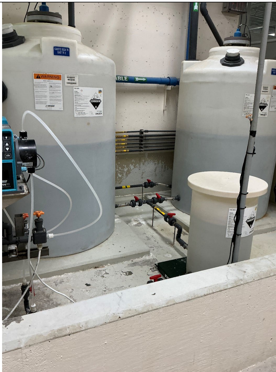
Caustic soda with secondary containment.
