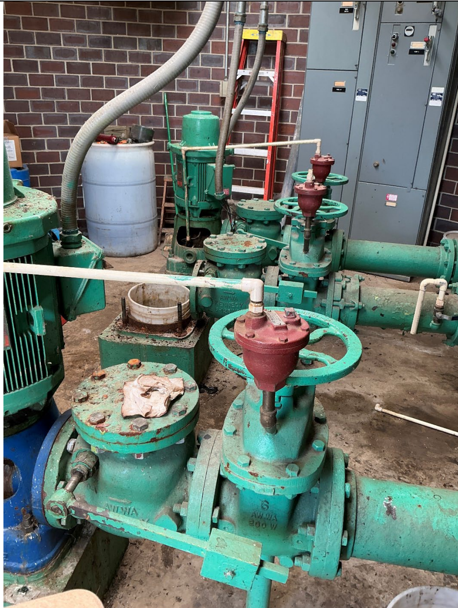
Raw water pumps.
