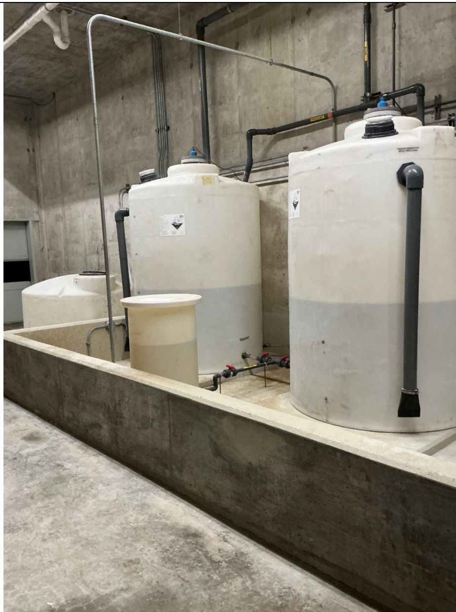
Coagulants with secondary containment.
