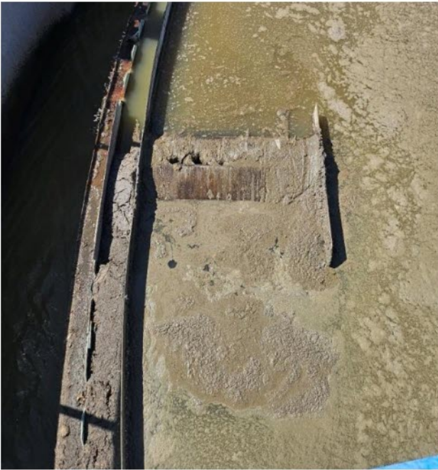
Primary Clarifier Scum Layer
