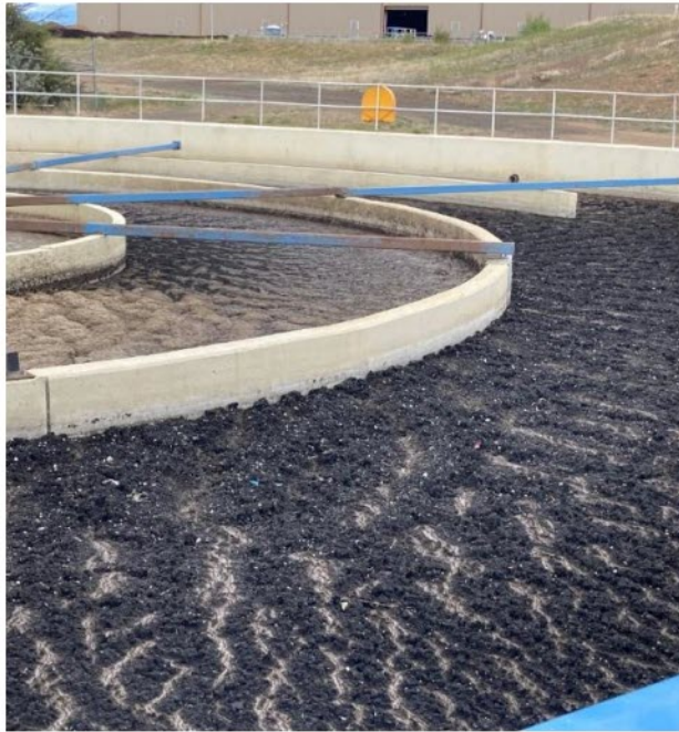
Oxidation Ditch Foam Layer
