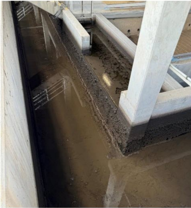
Filter Influent Channel
