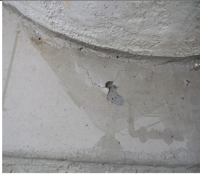
Permitted Tank Farm 1. The inspectors observed the secondary containment next to Tank 19, showed signs of gaps and the paint/sealant was cracked and peeling away from the concrete floor in this area. Photograph 29 taken at 12:15 p.m.
