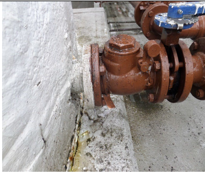
Permitted Tank Farm 3B. The inspectors observed several tags identifying pieces of equipment covered by paint and could not be read. Photograph 23 taken at 11:55 a.m.
