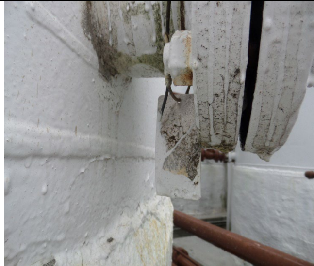
Permitted Tank Farm 3B. The inspectors observed several tags identifying pieces of equipment covered by paint and could not be read. Photograph 25 taken at 12:00 p.m.
