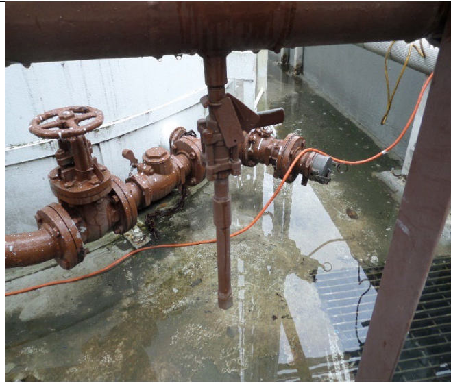
Permitted Tank Farm 1, Distribution Manifold. The inspectors observed several tags identifying pieces of equipment covered by paint and could not be read. Photograph 37 taken at 12:22 p.m.
