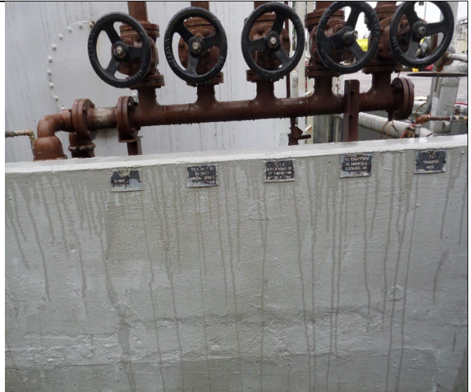
Permitted Tank Farm 1, Distribution Manifold. The inspectors observed several tags identifying pieces of equipment covered by paint and could not be read. Photograph 38 taken at 12:23 p.m.
