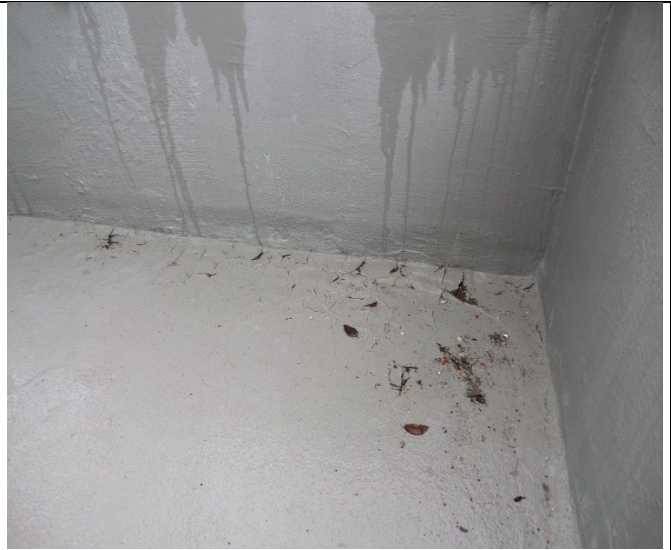
Permitted Tank Farm 1. The inspectors observed the secondary containment in the corner adjacent to Tank 21, showed signs of gaps and the paint/sealant was cracked and peeling away from the concrete floor in this area. Photograph 26 taken at 12:13 p.m.
