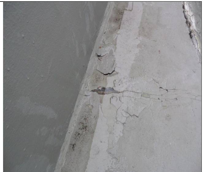
Permitted Tank Farm 1. The inspectors observed the secondary containment next to Tank 23, showed signs of gaps and the paint/sealant was cracked and peeling away from the concrete floor in this area. Photograph 28 taken at 12:14 p.m.
