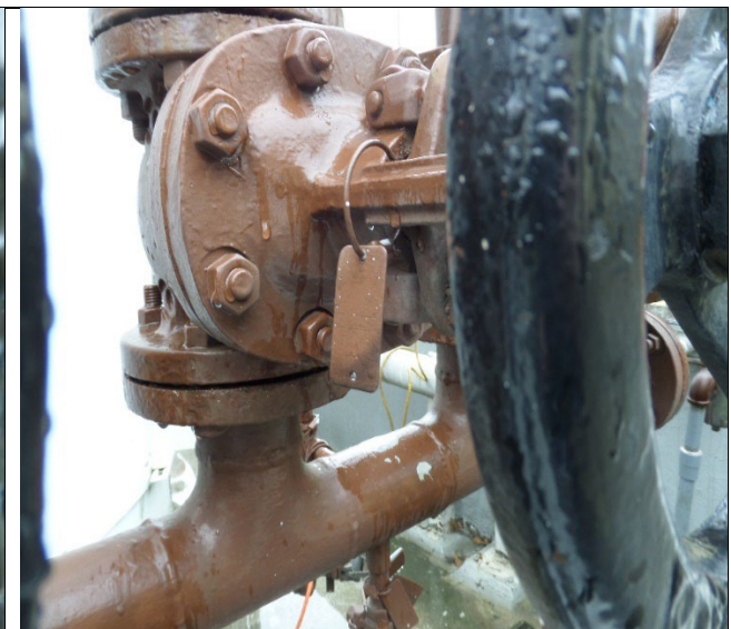
Permitted Tank Farm 1, Distribution Manifold. The inspectors observed several tags identifying pieces of equipment covered by paint and could not be read. Photograph 36 taken at 12:21 p.m.
