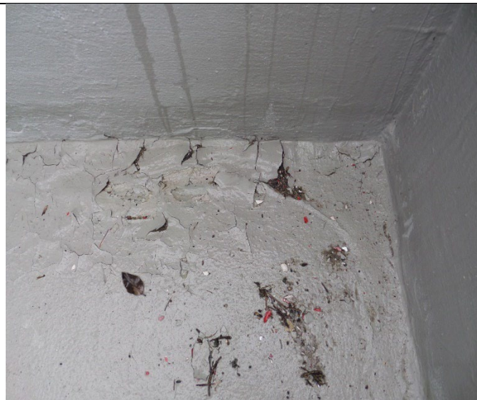
Permitted Tank Farm 1. The inspectors observed the secondary containment in the corner adjacent to Tank 21, showed signs of gaps and the paint/sealant was cracked and peeling away from the concrete floor in this area. Photograph 27 taken at 12:13 p.m.
