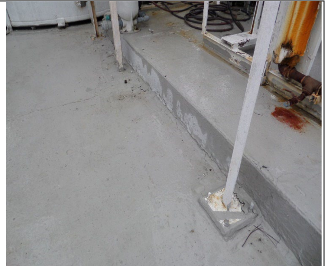
Permitted Tank Farm 1. The inspectors observed the secondary containment next to Tank 14, showed signs of gaps and the paint/sealant was cracked and peeling away from the concrete floor in this area. Photograph 32 taken at 12:17 p.m.
