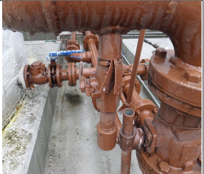
Permitted Tank Farm 3B. The inspectors observed several tags identifying pieces of equipment covered by paint and could not be read. Photograph 22 taken at 11:55 a.m.
