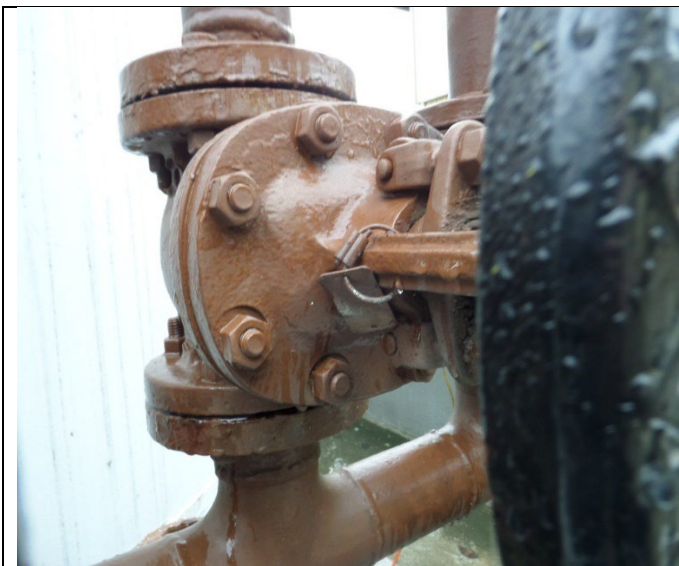
Permitted Tank Farm 1, Distribution Manifold. The inspectors observed several tags identifying pieces of equipment covered by paint and could not be read. Photograph 35 taken at 12:21 p.m.
