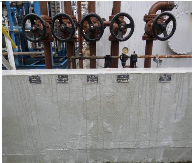
Permitted Tank Farm 1, Distribution Manifold. The inspectors observed several tags identifying pieces of equipment covered by paint and could not be read. Photograph 39 taken at 12:24 p.m.
