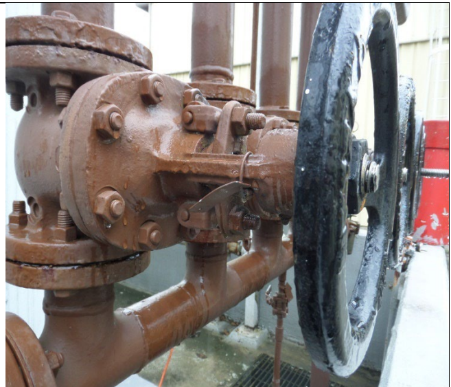
Permitted Tank Farm 1, Distribution Manifold. The inspectors observed several tags identifying pieces of equipment covered by paint and could not be read. Photograph 34 taken at 12:21 p.m.
