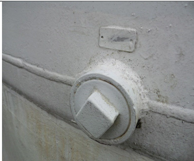
Permitted Tank Farm 6B. The inspectors observed one tag (above the fitting) that was completely covered by paint and unable to be read. SK provided a photograph of the tag (OE4610) after it had been cleaned in their email response dated February 10, 2023. Photograph 19 taken at 11:43 a.m.
