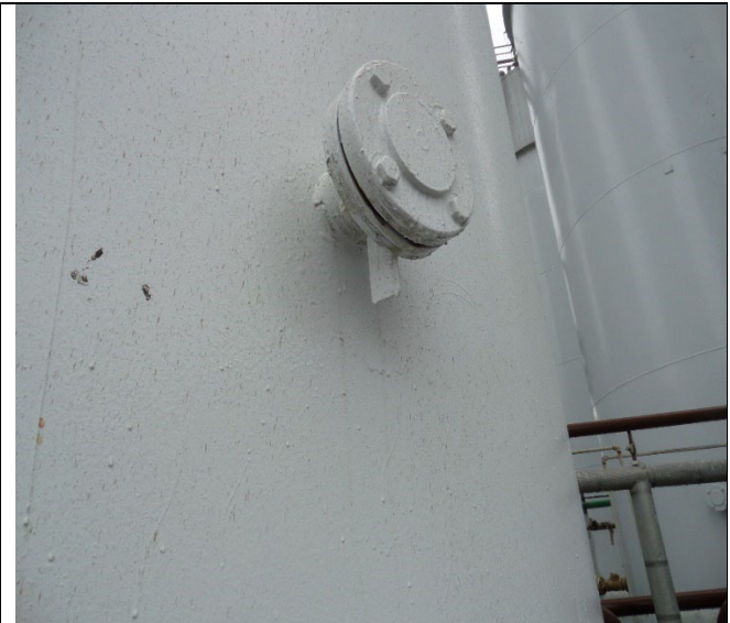
Permitted Tank Farm 3B. The inspectors observed the tag (tank connection port) identifying pieces of equipment covered by paint and could not be read. Photograph 24 taken at 12:00 p.m.
