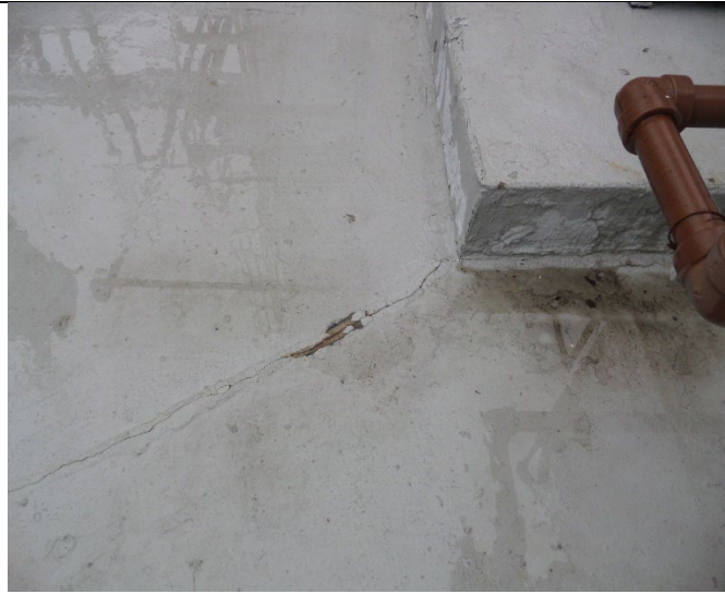
Permitted Tank Farm 1. The inspectors observed the secondary containment next to Tank 14, showed signs of gaps and the paint/sealant was cracked and peeling away from the concrete floor in this area. Photograph 31 taken at 12:17 p.m.
