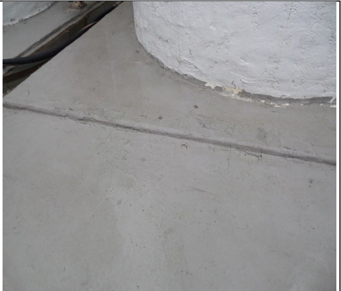
Permitted Tank Farm 1. The inspectors observed the secondary containment next to Tank 19, showed signs of gaps and the paint/sealant was cracked and peeling away from the concrete floor in this area. Photograph 30 taken at 12:16 p.m.
