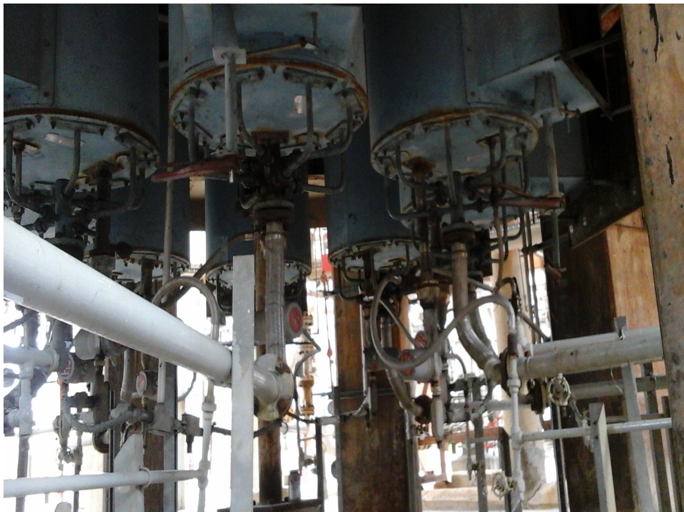
Crude Heater 301 Lo-NO x burners.
