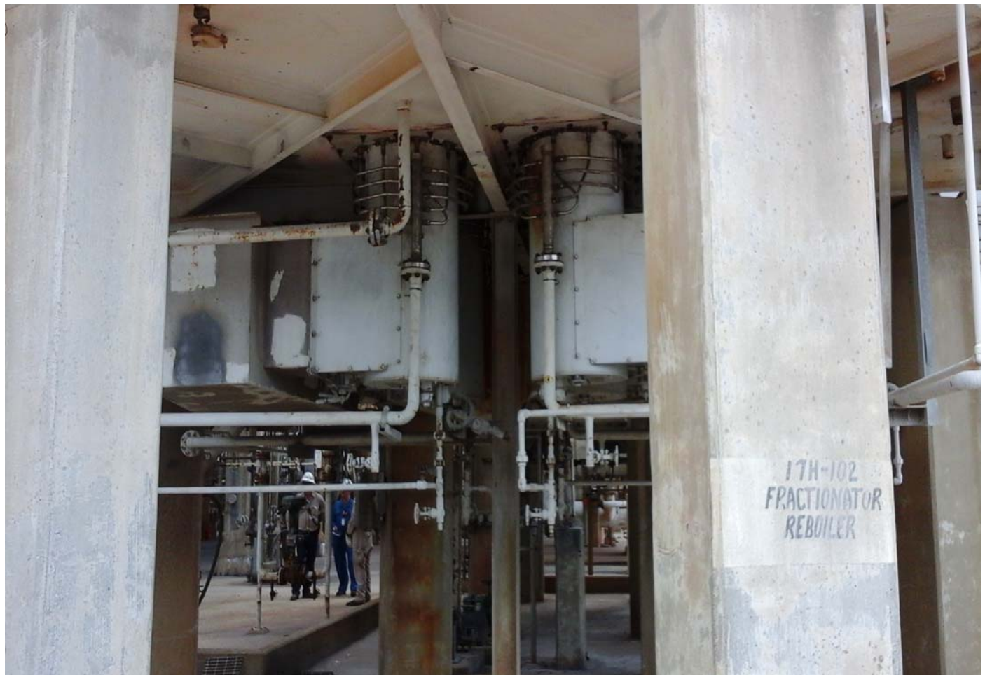
Reformer Heater H-102 Lo NO x burners.
