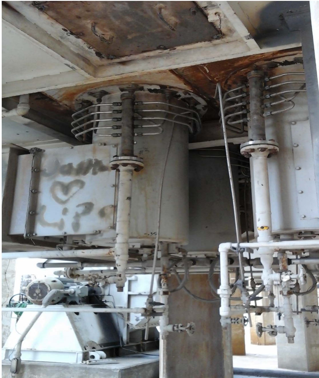
Reformer Heater H-101 Lo NO x burners.
