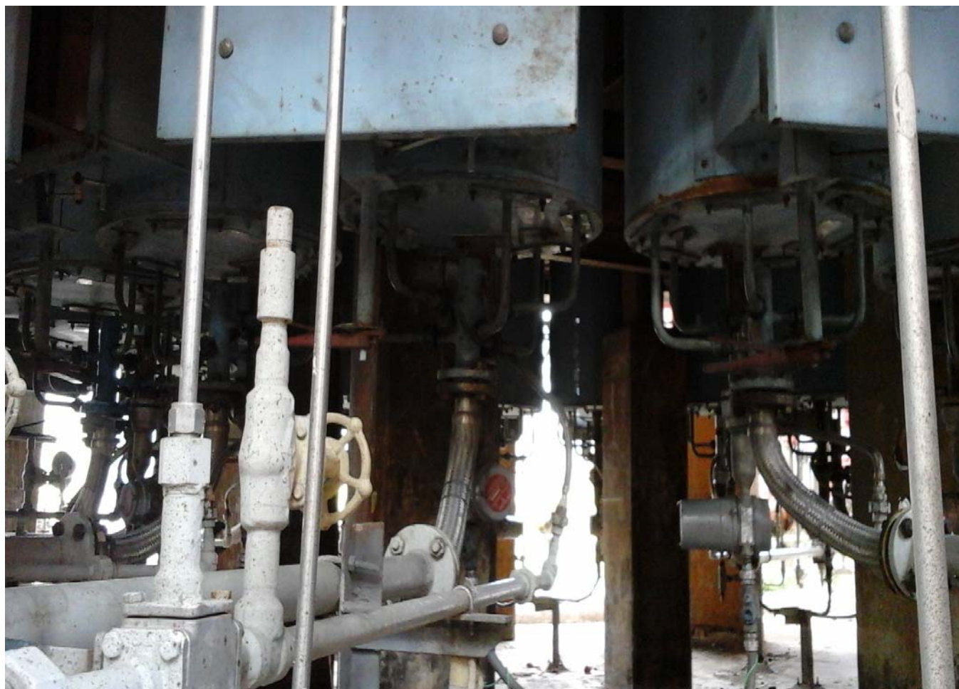
Crude Heater 201 Lo-NO x burners.
