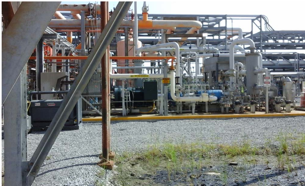
Flare Gas Recovery 2 Compressors.
