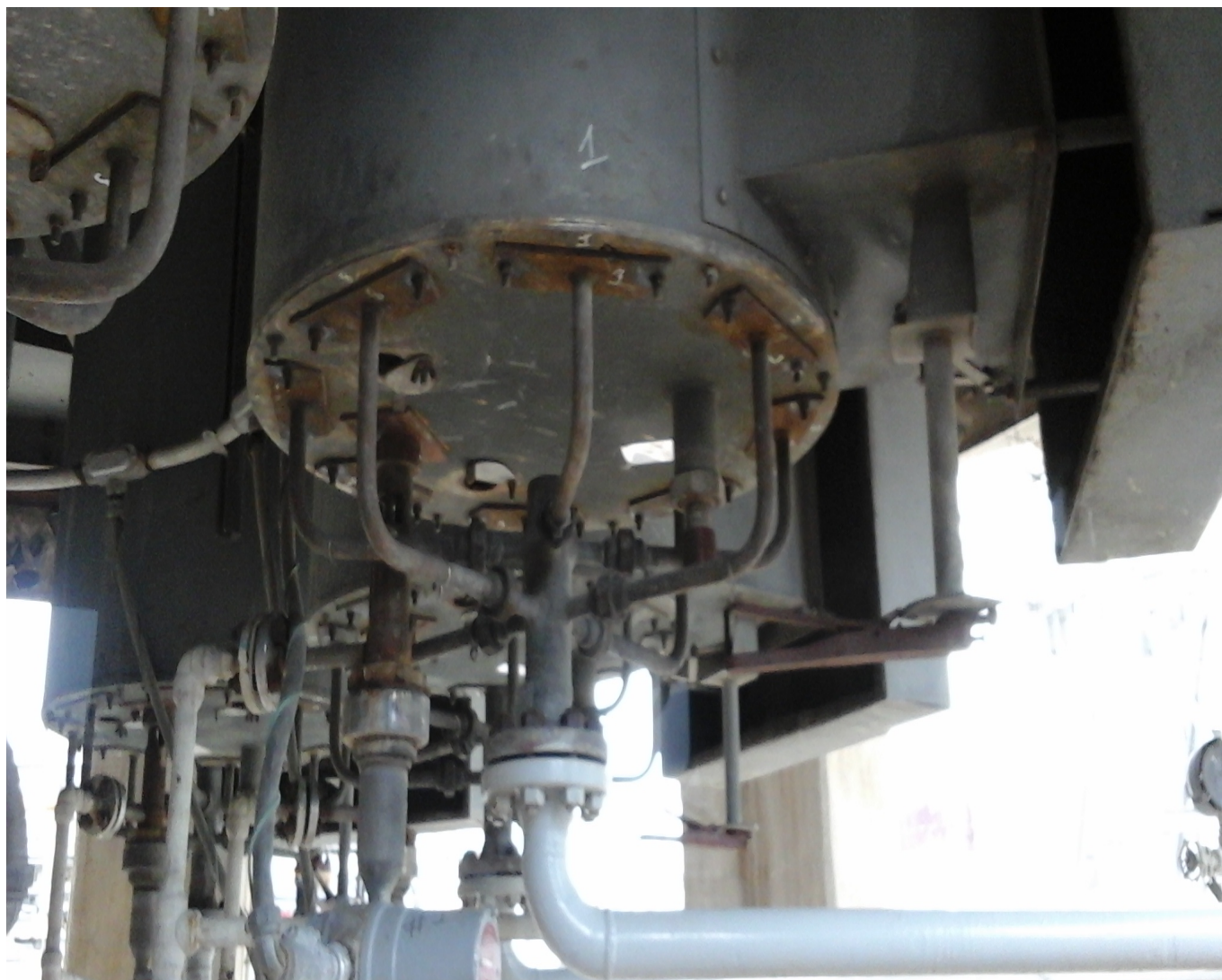
Crude Heater 101 Lo-NO x burners
