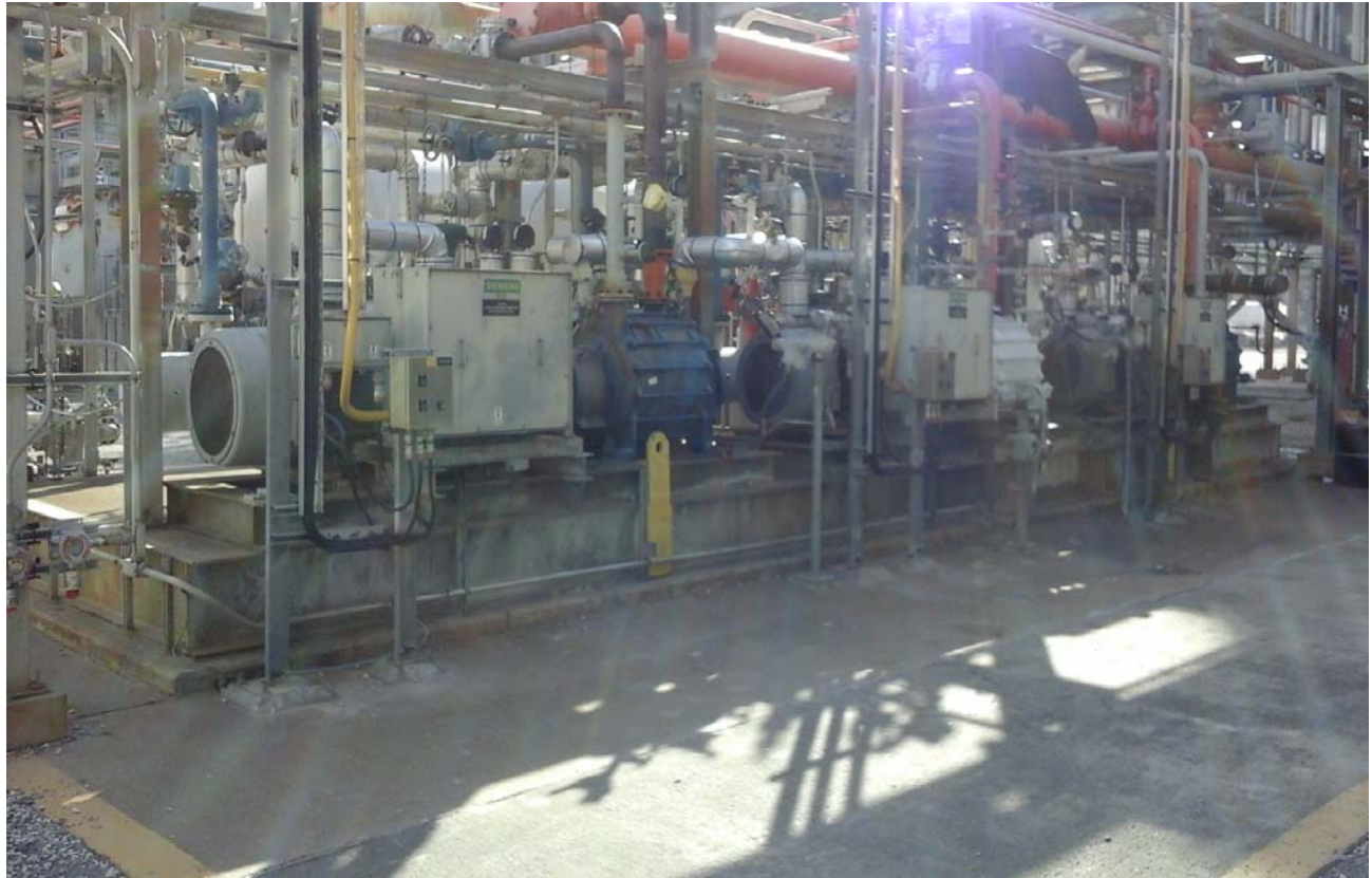
Flare Gas Recovery 1 Compressors
