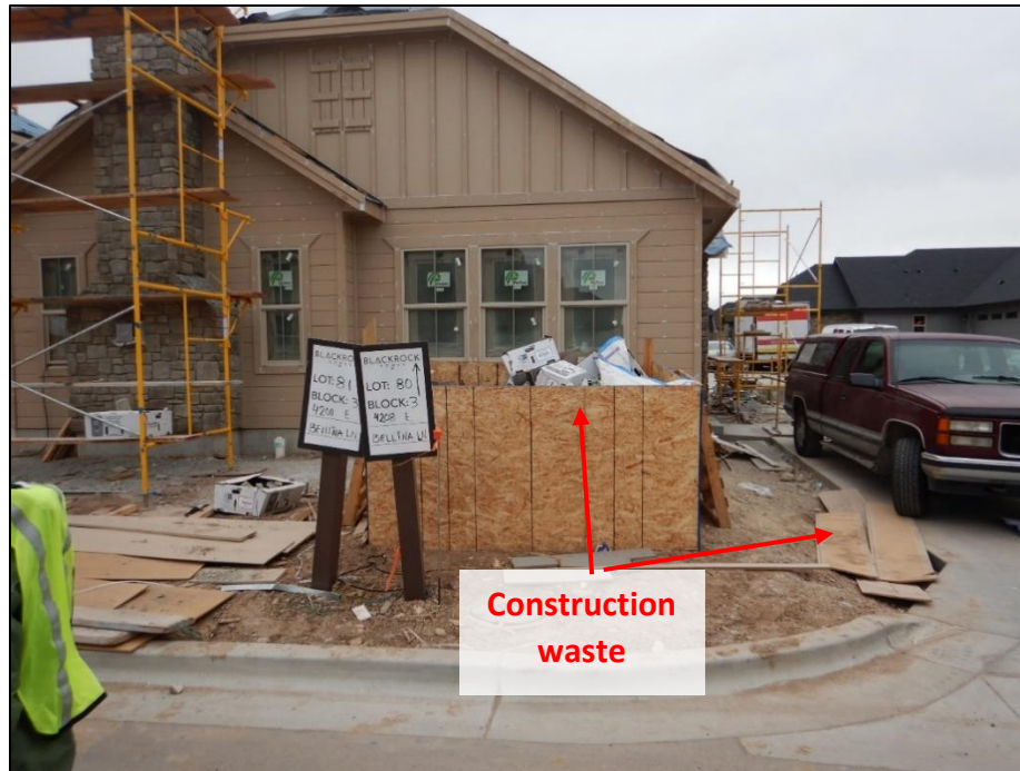
Photograph 4. View, facing west, of a pile of construction waste and debris in an uncovered plywood container located on the northern perimeter of Phase 5 in lot 80.
