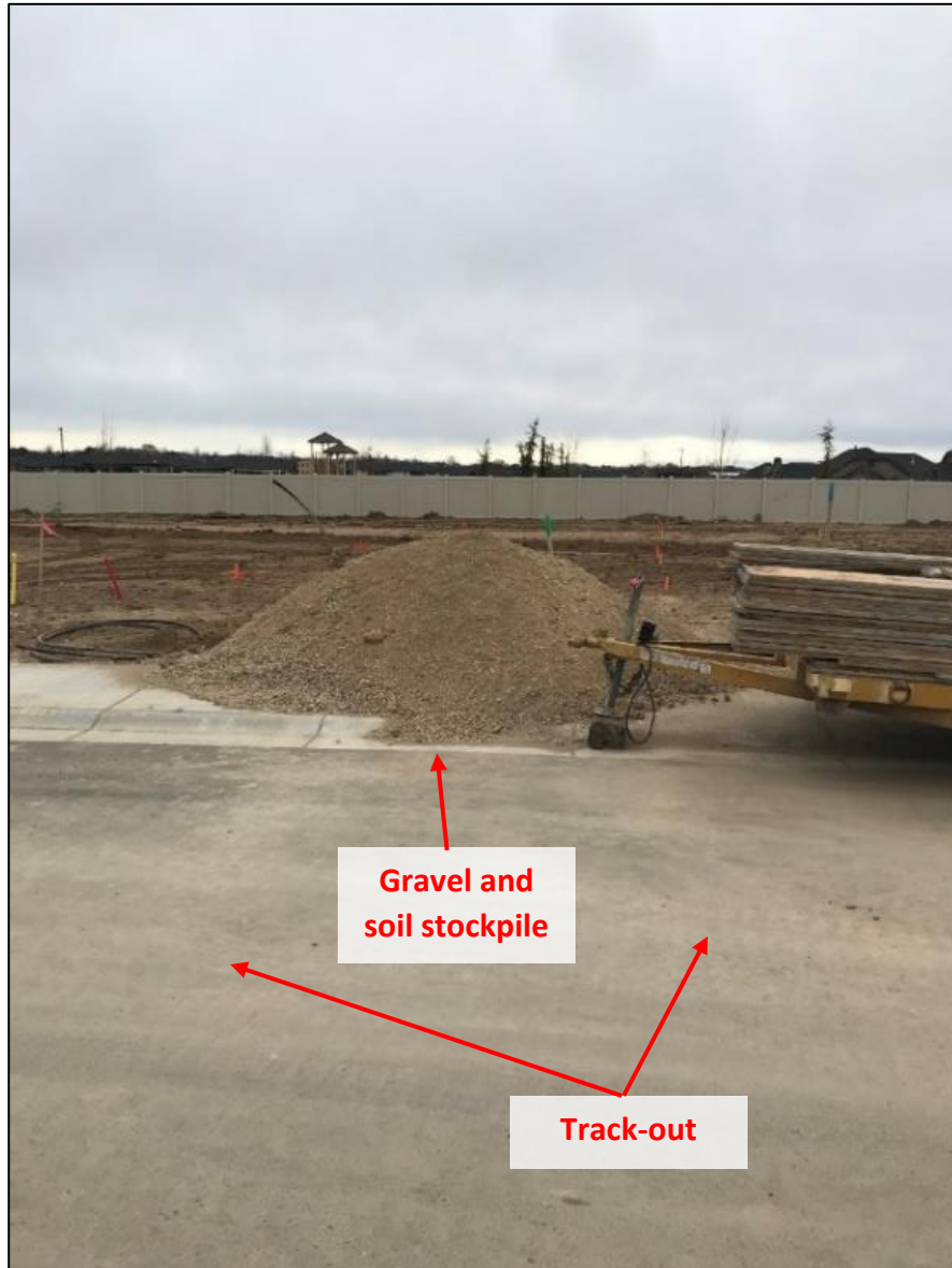
Photograph 3. View, facing east, of a gravel and soil stockpile located on the eastern area of the Site in Phase 7 on South Movado Way. The soil stockpile did not have a sediment barrier installed on the downgradient perimeter areas on the roadway and appeared to be contributing to track-out on the surrounding roadway.
