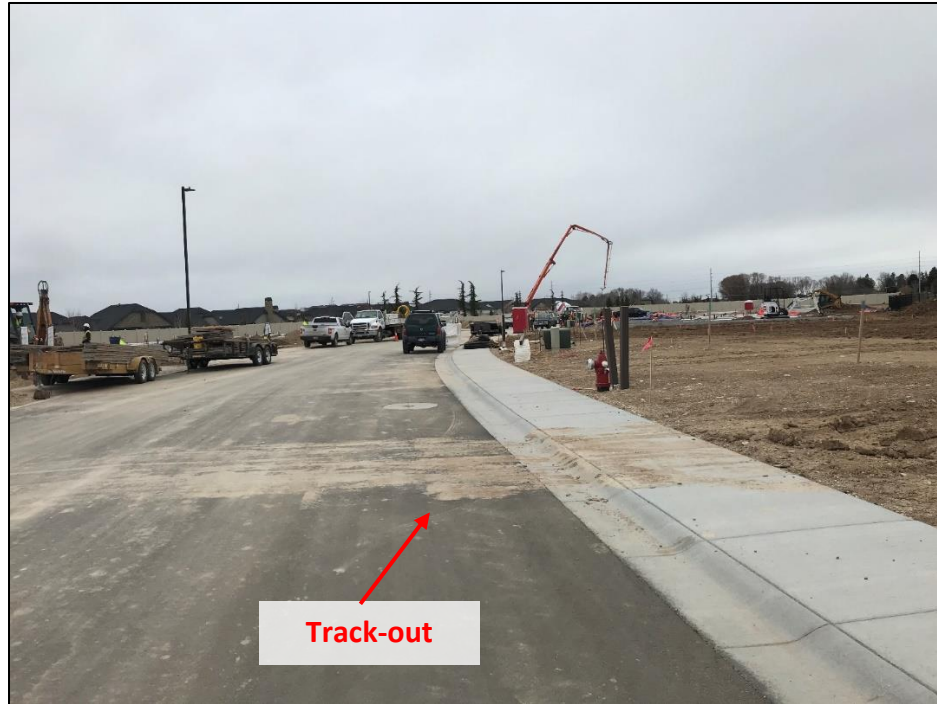
Photograph 10. View, facing north, of a non-designated and unstabilized access point on South Movado Way. Note the sediment track out on to paved roadways.
