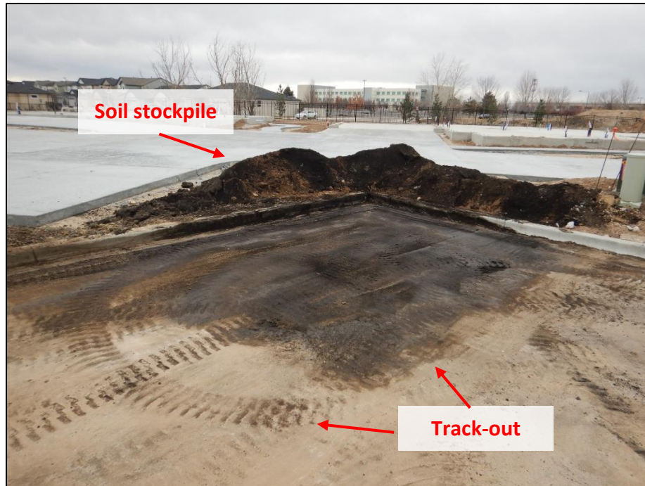
Photograph 1. View, facing southwest, of a soil stockpile located on the northwestern perimeter of Phase 5 on a roadway. The stockpile did not have a sediment barrier installed downgradient. Note the track out surrounding the soil stockpile.
