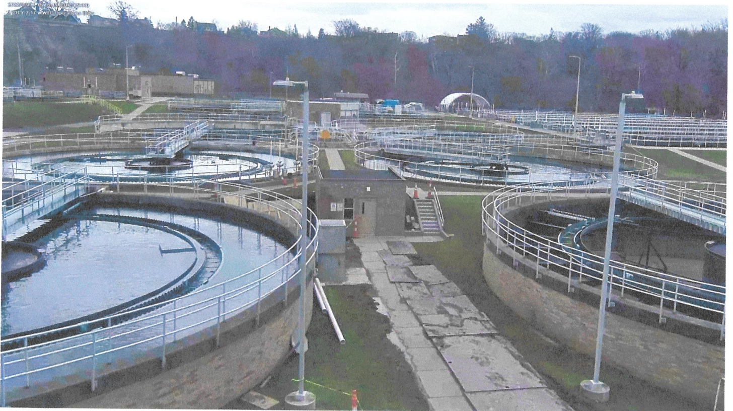
Final Clarifiers, S&G Building, CEHRT Facility
