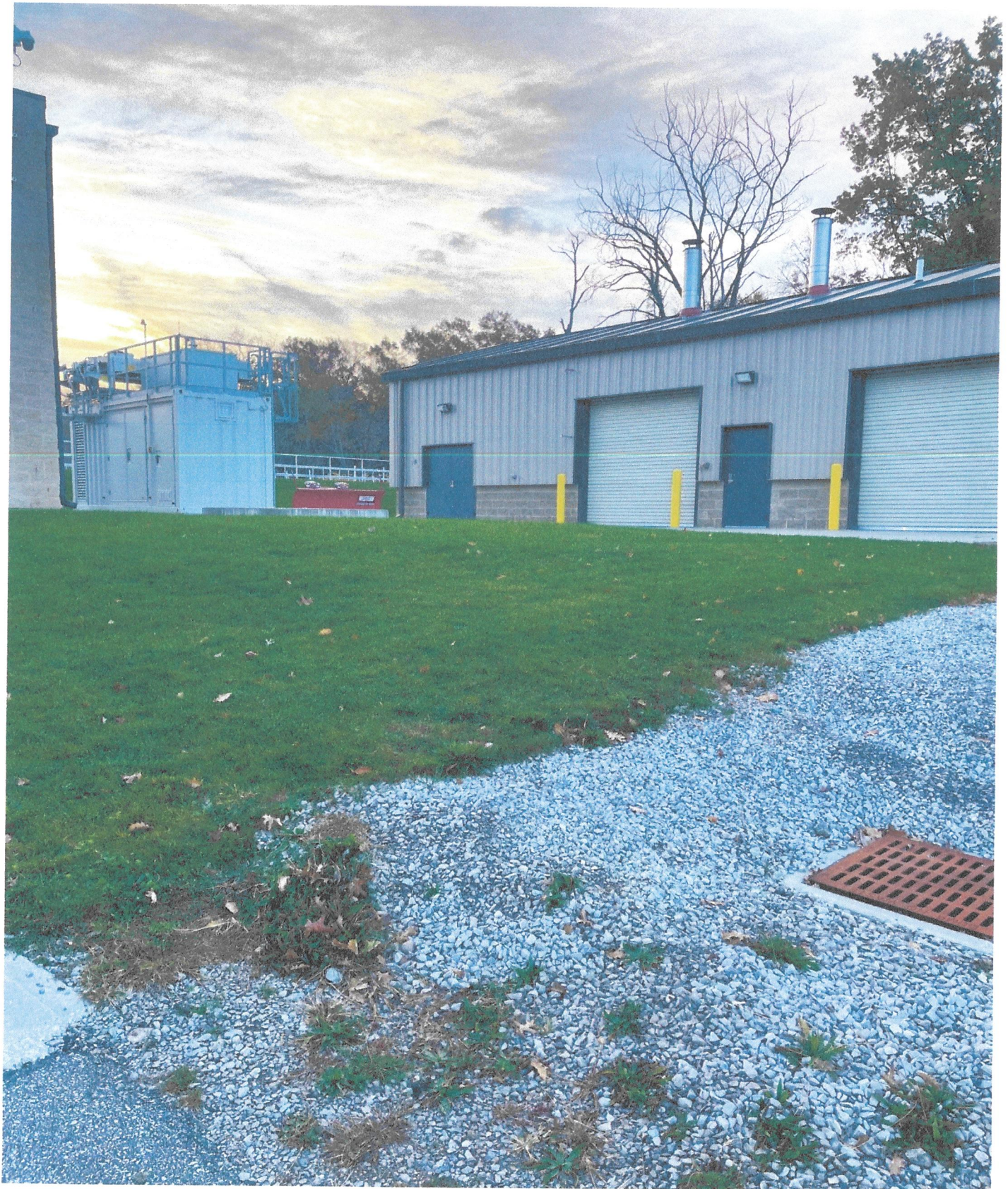
CHP (Combined Heat & Power) Generator and ERB (Energy Recovery Building)
