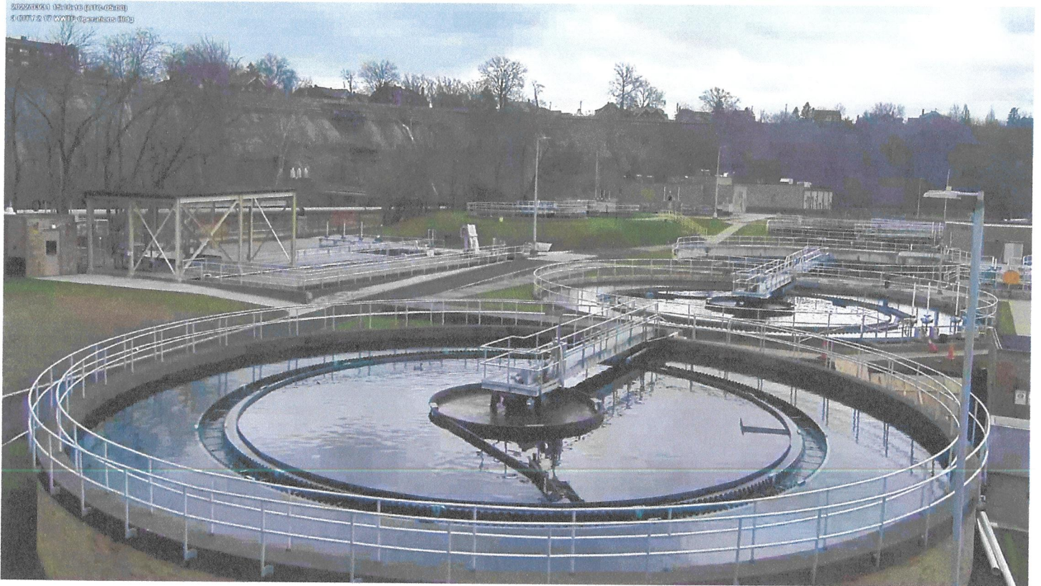
WWTP Effluent, Final Clarifiers #3 and #5
