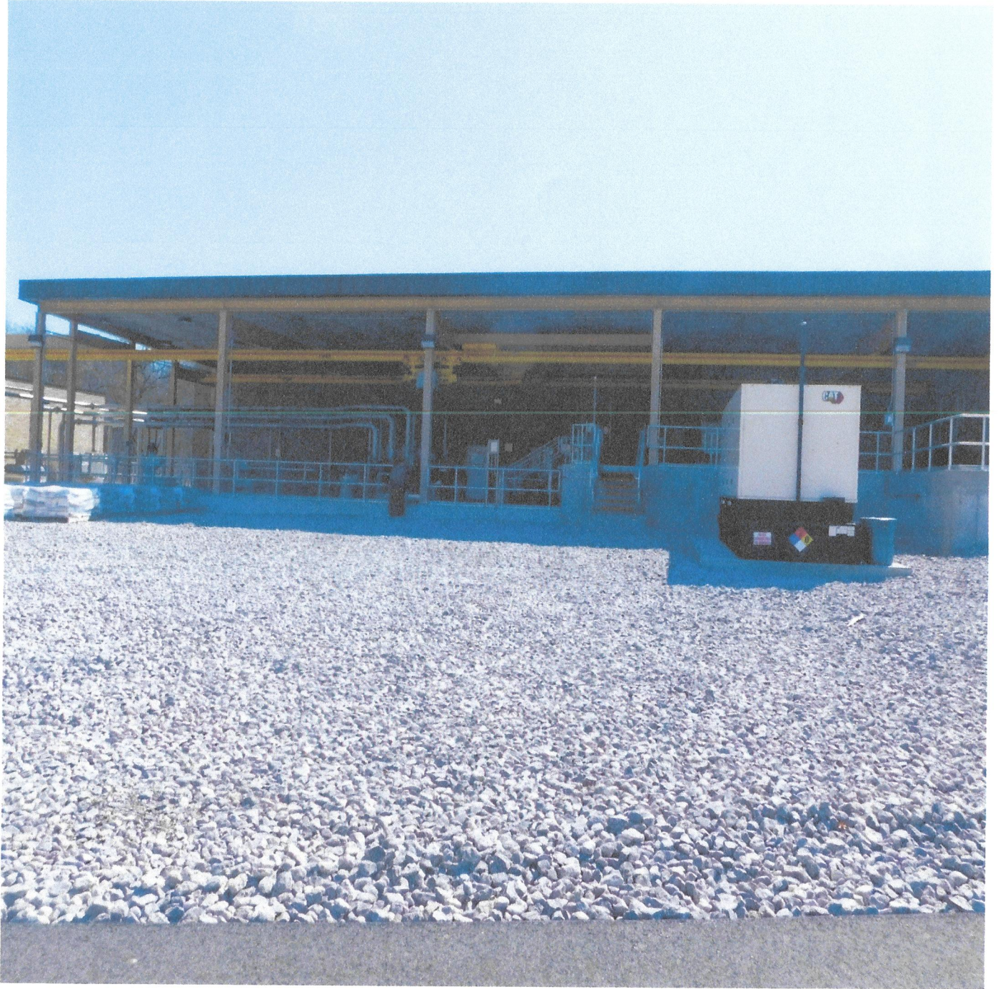
Actual HRT Actiflo Portion Canopy and Emergency Backup Generator
