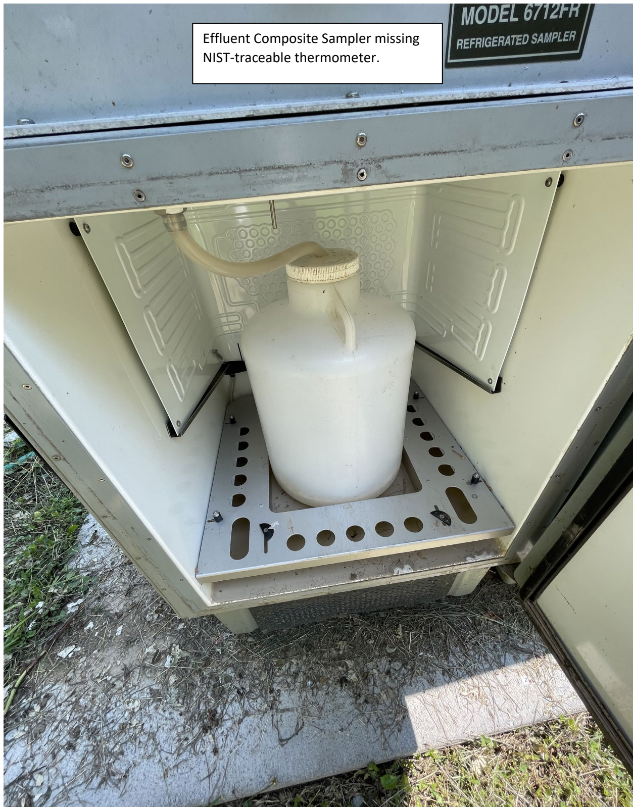
Figure 4: Effluent composite sampler photo: Taken 6/13/23 10:12 am
