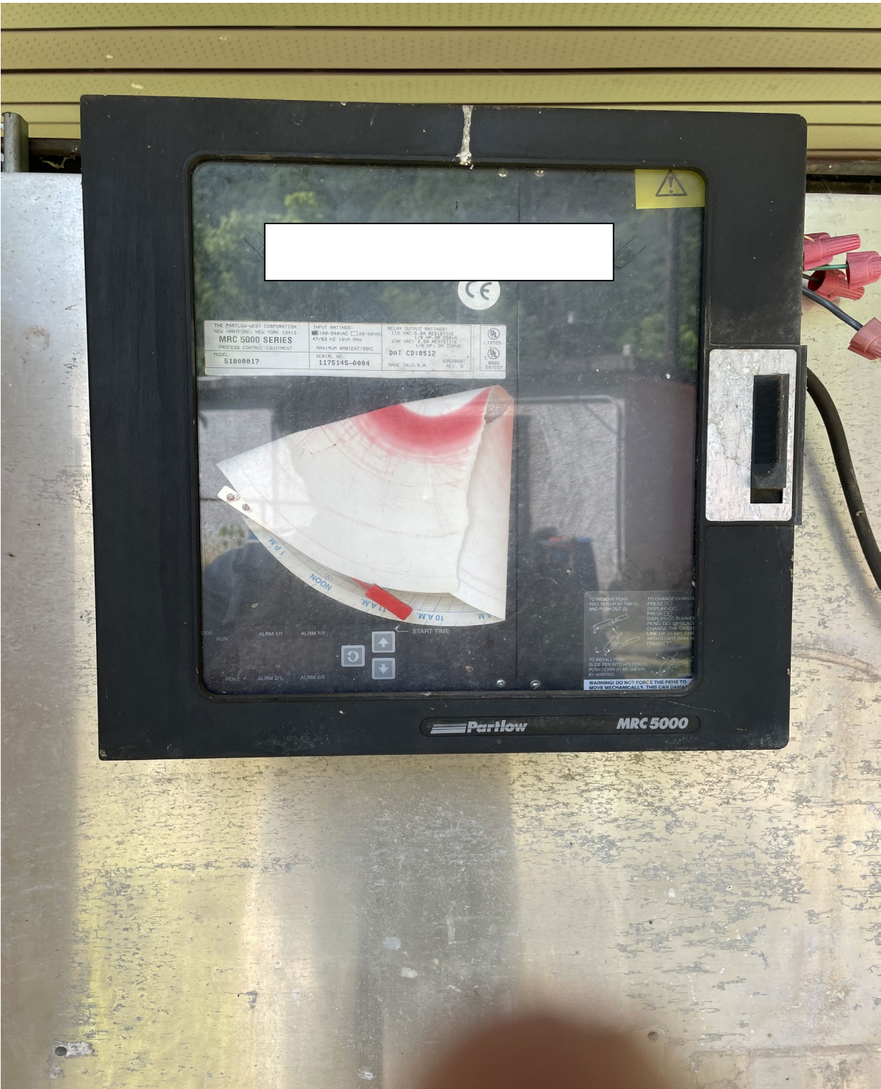
Figure 5: Effluent Flow Totalizer non-operating photo: Taken 6/13/23 10:18 am
