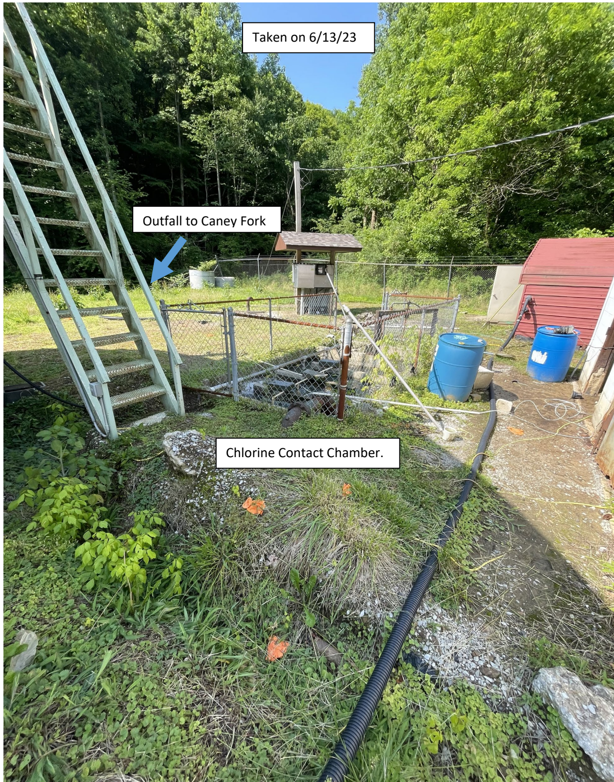
Figure 2: Facility grounds Chlorine contact chamber, effluent discharge photo: Taken 6/13/23 10:10 am
