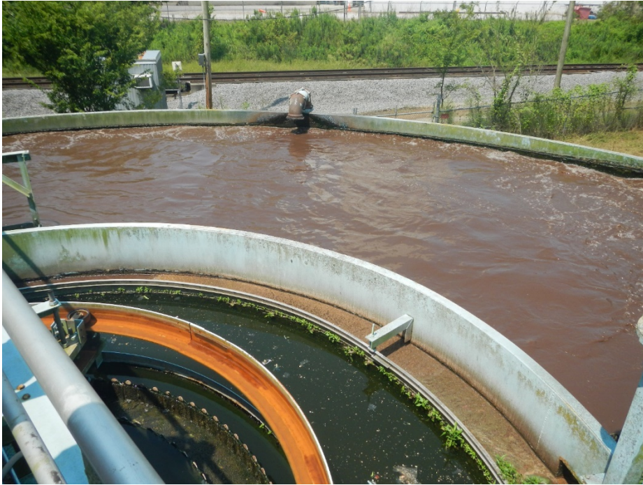
Photo 7: Influent pipe from pump station to aeration tank 2.
