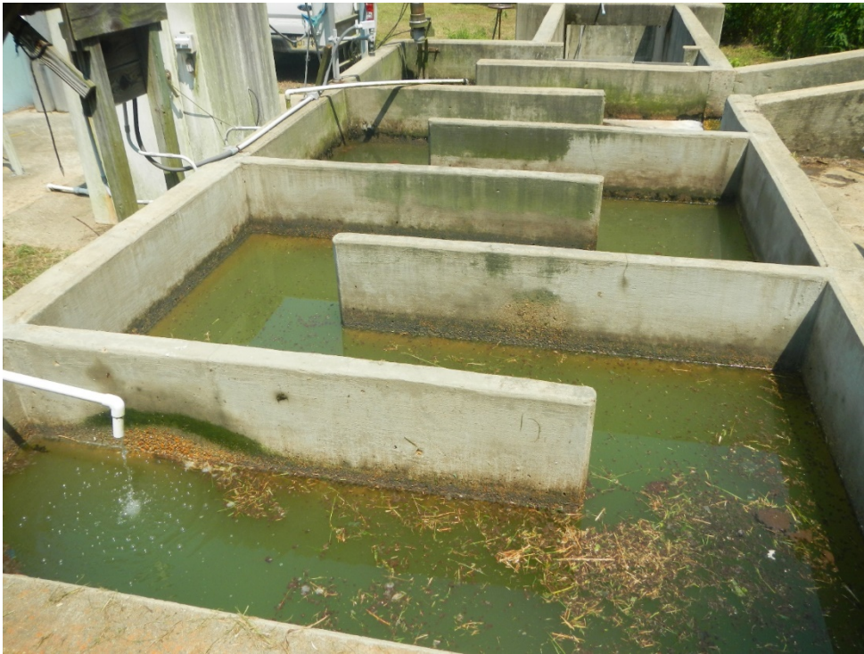
Photo 15:Chlorine contact chamber 1.
