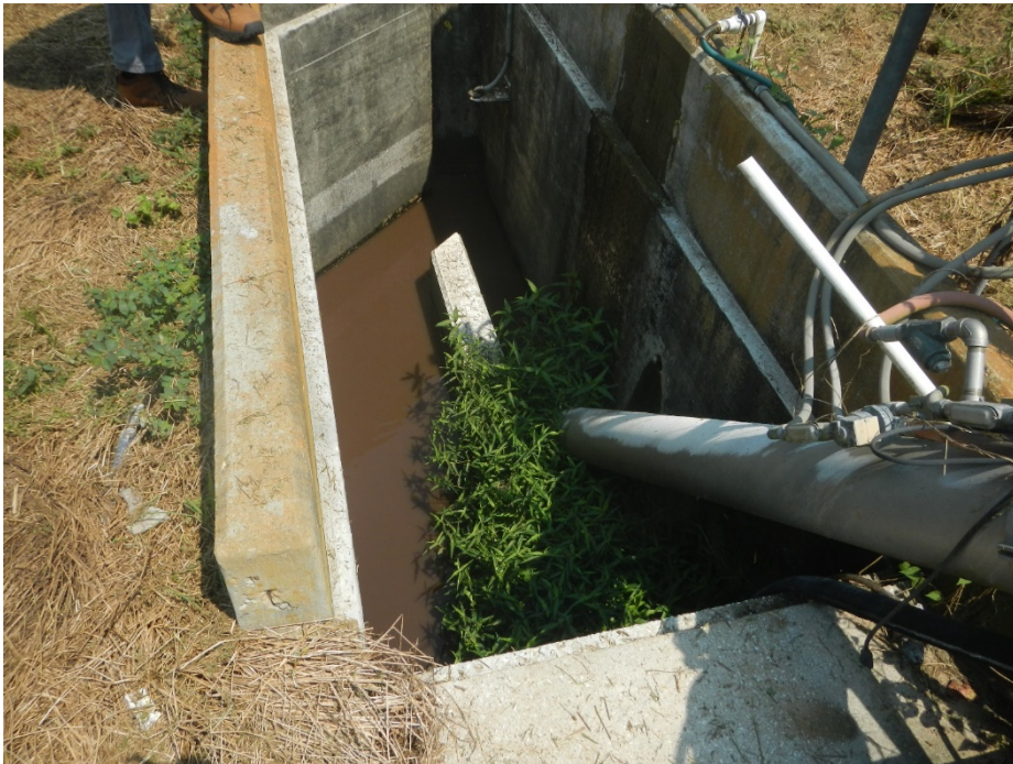
Photo 2: Facility headworks. Area is overgrown and cleaning mechanism inoperable.
