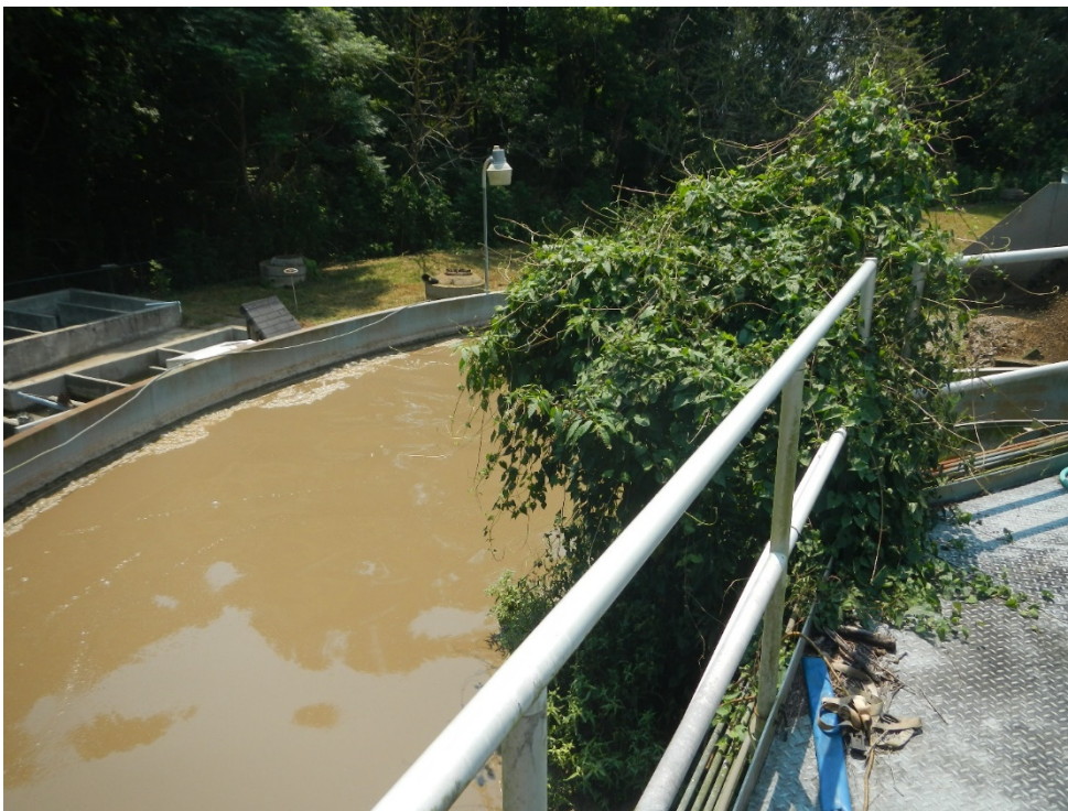
Photo 12: Heavy vegetative growth and water coloration in aeration tank 1.
