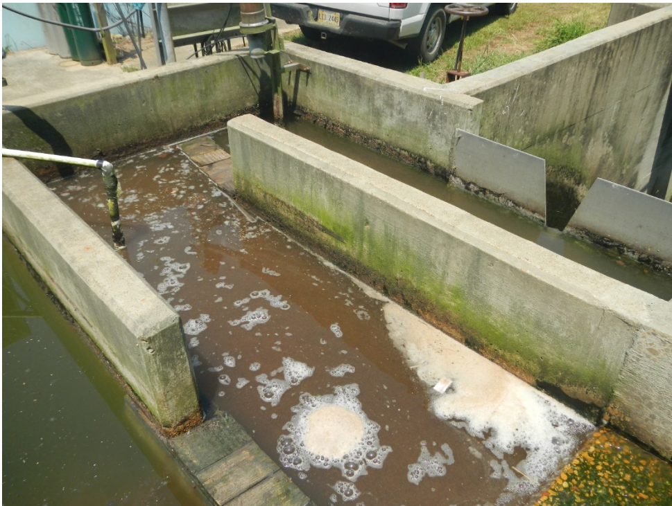
Photo 16: Foam and solids after chlorine contact chamber 1.
