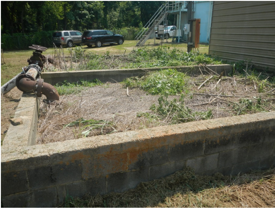
Photo 3 :Overgrown drying beds.
