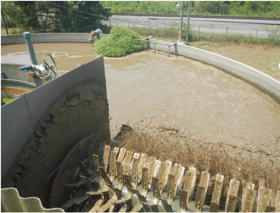
Photo 13: Vegetative growth and aerator in aeration tank 1.
