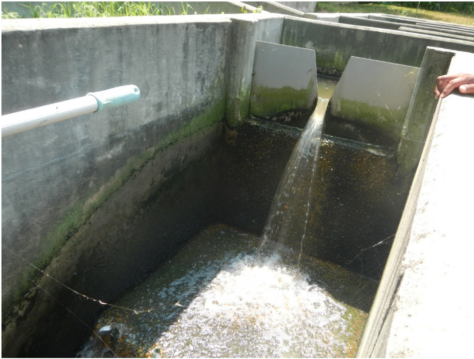
Photo 20: Effluent v-notch weir. Solids visible in effluent.
