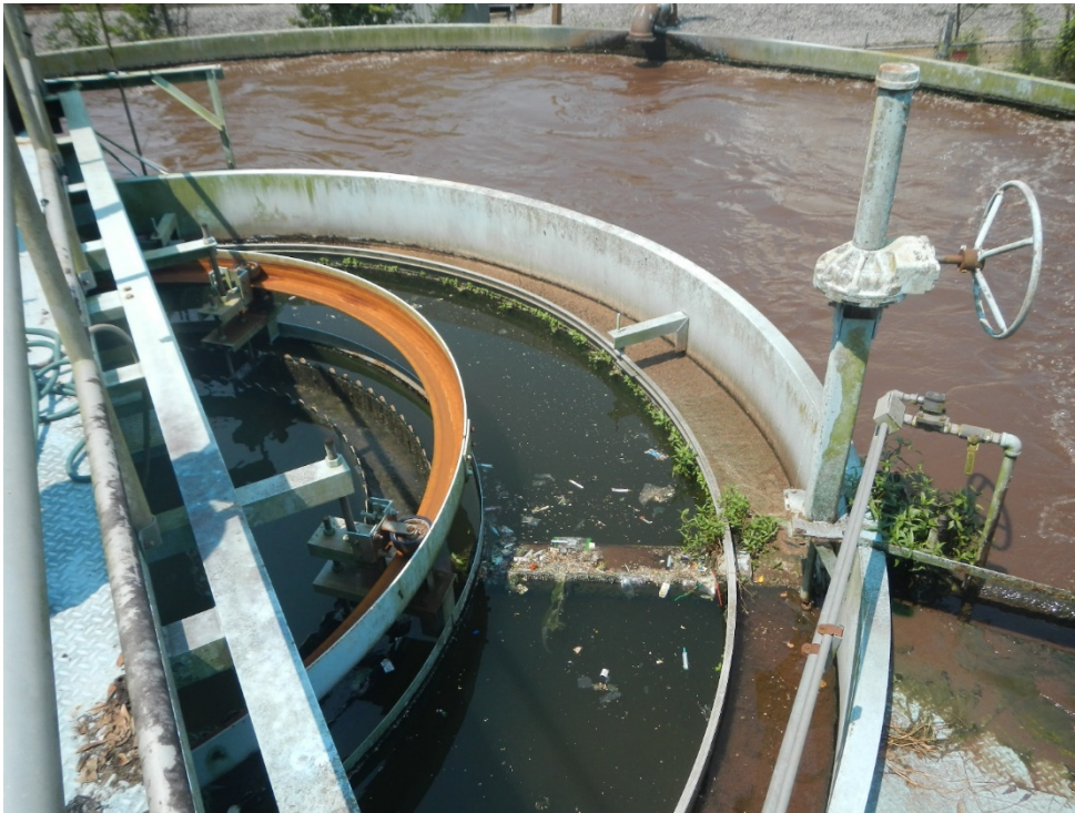
Photo 9: Suspended trash and vegetative growth in aeration tank 2.
