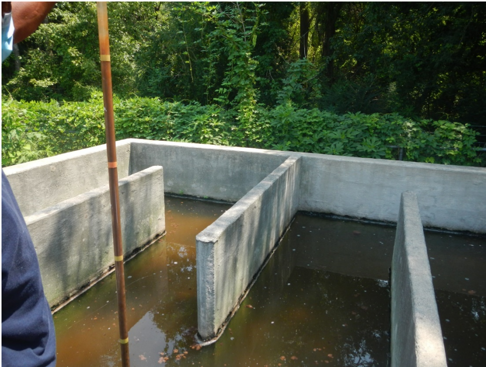
Photo 19: Sludge judge from chlorine contact chamber 2.
