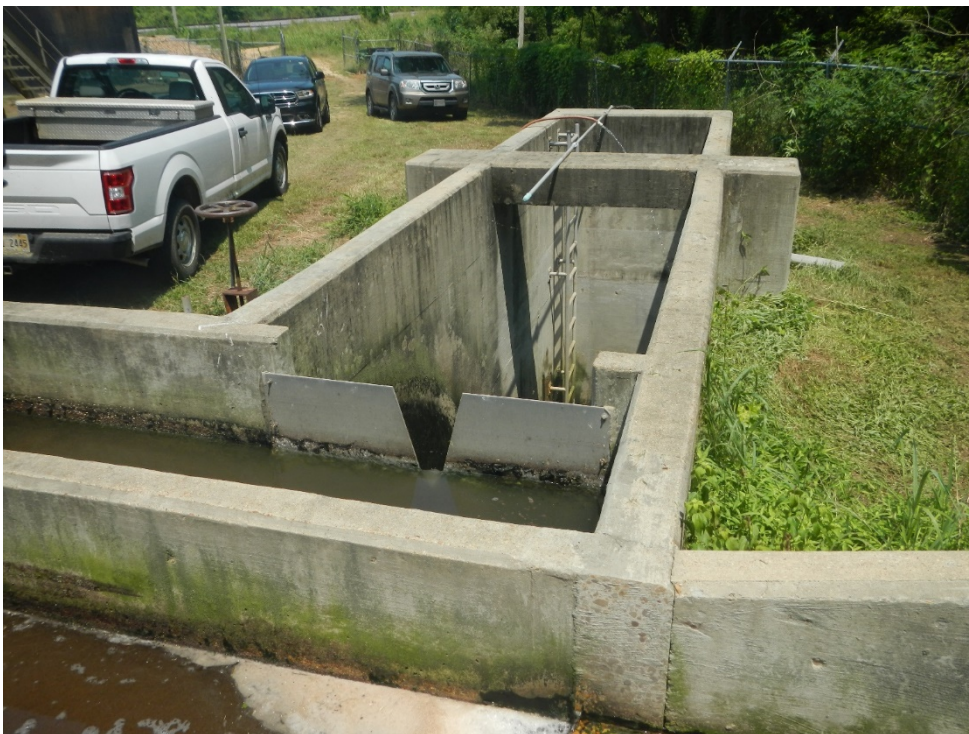
Photo 20: Effluent v-notch weir.
