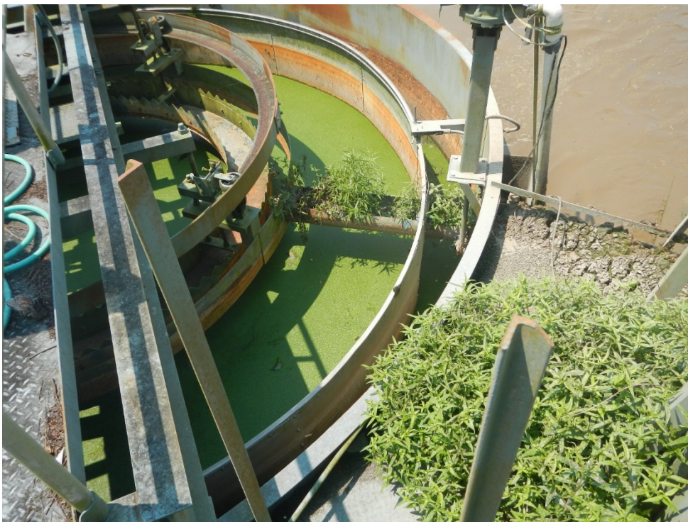
Photo 14: Vegetative and algae growth in aeration tank 1.
