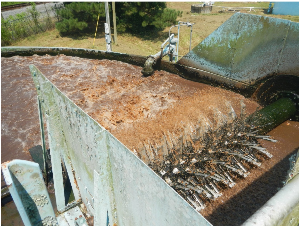
Photo 8: Aerator in aeration tank 2. Return sludge pipe.
