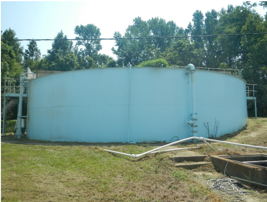
Photo 6: Aeration tank 2 from new pump station.
