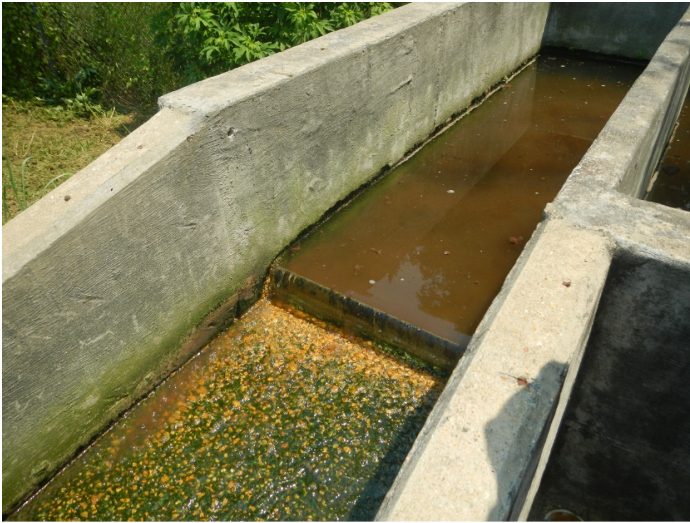
Photo 17: Solids after chlorine contact chamber 2.
