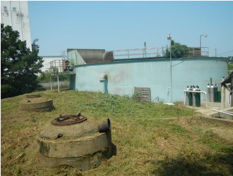
Photo 11: Aeration tank 1 and manholes leading to chlorine contact chambers.
