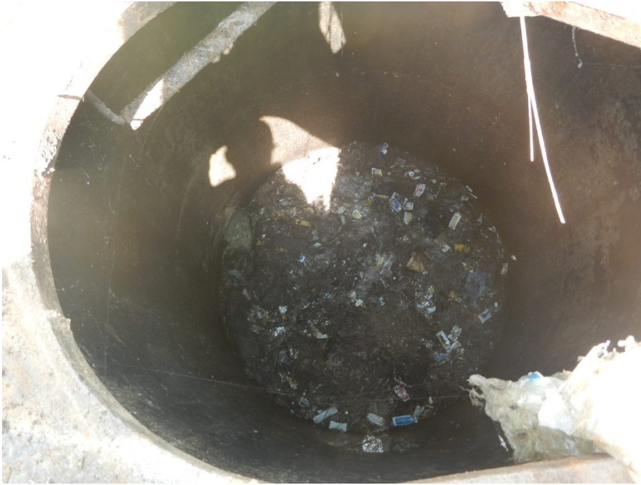
Photo 1: Old Influent lift station. Inoperable and filled with trash and debris.
