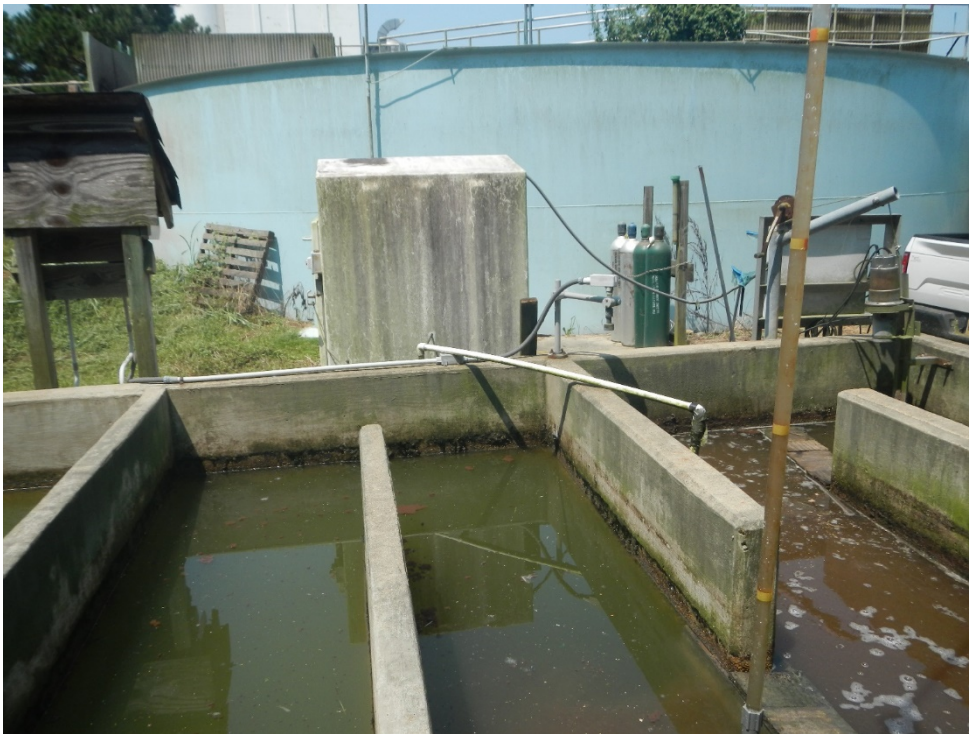
Photo 18: Sludge judge from chlorine contact chamber 1.
