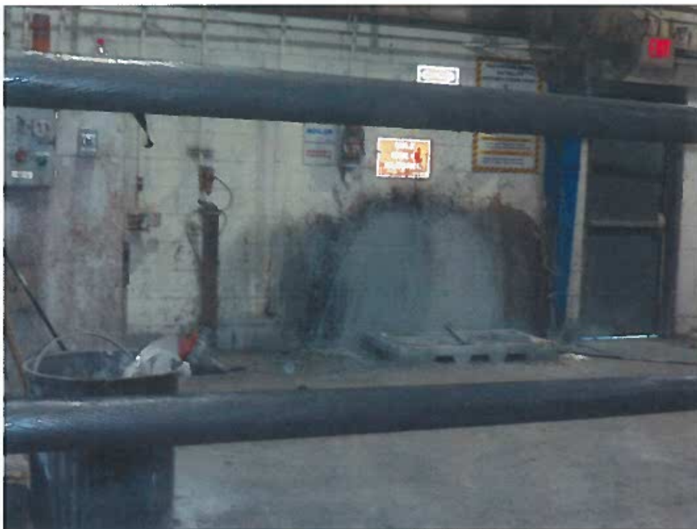
Photo 17: SAA for accumulating waste MEK used to flush painting lines in the automated painting area within the Light Pole Building.
