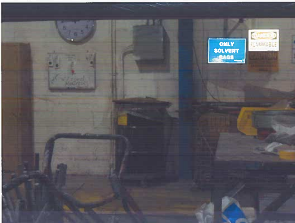
Photo 16: SAA for accumulating solvent contaminated rags used in the painting area within the Light Pole Building.
