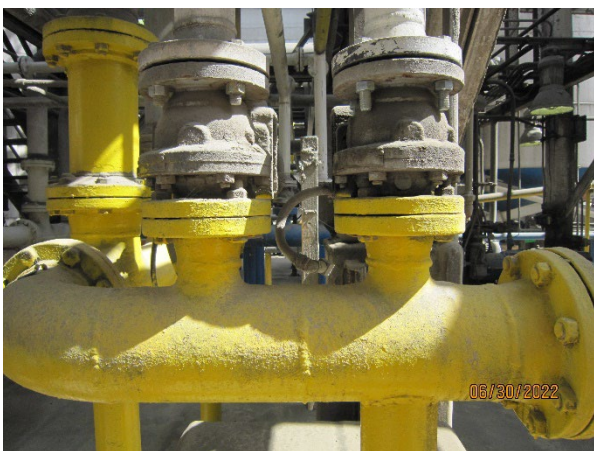
Tank Farm area with indistinguishable tags on equipment. Photograph 11 taken at 10:48am
