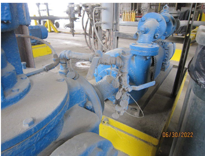
LWDF Loading Area equipment with indistinguishable tags. Photograph 3 taken at 10:34am
