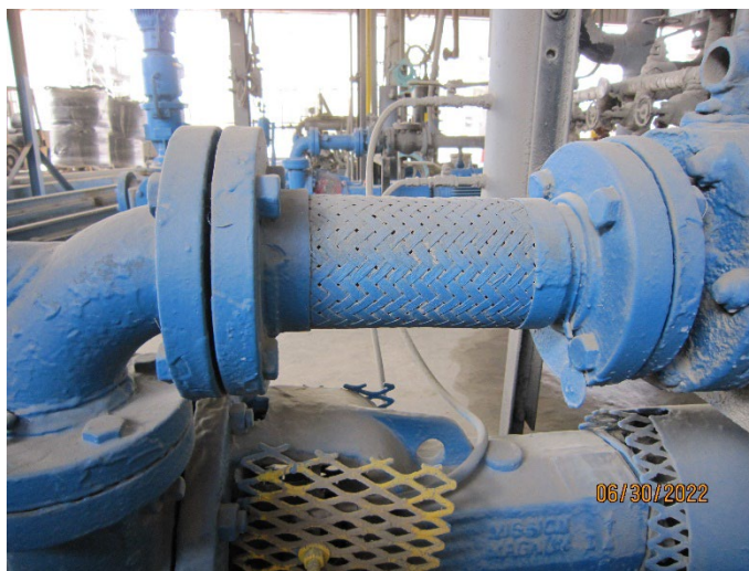
LWDF Loading Area equipment with indistinguishable tags. Photograph 2 taken at 10:34am
