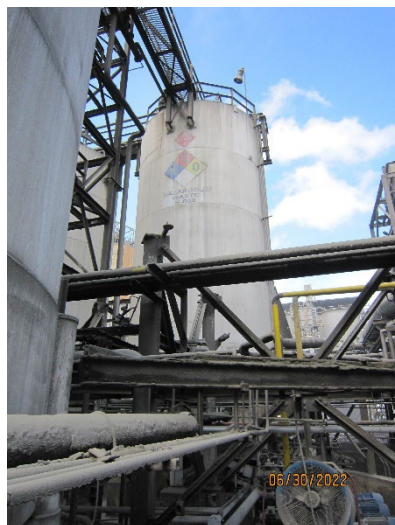
Tank Farm area hazardous waste tank labels. Photograph 22 taken at 11:02am
