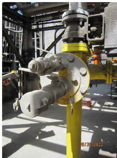
Tank Farm area with indistinguishable tags on equipment. Photograph 10 taken at 10:47am
