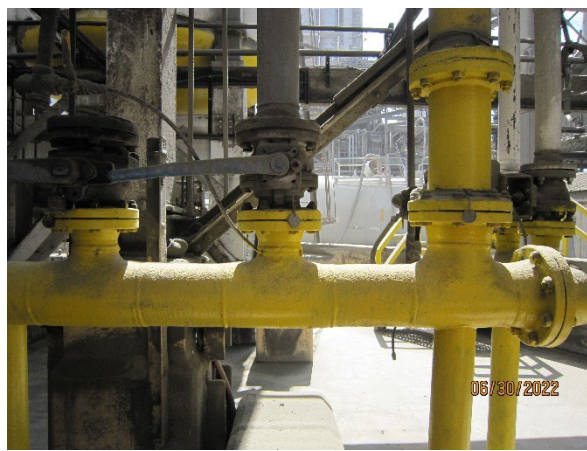
Tank Farm area with indistinguishable tags on equipment. Photograph 12 taken at 10:49am
