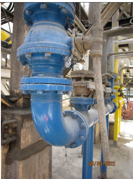
Tank Farm area with indistinguishable tags on equipment. Photograph 15 taken at 10:51am
