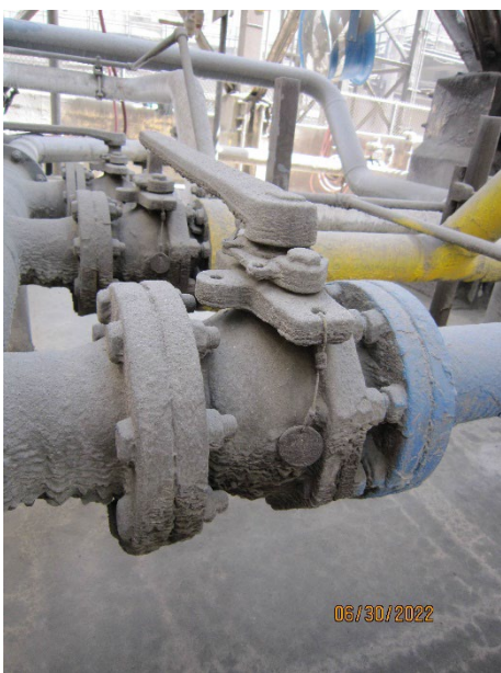
Tank Farm area with indistinguishable tags on equipment. Photograph 19 taken at 10:57am
