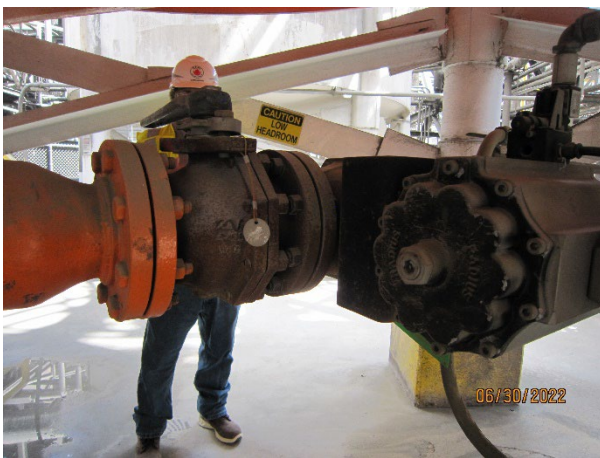
Tank Farm area with indistinguishable tags on equipment. Photograph 17 taken at 10:53am
