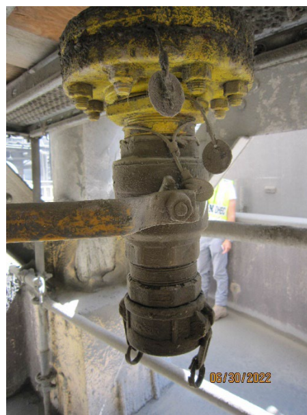
Tank Farm area with indistinguishable tags on equipment. Photograph 20 taken at 10:59am
