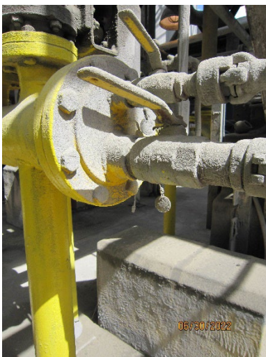
Tank Farm area with indistinguishable tags on equipment. Photograph 9 taken at 10:45am
