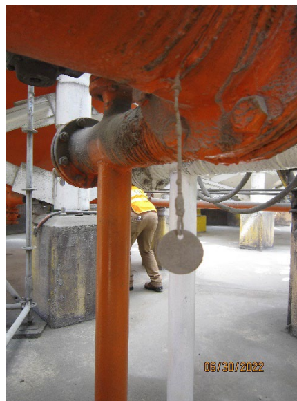
Tank Farm area with indistinguishable tags on equipment. Photograph 14 taken at 10:50am
