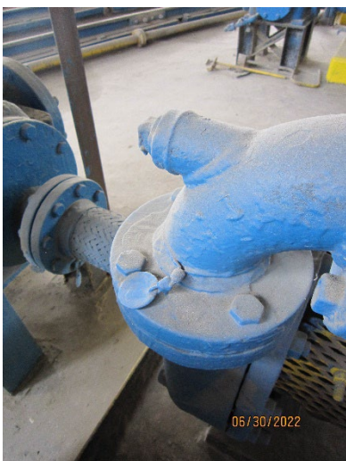
LWDF Loading Area equipment with indistinguishable tags. Photograph 1 taken at 10:34am
