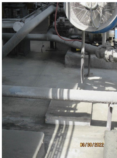
Tank Farm area with tubing connected to containers. Photograph 24 taken at 11:03am
