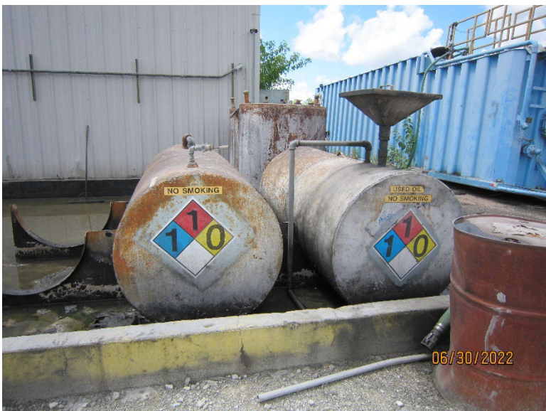
Product and Used Oil tank farm. Photograph 29 taken at 11:55am
