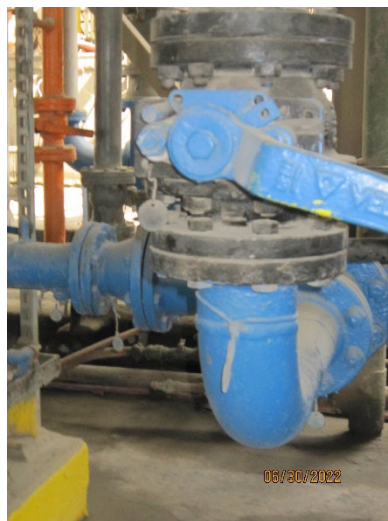
LWDF Loading Area equipment with indistinguishable tags. Photograph 6 taken at 10:39am
