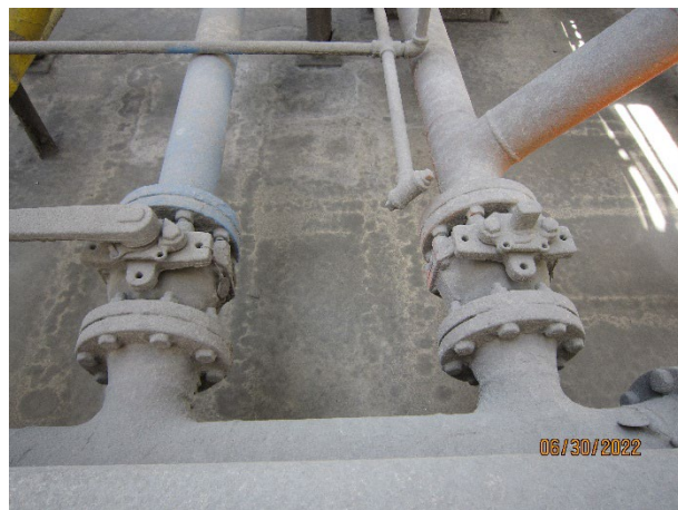
Tank Farm area with indistinguishable tags on equipment. Photograph 18 taken at 10:57am
