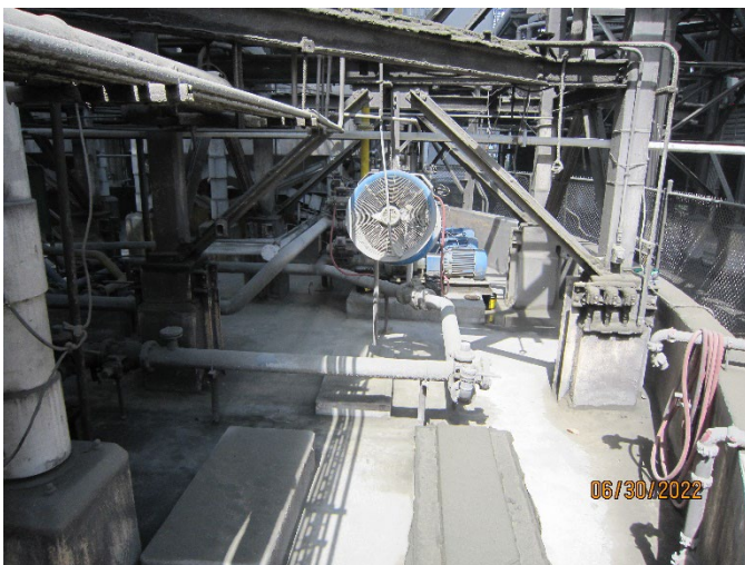
Tank Farm area with three (3) containers; two (2) with tubing and one (1) left open. Photograph 23 taken at 11:02am
