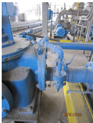
LWDF Loading Area equipment with indistinguishable tags. Photograph 4 taken at 10:35am
