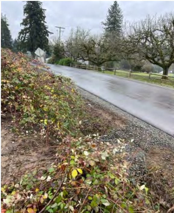
Photo 7a: Phase 3 observed break in vegetation at S. 25 th Place and low point is open to roadway.
