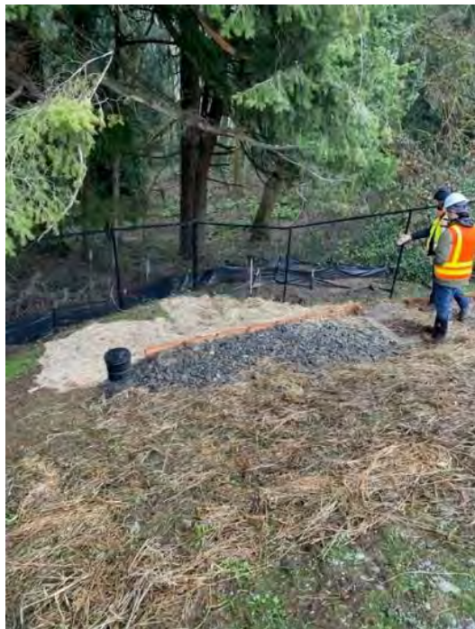
Photo 13a: Pond B silt fence needs maintenance
