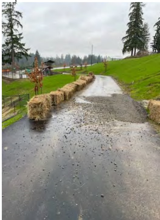
Photo 6a: Erosion observed above Pond A across paved footpath.
