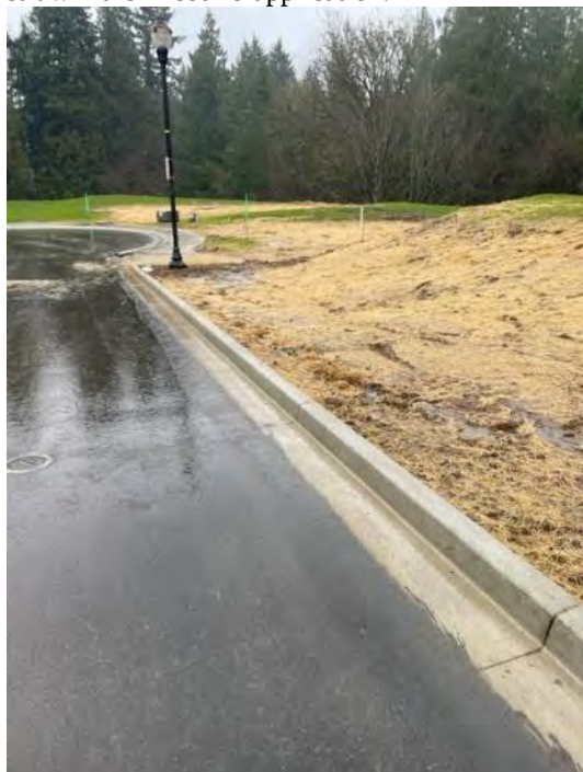
Photo 17a: Phase 2 cul-de-sac, exposed areas within straw mulch need re-application.
