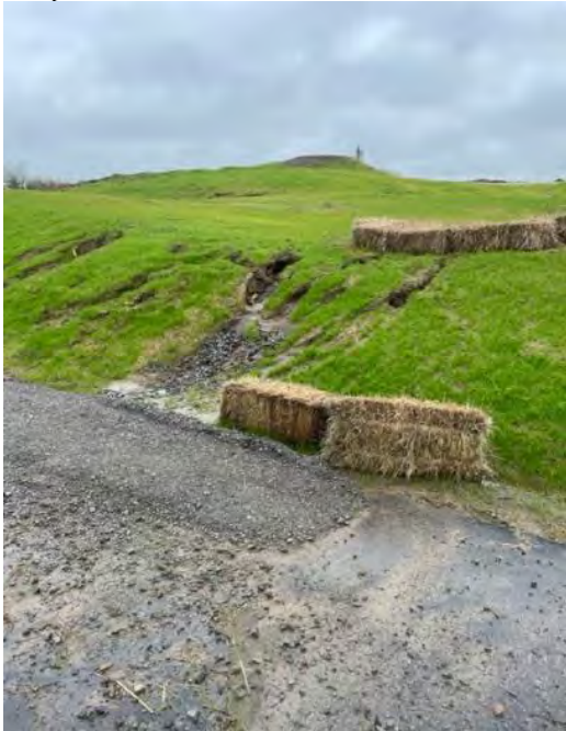
Photo 6c: Erosion observed above Pond A across paved footpath.
