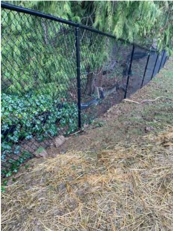
Photo 16a: Pond C silt fence needs maintenance where needed.
