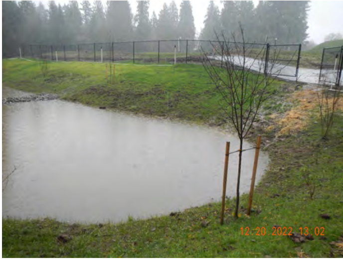
Photo #:29 (DSCN3125) Description: Facing south, photo of Pond C. Erosion observed on the southwest slope.
