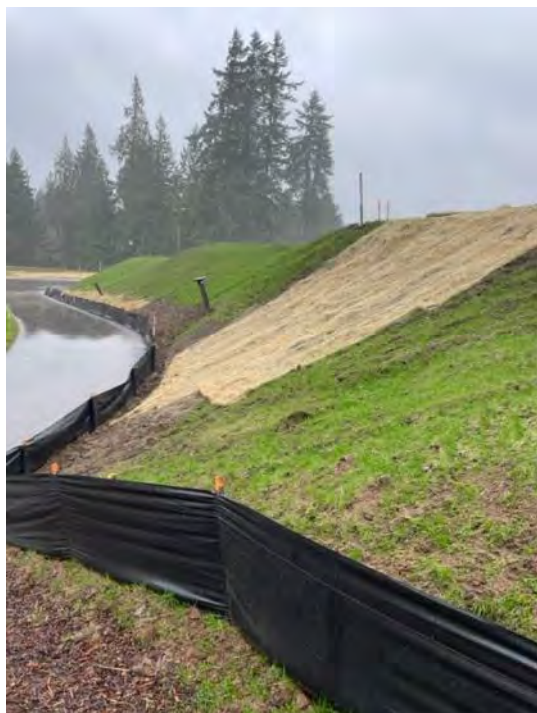
Photo 14a: North side of walking path and Pond B, silt fence needs maintenance.
