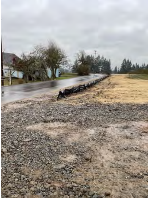
Photo 8a. West entrance to Phases 3-5 needs maintenance (Facing north).
