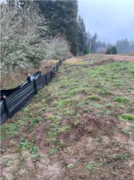
Photo 11a: Phase 5 northwest corner, silt fence needs maintenance.
