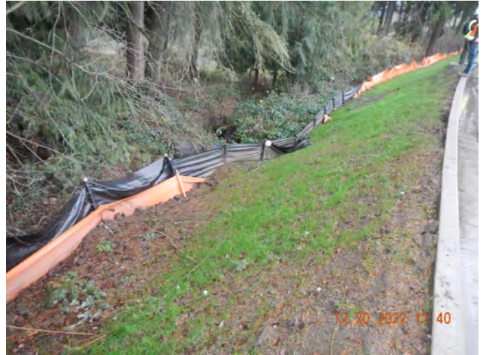
Photo #:06 (DSC3102) Description: Facing west, photo of silt fencing installed north of the Pond A discharge location, south of S. 10 th Way. A section of perimeter silt fencing was observed to have sediment deposited above one-third the height of the section of silt fence.
