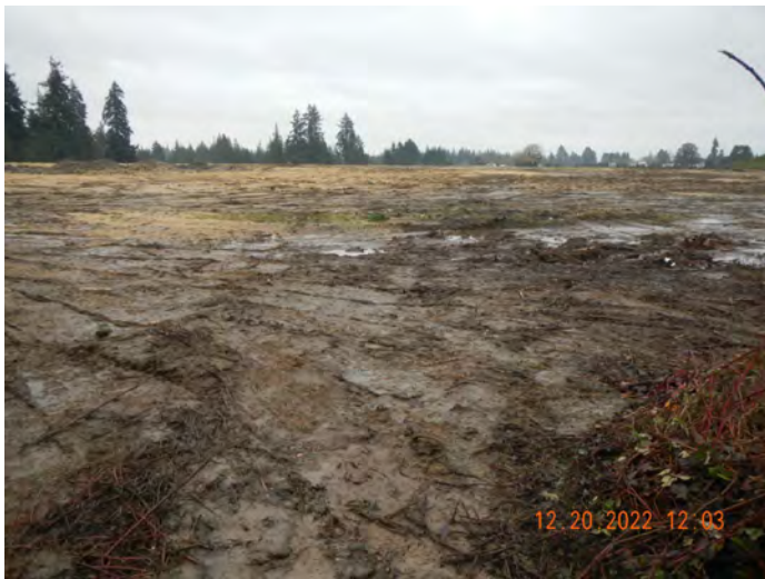
Photo #:15 (DSCN3111) Description: Facing east within Phase 3, photo of the area east of the partially cleared perimeter along S. 25 th Place. Area lacked stabilization.
