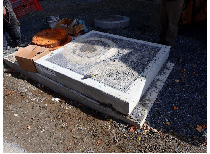
Photo #:18 Description: Photo of oil/water separator installed on 6/18/2024 (sticker on side).
