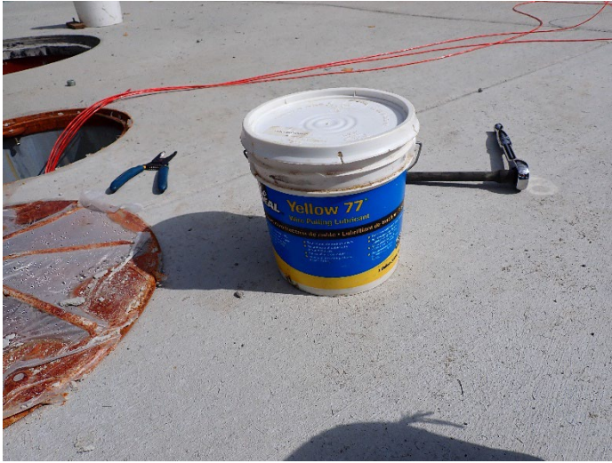
Photo #:17 Description: Photo of Yellow 77 Wire Pulling Lubricant on pavement over underground storage tanks basin.
