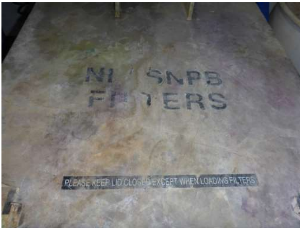
Photo 5: Lid of filter unit to drain filters from the nickel, tin and lead plating lines.
