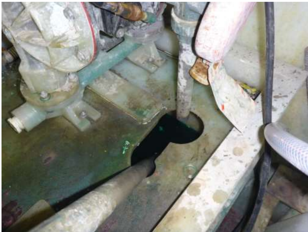
Photo 10: Hole built into the lid of the collection system and sump in the corner of the chemical storage area so that the pumping wand can be placed into the unit.
