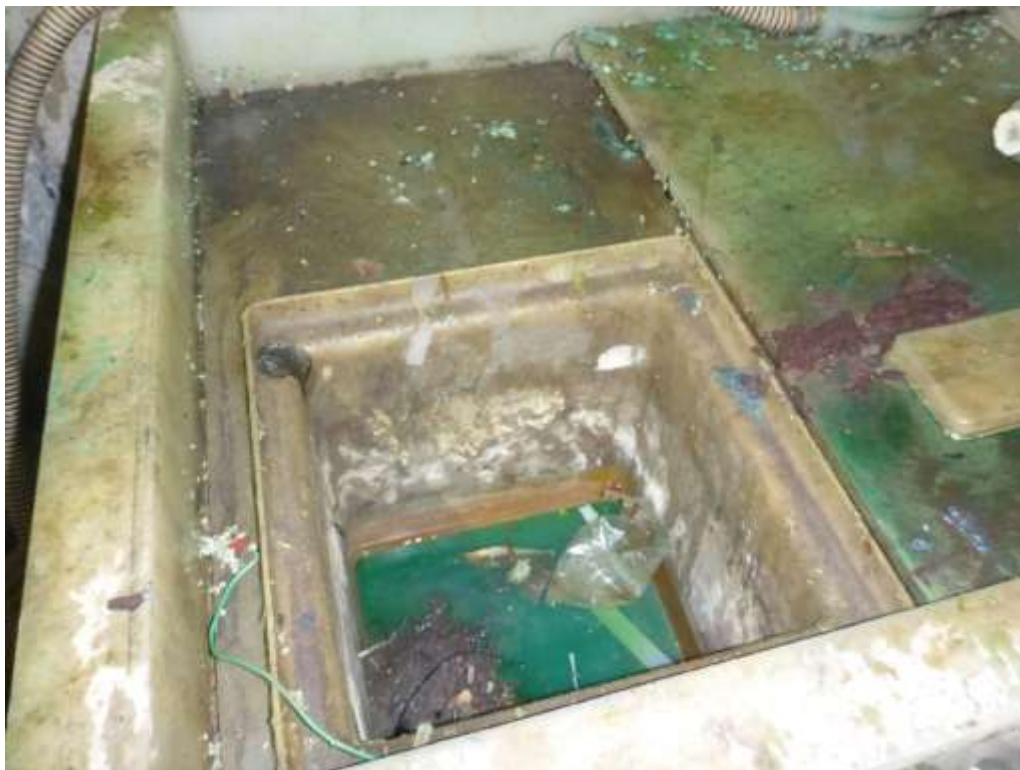
Photo 9: Strainer basin built into the lid of the collection system and sump in the corner of the chemical storage area.
