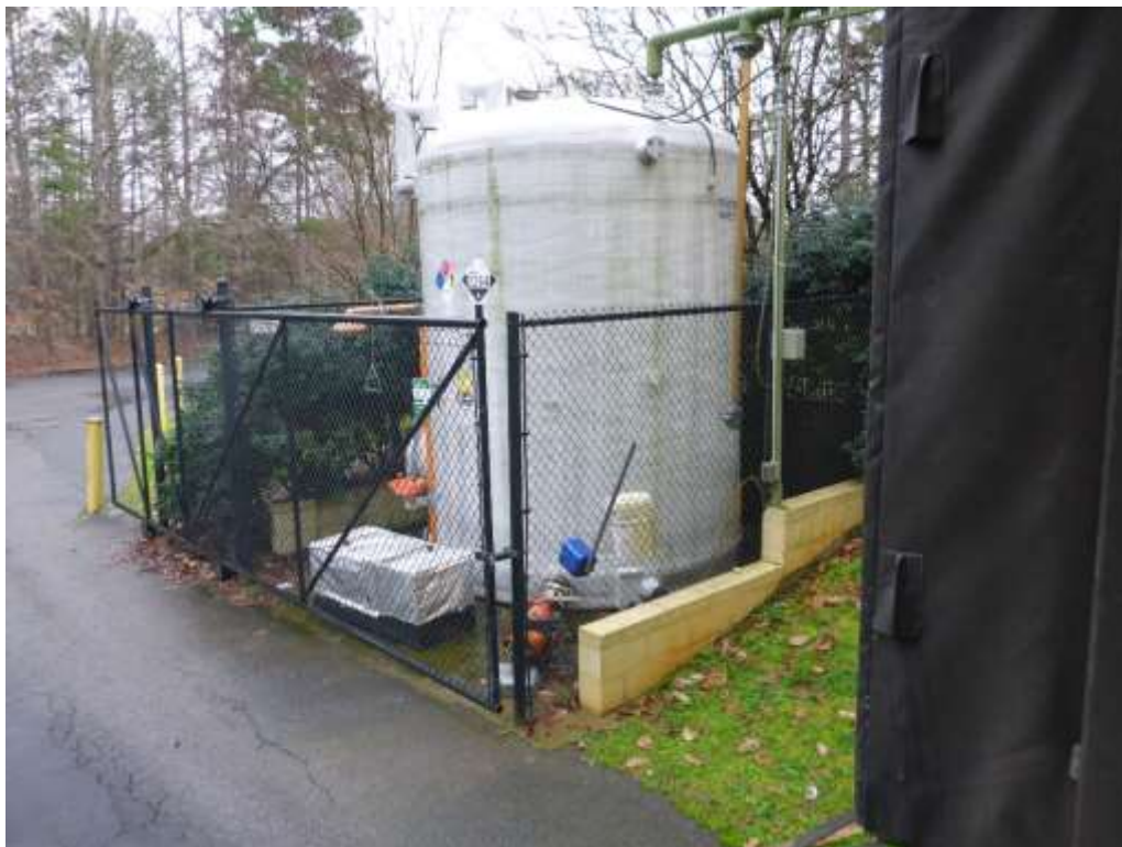
Photo 16: 5,000-gallon hazardous waste storage tank in an area just outside the bay door of the shipping and storage room.
