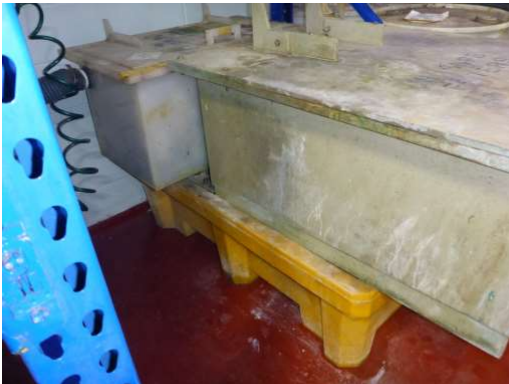
Photo 4: Two filter draining units located between the large metal shelving units in the chemical storage area.
