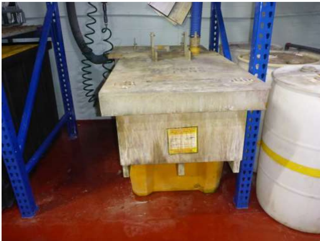
Photo 3: Two filter draining units located between the large metal shelving units in the chemical storage area.
