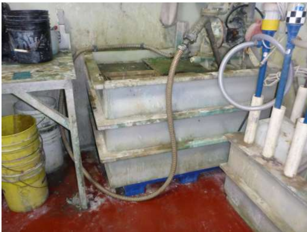
Photo 8: Collection system and sump in the corner of the chemical storage area room used to transfer liquid hazardous waste from this area into the outdoor hazardous waste storage tank.
