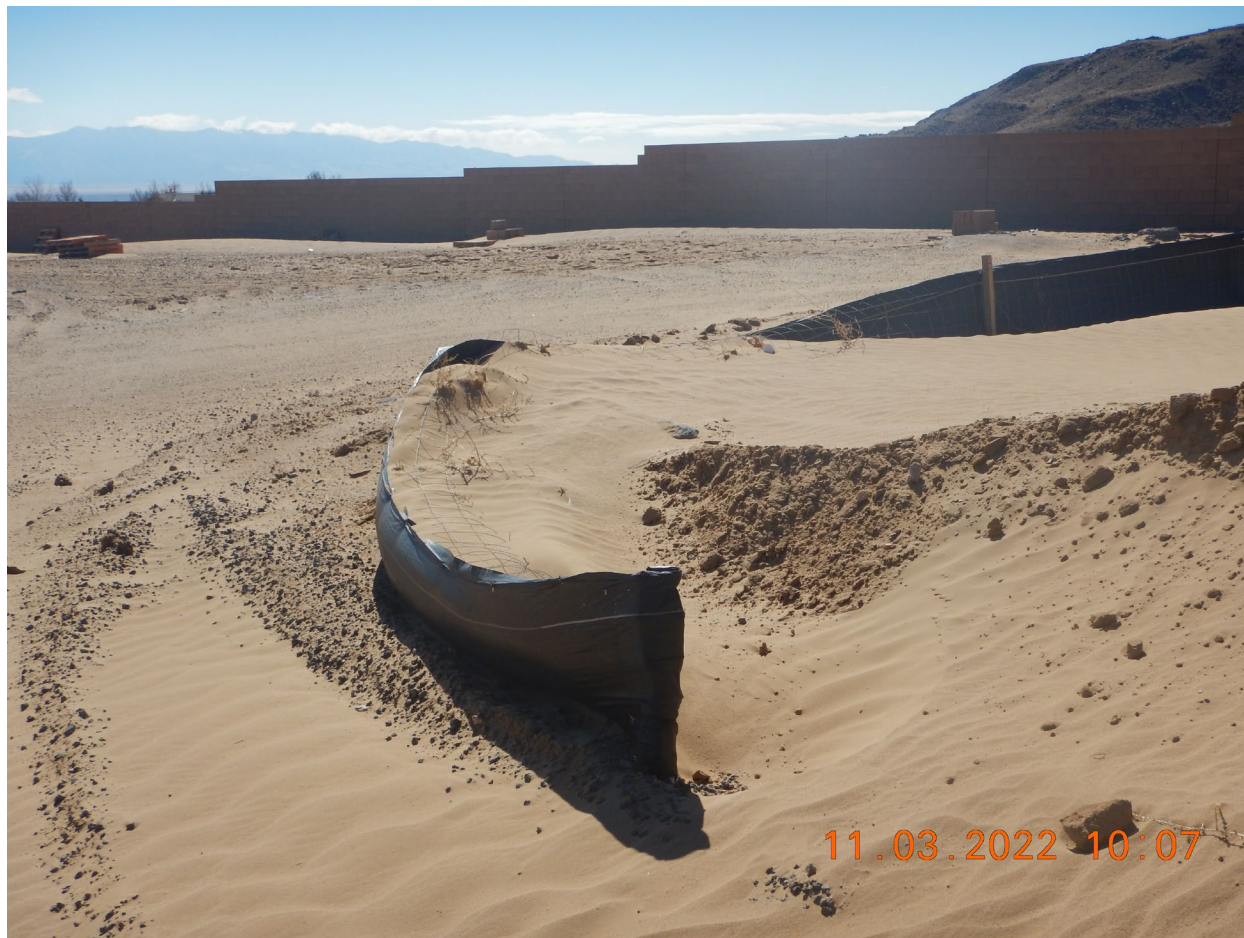
View of silt fencing in need of cleaning, repair, or replacement.(DSCN2173). Photographed by D. Esparza
