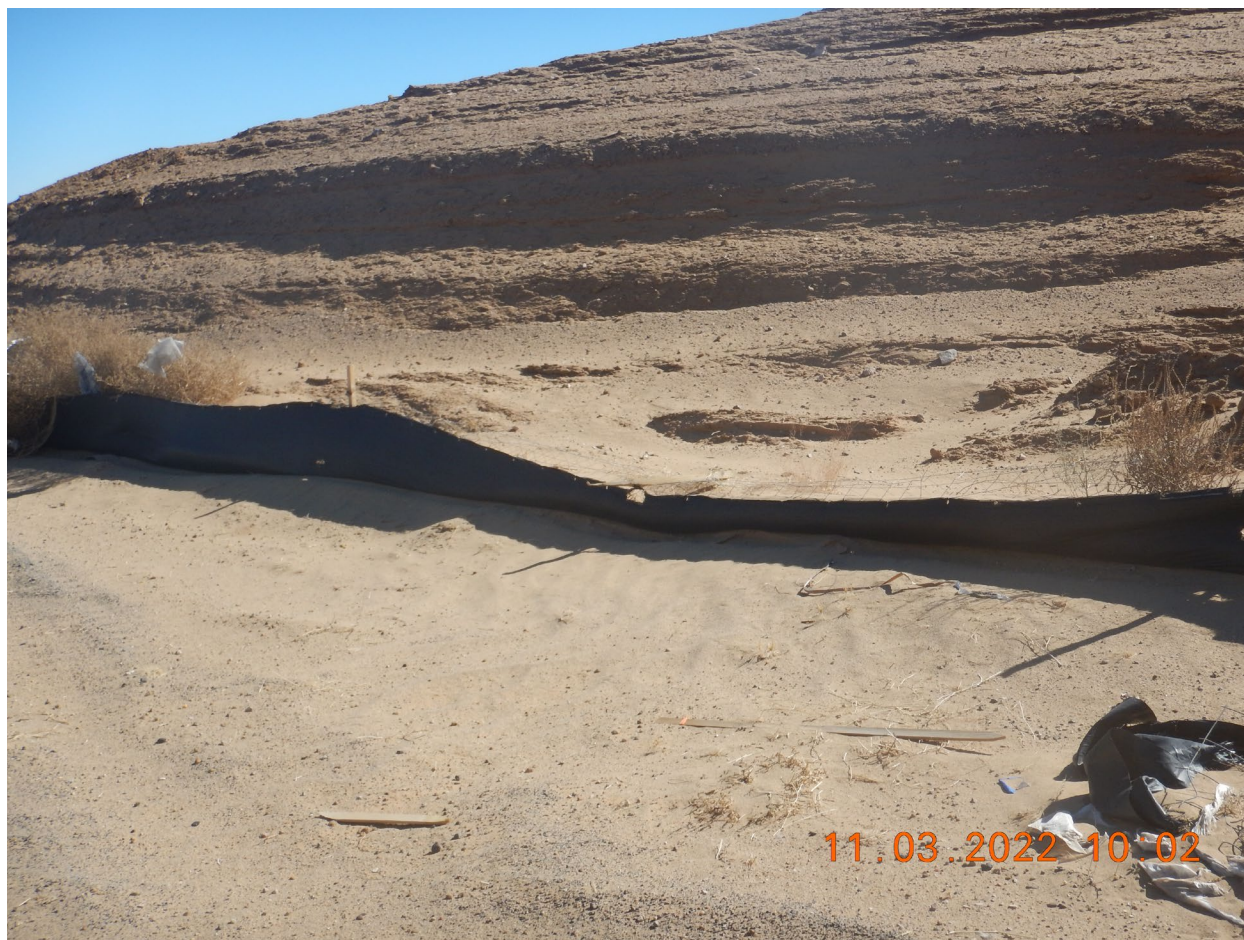
View of silt fencing in need of cleaning, repair, or replacement.(DSCN2166). Photographed by D. Esparza
