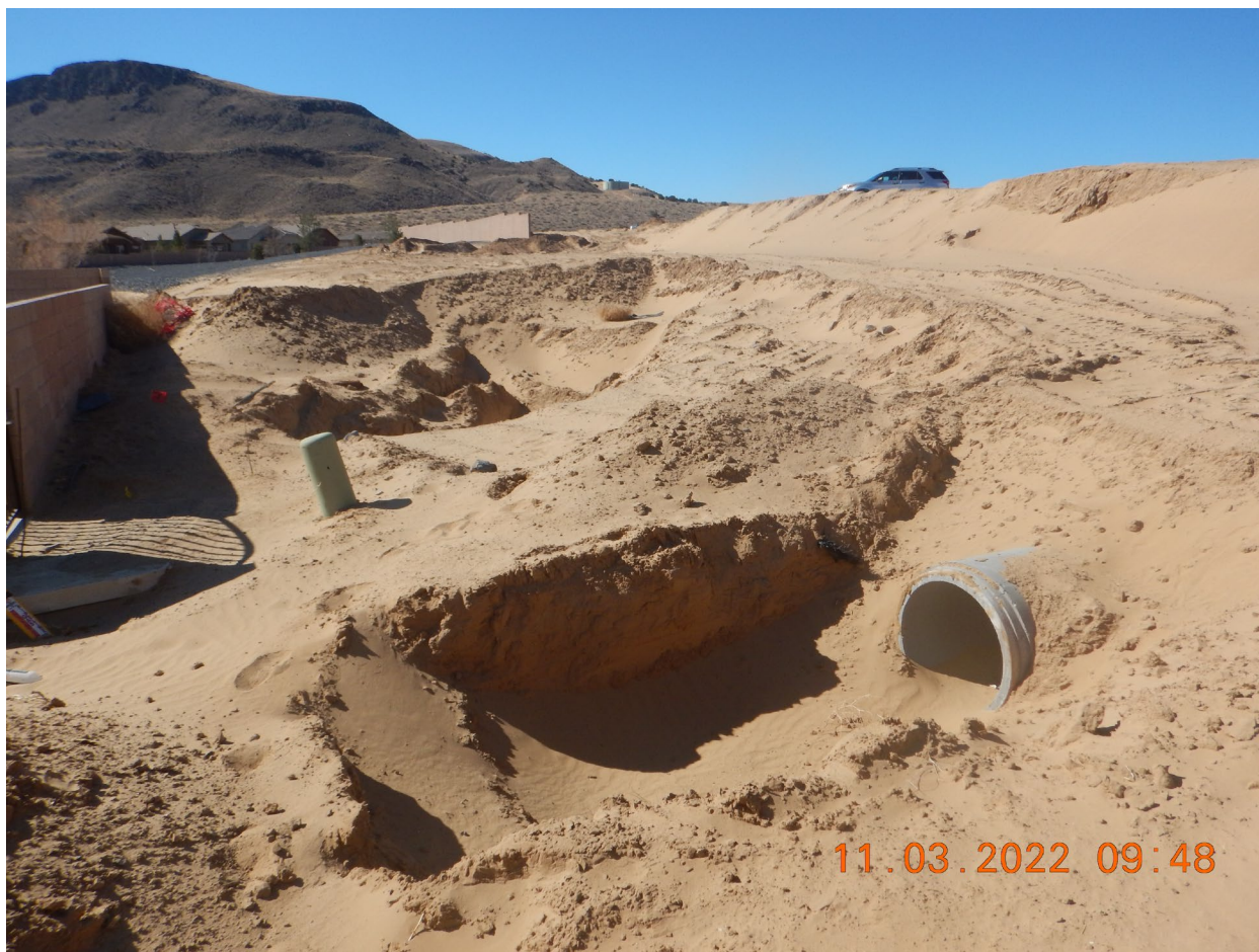
View of unstabilized excavation and embankment located along eastern side of development. (DSCN2153). Photographed by D. Esparza
