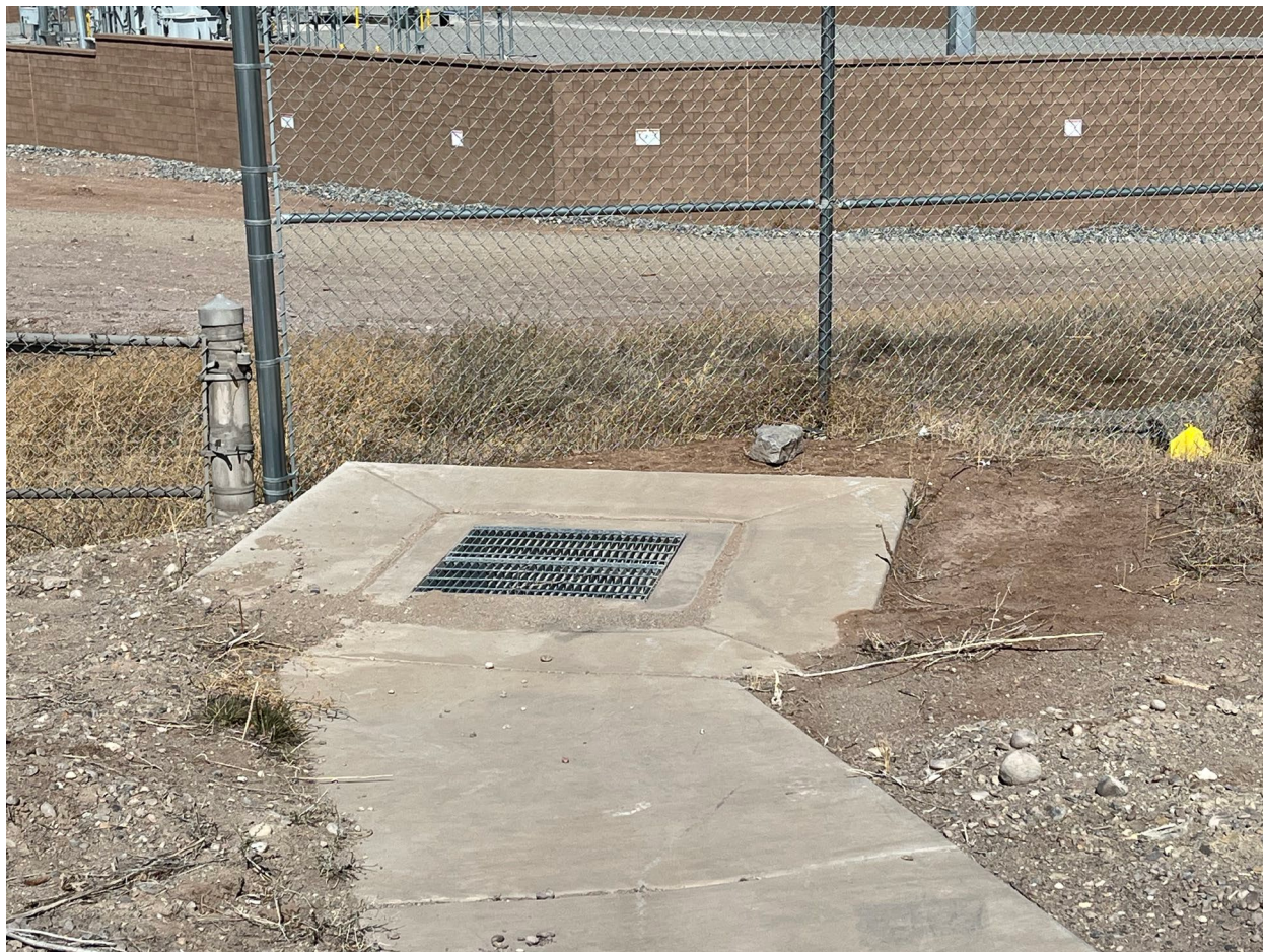
View of drop drain located at Outfall 002. (IMG_0280). (Photographed 03/12/2025: 12:01 PM) Photographed by D. Esparza.
