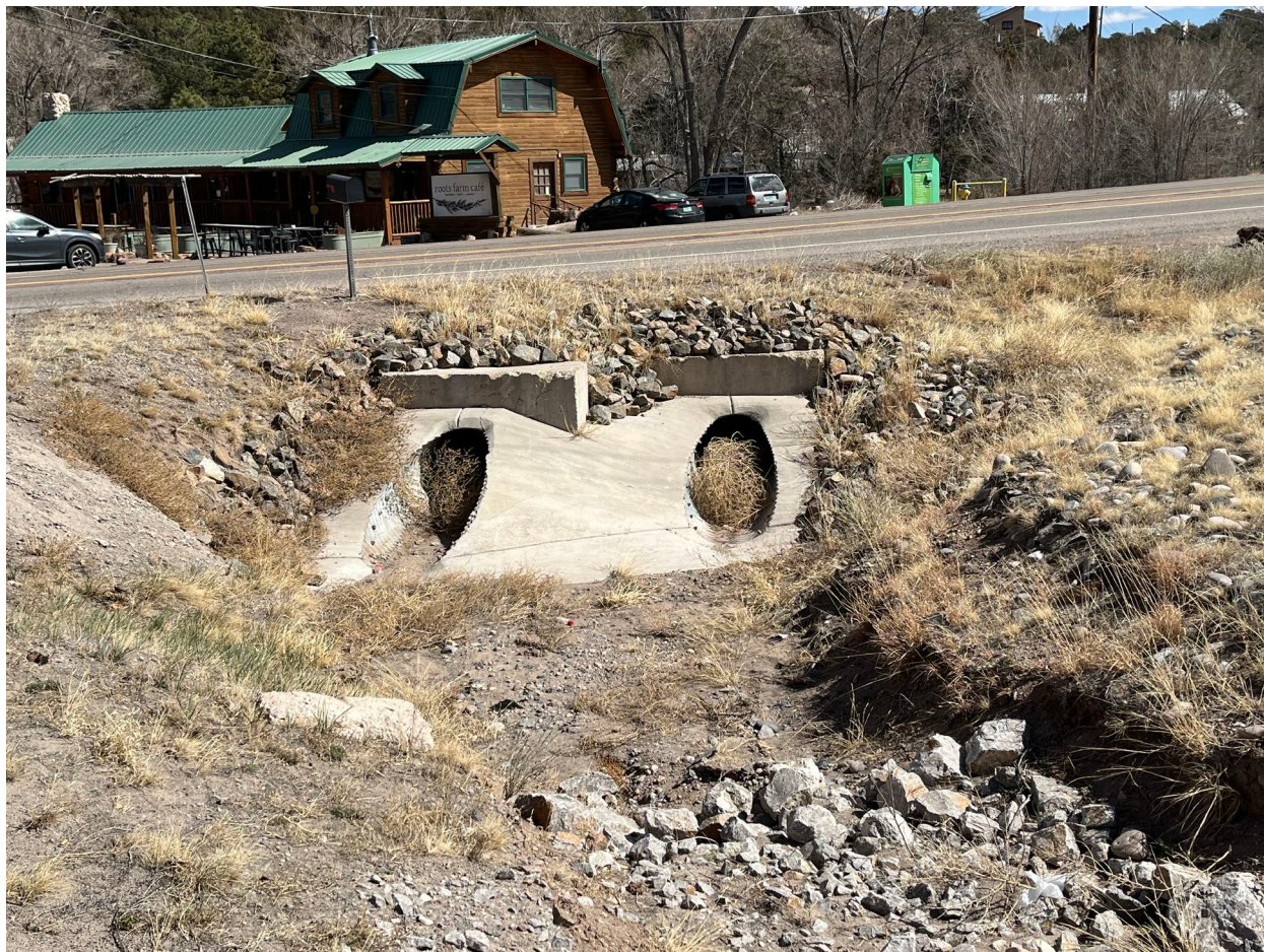
View of the obstructed culverts at the entrance to Outfall 003 adjacent to State Highway 337 looking approximately Southeast. (IMG_0282). (Photographed 03/12/2025: 12:02 PM) Photographed by D. Esparza
