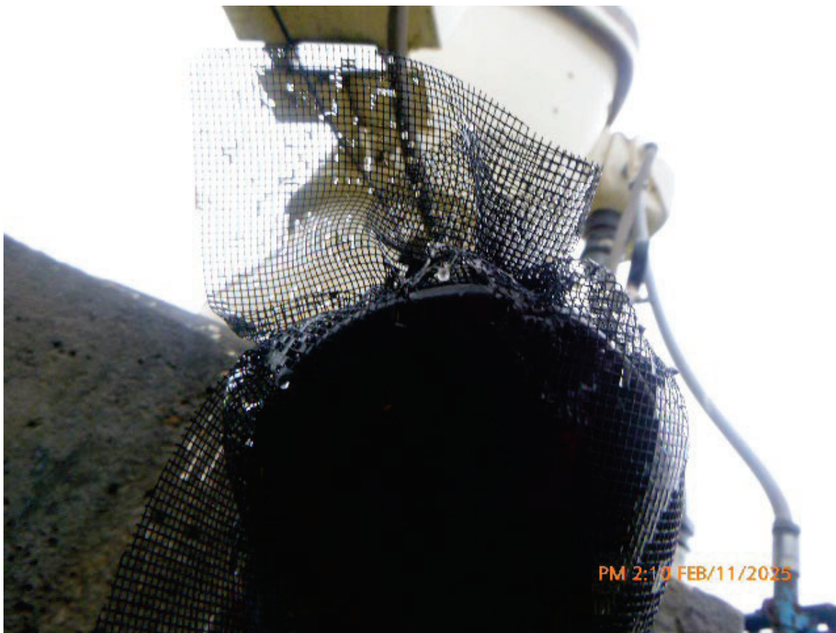
Photograph 8. 02/11/2025 2:10 PM P1010187.JPG Description: Plant 2. Torn screen on Well #2 sounding tube.
