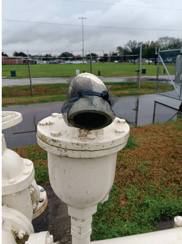
Screen on air release valve at Well #2. This photograph addresses Observation 6.
