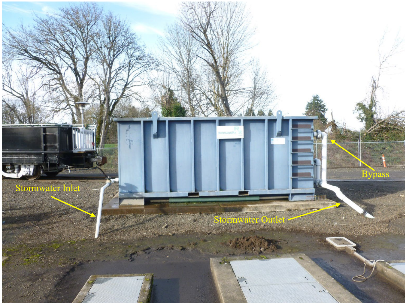
Photo 18 / P1010144 – stormwaterRx™ Filtration Unit
