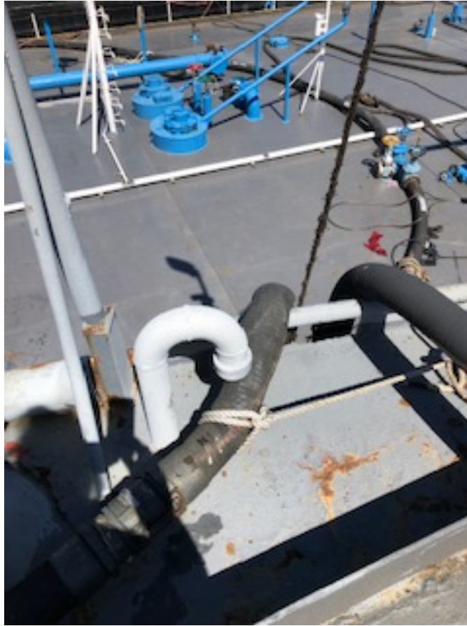
Photo 1: SPDES Discharge Hose – To Newark Bay
