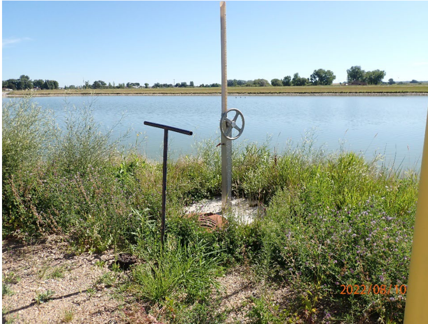
6: P8100030 Description: Discharge Valve and Outfall Location: Waubun WWTF Camera Direction: E Date/Time: August 10, 2022
