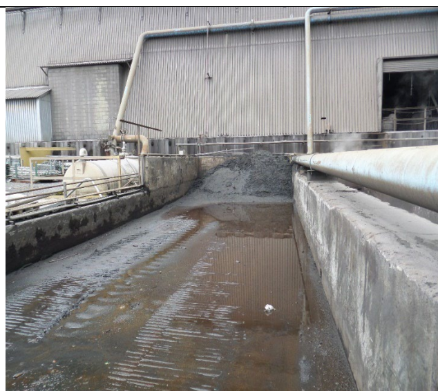
Caster Dirty Water Settling Basin. Observed a pile of cast scale. Photograph 8 taken at 11:40 a.m.
