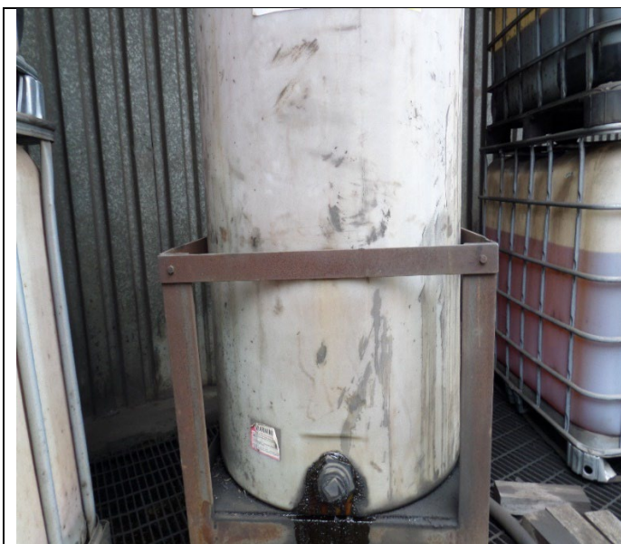
Cold Finishing Building - Used Oil Storage. Observed used oil on the bottom of 100-gallon container, the stand and around the valve. Photograph 17 taken at 1:45 p.m.
