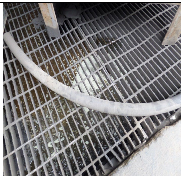
Cold Finishing Building - Used Oil Storage. Observed used oil in containment sump and on the grated platform under 100-gallon container. Photograph 18 taken at 1:45 p.m.
