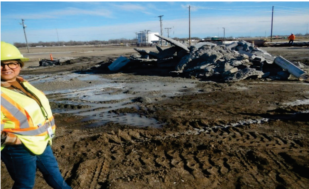
Photo 22, Illegal concrete washout practices at the Wichita Industrial District.
