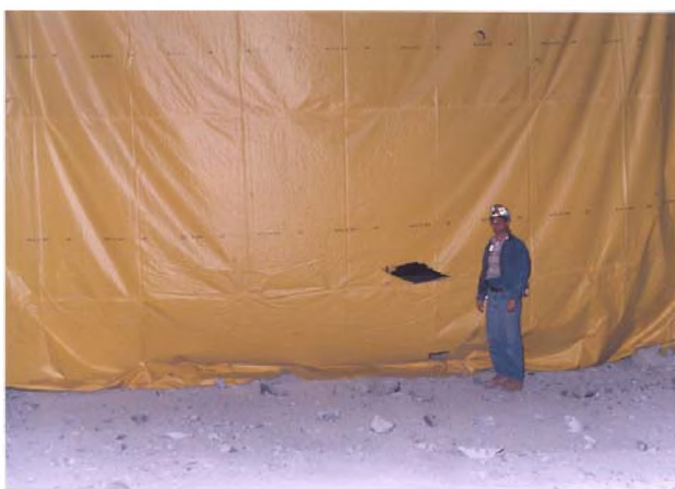
Figure 6. Fly rock damage in brattice cloth.
